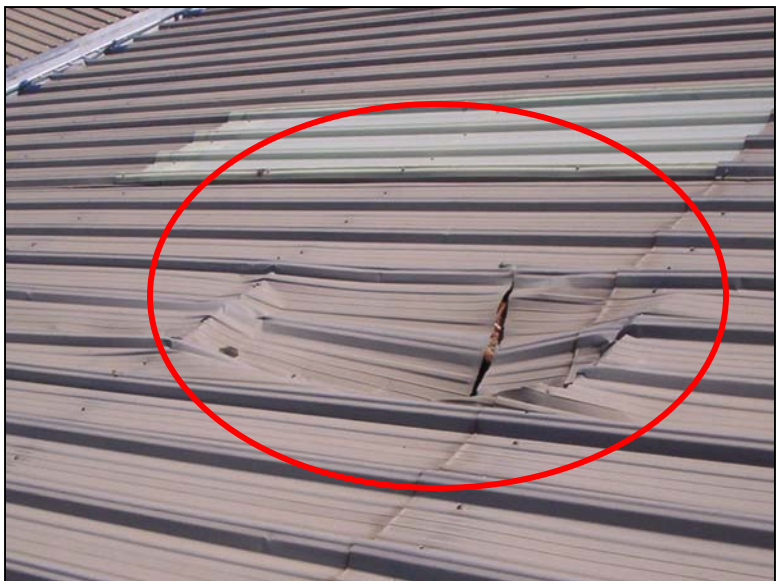
3. Damage to roof from flying debris.
