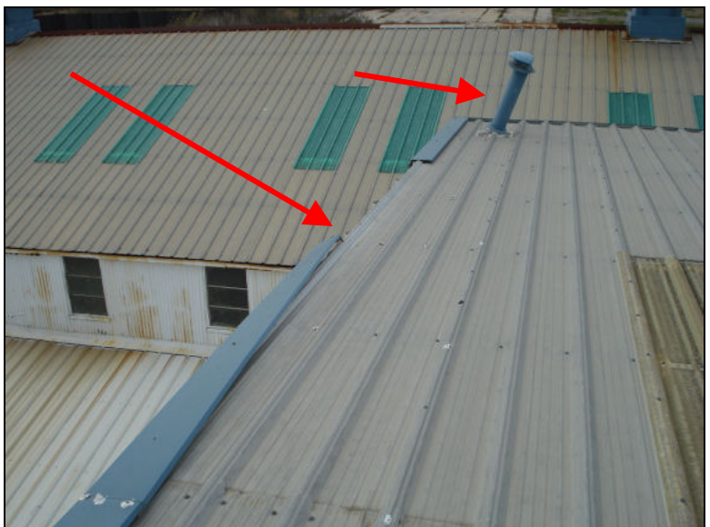
9. Missing rake trim also vent is damaged.
