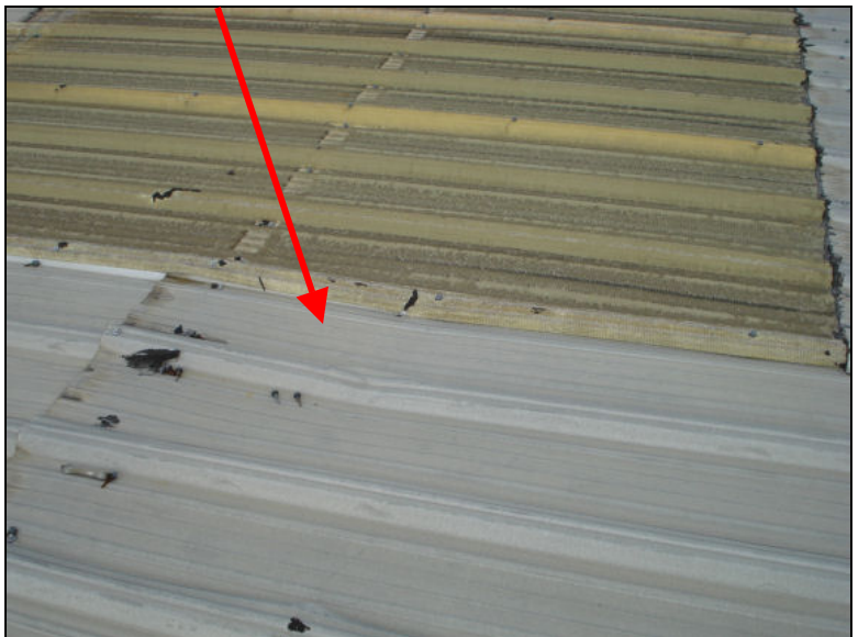
8. Buckled from flying debris.
