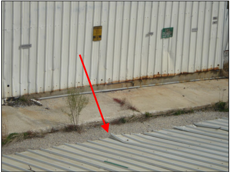
10. Damaged by flying debris.
