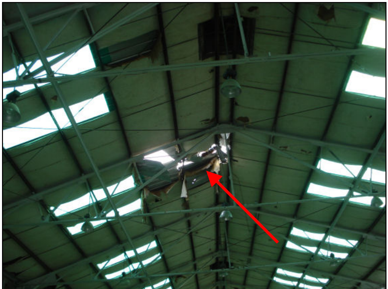
12. Roof panel and insulation damaged from flying debris.
