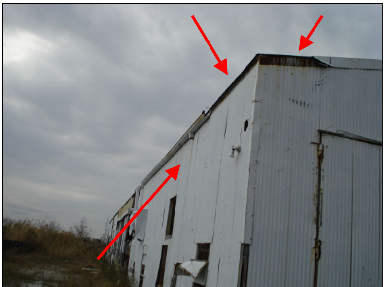
15. Missing eave and rake trim also down spout.
