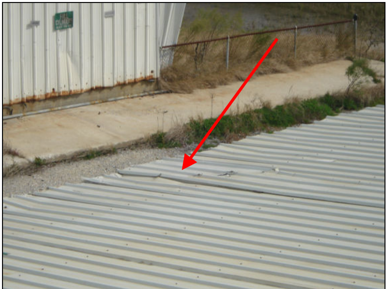
9. Damaged by flying debris.
