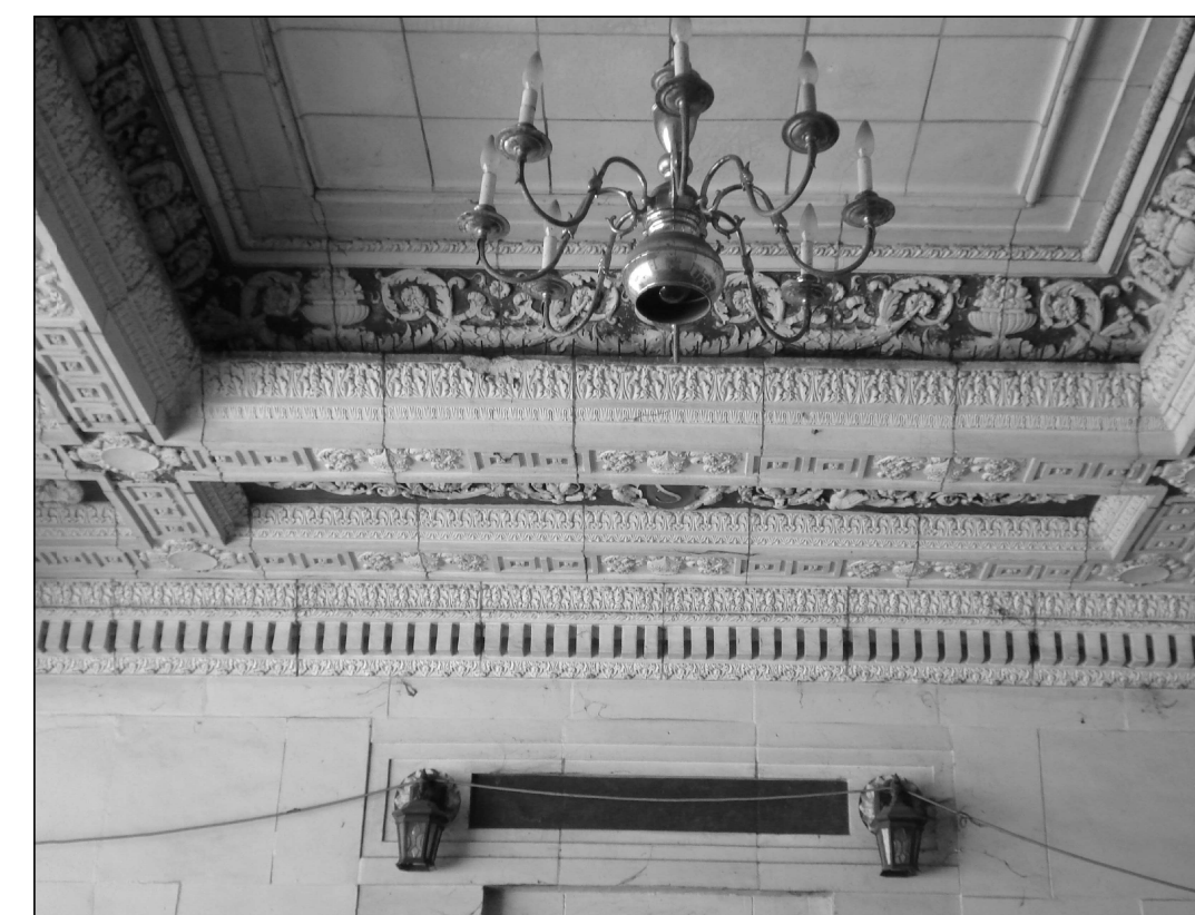
G PHOTO DSC01961 DECORATIVE DETAILS ALONG SIDE CORNICE - NOTE CHIPPED EDGE LEFT OF CENTER
