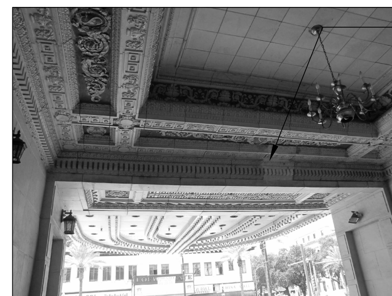
E PHOTO 1435 ENTRANCE CEILING FACING CANAL STREET; REPLACE FIBERGLAS WITH NEW TERRA COTTA TO MATCH EXISTING IN DETAILING, AND FINISH
