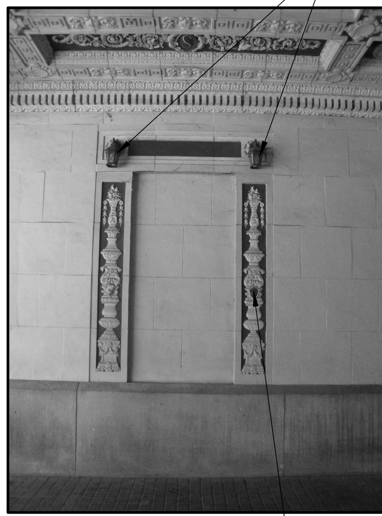
649 ALCOVE REMOVE ALL PAINT AND RESTORE DETAILS TO ORIGINAL CONDITION REPAIR TO MATCH EXISTING
