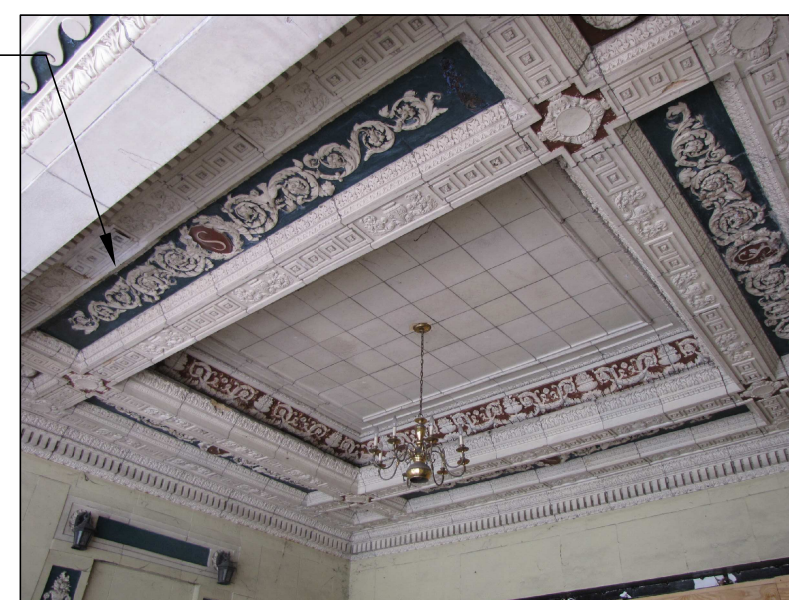
D PHOTO 1434 ENTRANCE CEILING FACING INTO ENTRANCE; REMOVE PAINT AND REPAIR ALL CHIPS, CRACKS AND BROKEN PIECES.
