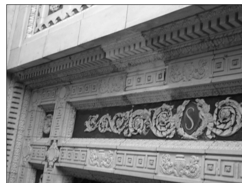
C PHOTO DSC01963 FIBERGLASS REPLACEMENT PIECE IN ENTRANCE CEILING
