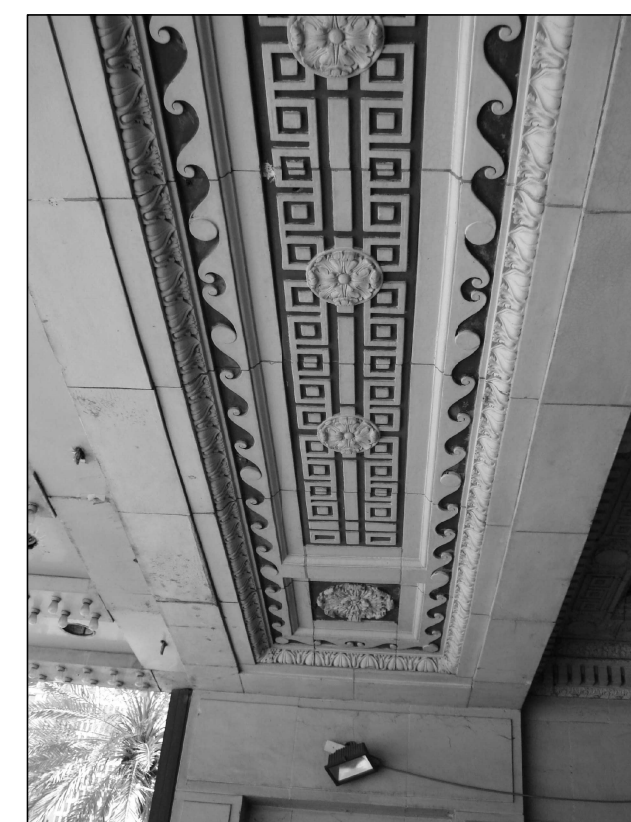
F PHOTO DSC01971 DECORATIVE BAND ACROSS ENTRANCE BEAM; INSPECT STAINED TERRA COTTA FOR CONDITION OF HANGERS, REPAIR AND REPLACE AS NECESSARY
