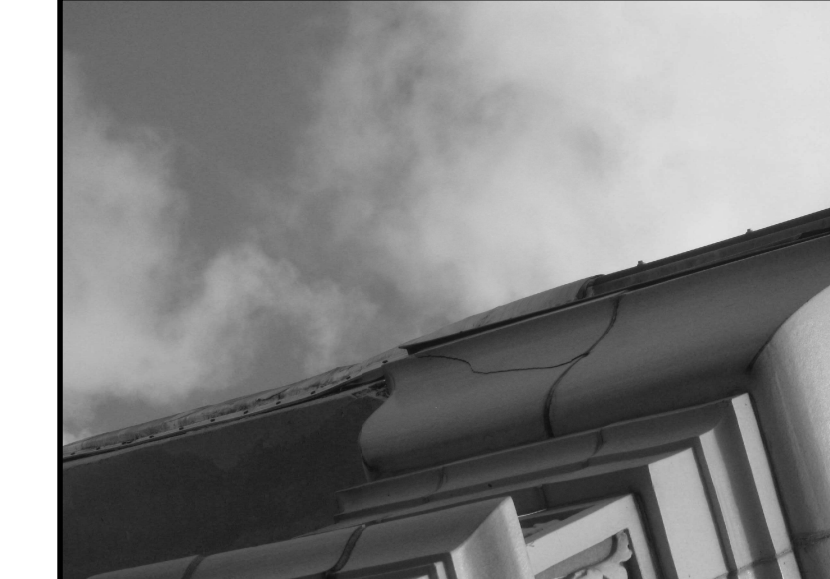
K PHOTO 1851 CRACKS IN CORNICE AT SOUTHERN CORNER OF RAMPART ST. FACADE - CHECK HANGERS, REPAIR AND REPLACE AS NECESSARY
