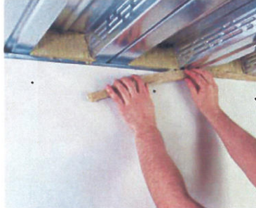
The deflection gag is filled with mineral wool.
