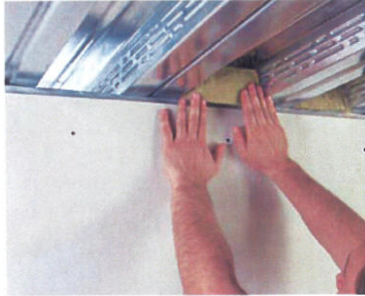
Mineral wool is placed in the fluted metal deck after the drywall is installed
