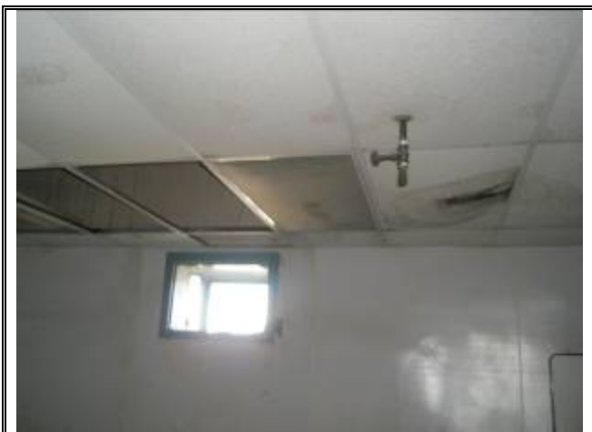
Photograph No. 051: inside compressor room of bldg 4
