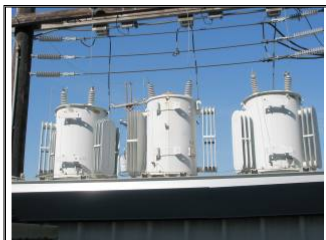
Photograph No. 078: transformers
