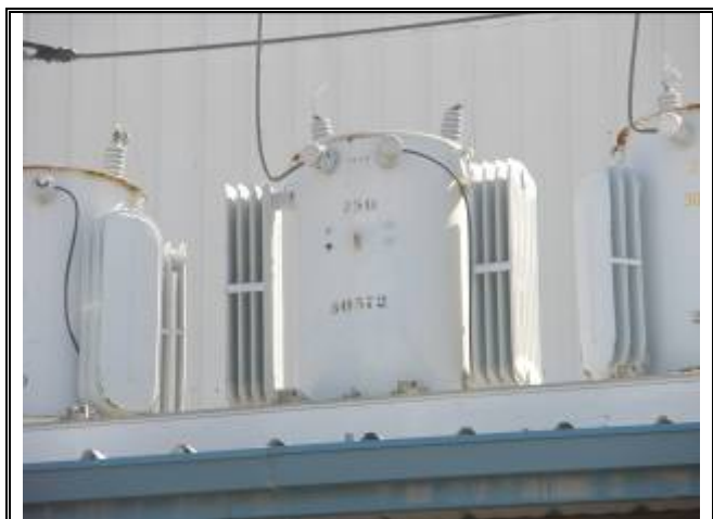
Photograph No. 080: transformers
