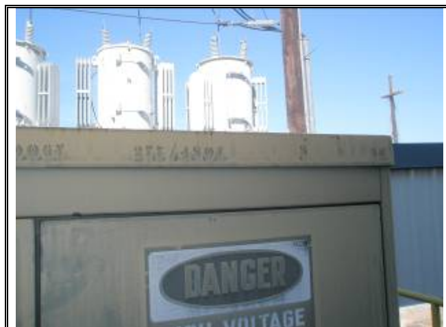
Photograph No. 077: transformers
