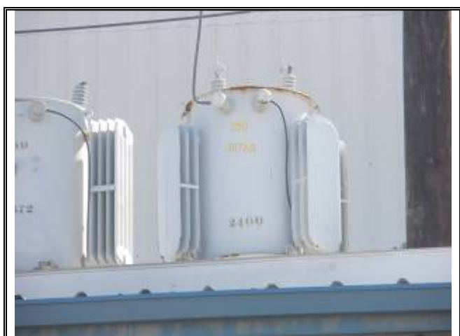
Photograph No. 081: transformers
