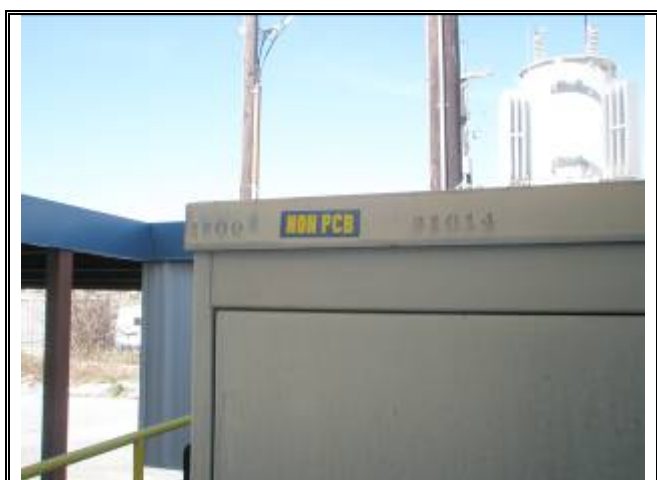
Photograph No. 075: transformers
