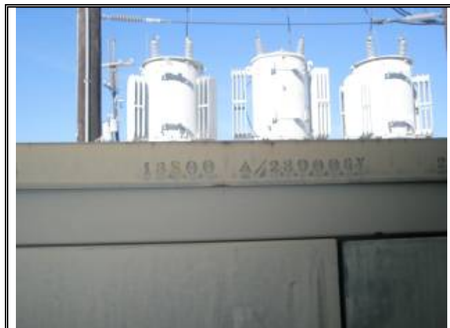
Photograph No. 076: transformers
