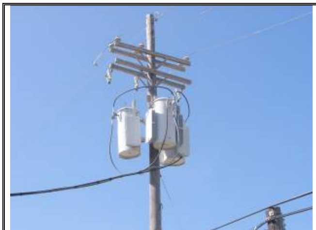
Photograph No. 082: transformers
