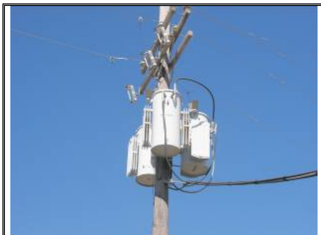
Photograph No. 083: transformers
