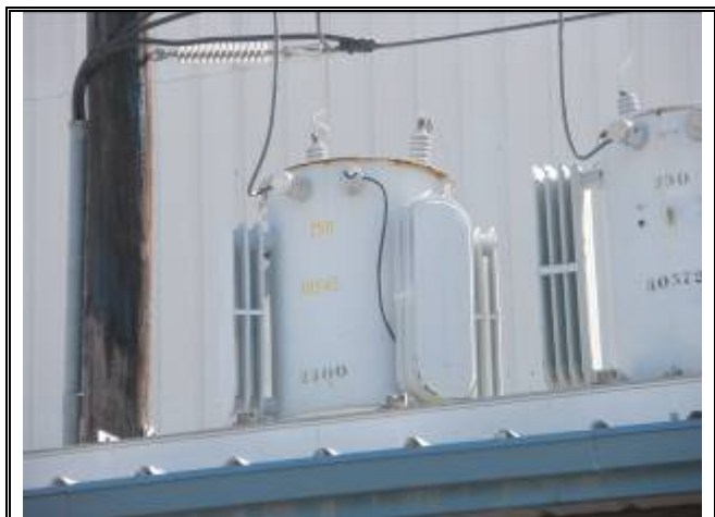
Photograph No. 079: transformers
