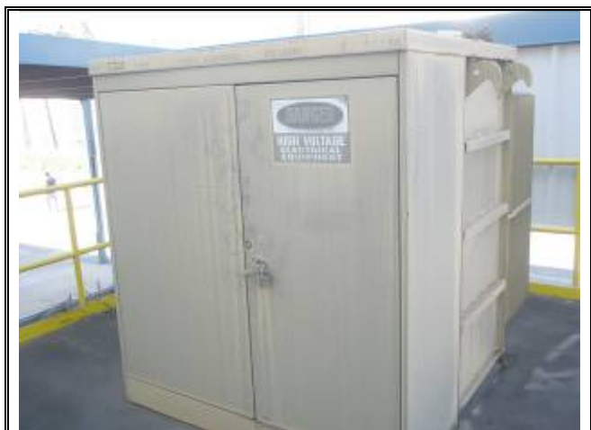
Photograph No. 074: transformers
