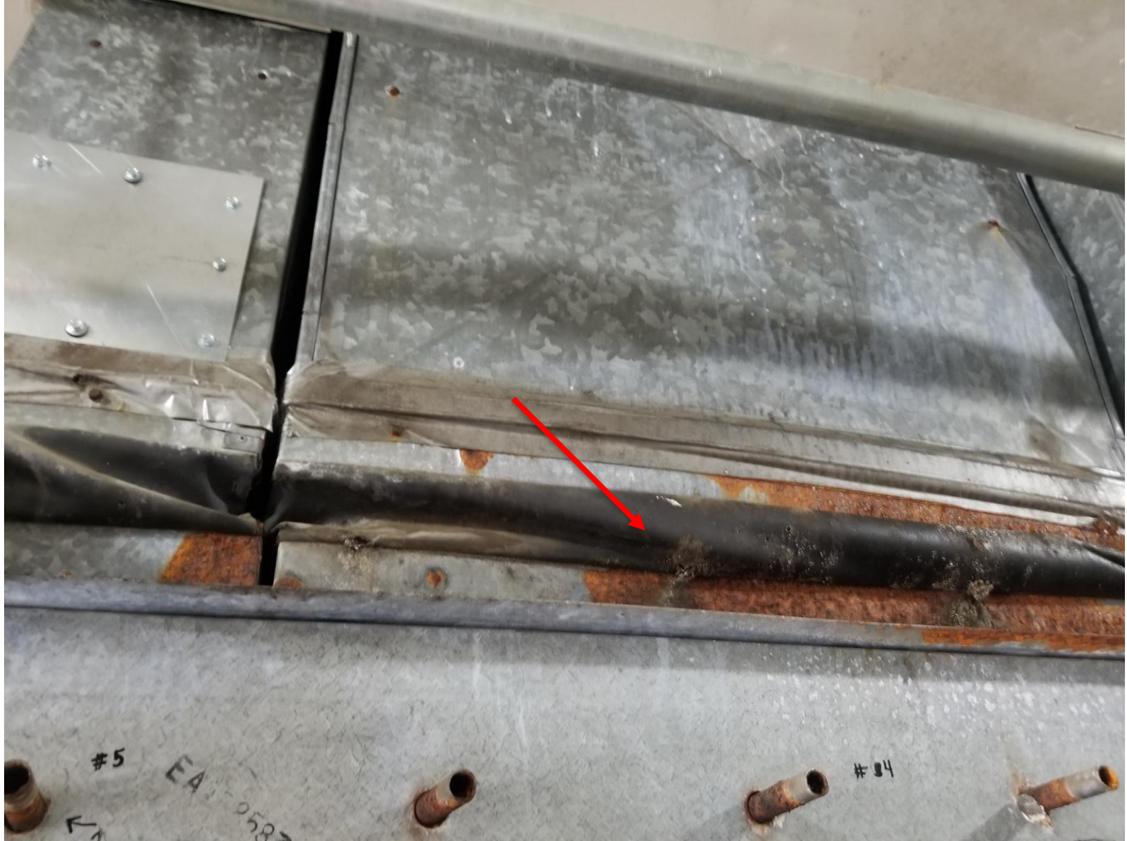
View of HA-03: Black HVAC vibration dampener.
