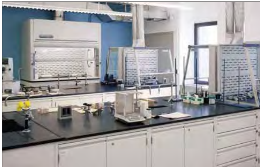
A Protector XStream Laboratory Hood is installed along the wall. Protector XVS Ventilation Stations are mounted back-to-back on islands of casework.
