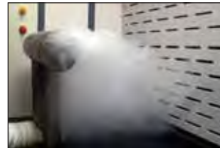
Smoke released inside the hood moves in a horizontal stream to the primary baffle slots.
