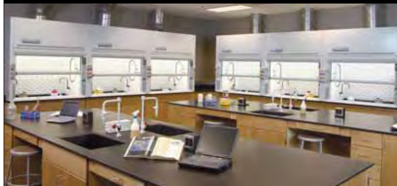
Protector XStream Laboratory Hoods line the walls in this laboratory at Gwinett University Center, Lawrenceville, Georgia.
