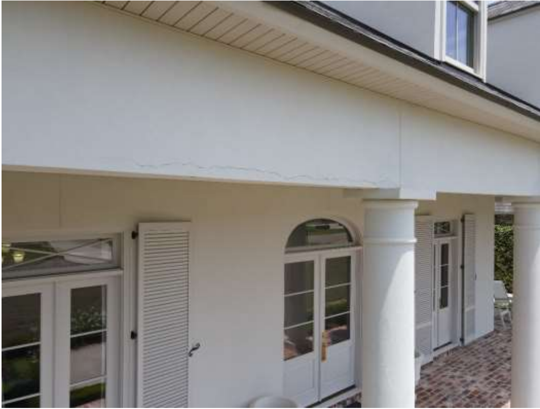
Photograph #1 – View of the horizontal crack in the stucco-finished wall.
