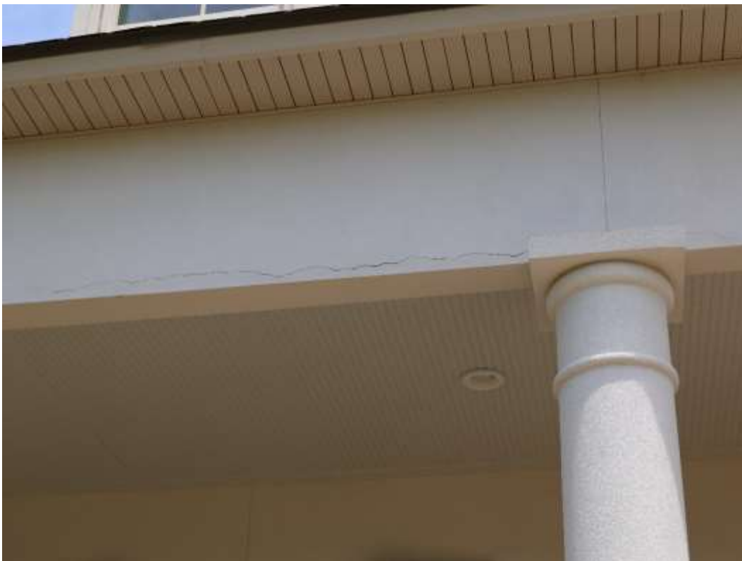
Photograph #2 – View of the horizontal crack in the stucco-finished wall.
