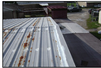
DAMAGED ROOF END RAKE N.T.S. J A1|A2
