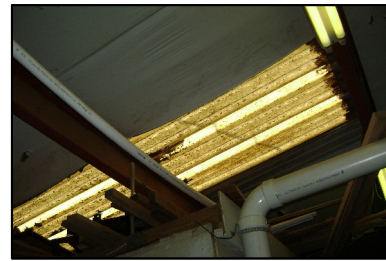
DAMAGED INTERIOR CEILING/ROOF N.T.S. K A1|A2
