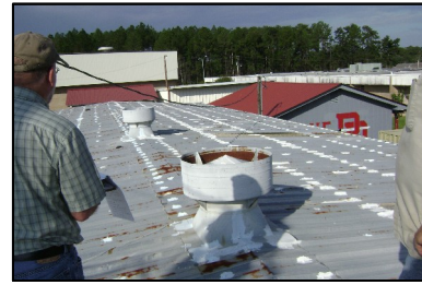
DAMAGED ROOF AND VENTILATORS N.T.S. B A1|A2
