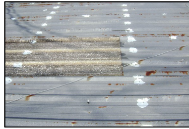
DAMAGED FIBERGLASS ROOF PANELS N.T.S. C A1|A2
