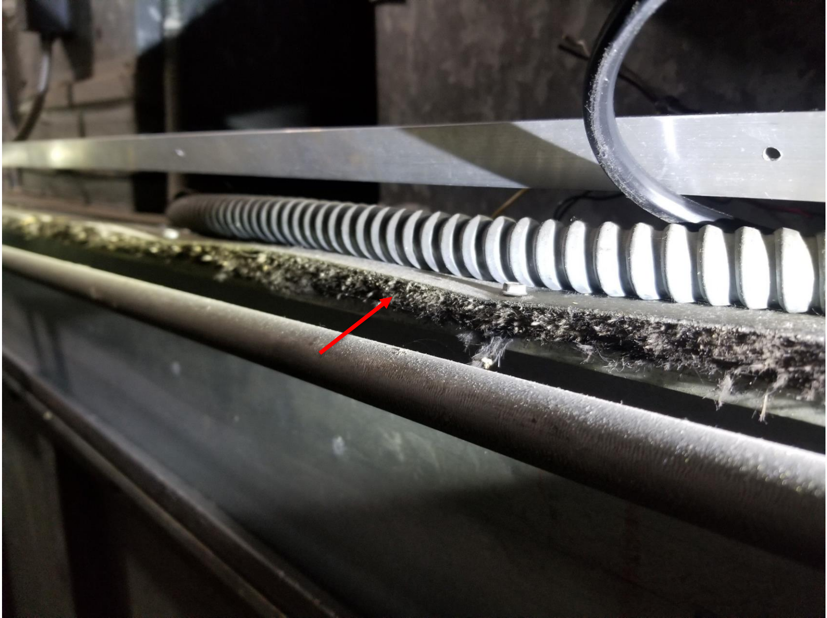
View of HA-04: Black/gray HVAC air handler jacket.
