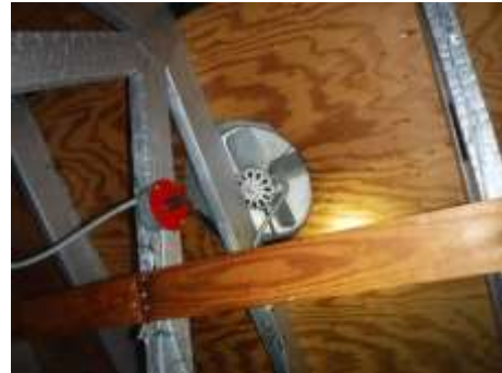
Figure 44 Power fan does not operate.
