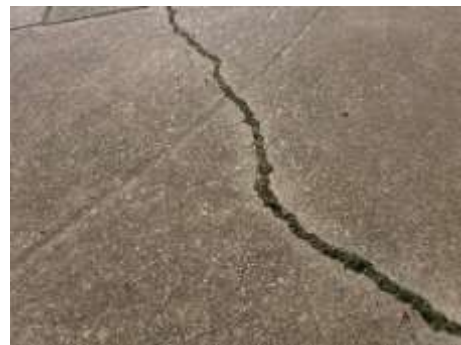
Figure 18 Seal the cracks to prevent a trip hazard.
