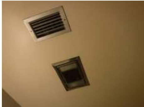
Figure 55 Bath fans run poorly; second floor.
