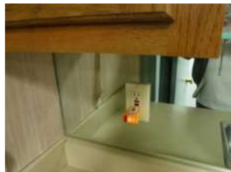
Figure 54 The GFCI by the bar sink to the left does not operate.
