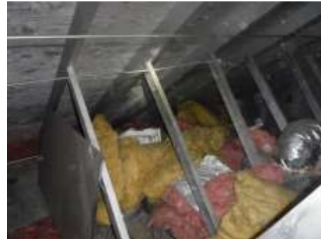
Figure 50 Insulation is displaced.
