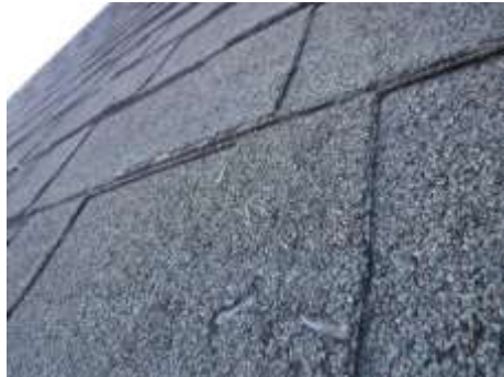
Figure 13 Same as 12; possible hail damage.
