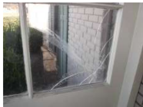
Figure 30 Cracked glass needs repairs.
