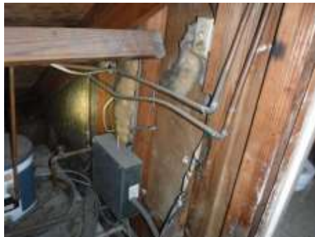
Figure 35 Replace all missing insulation.
