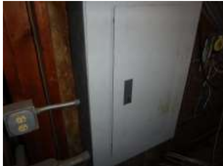
Figure 37 The lock does not operate.
