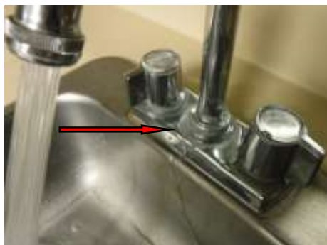
Figure 53 Bar sink leaks at the nut.
