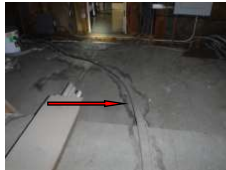
Figure 36 Refrigerant lines dripping.
