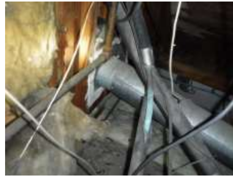
Figure 34 Refrigerant lines need insulation.
