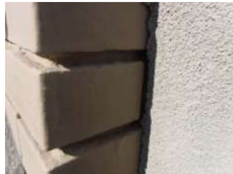
Figure 22 Caulk all vertical cracks where 2 different wall claddings meet, also caulk the windows and doors where the caulk has failed. Recommend a licensed contractor make all repairs.
