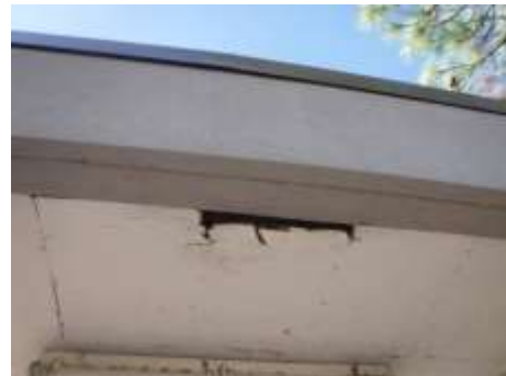
Figure 28 Soffit materials are rotten at the rear canopy, possible hidden damage; recommend a licensed contractor evaluate.
