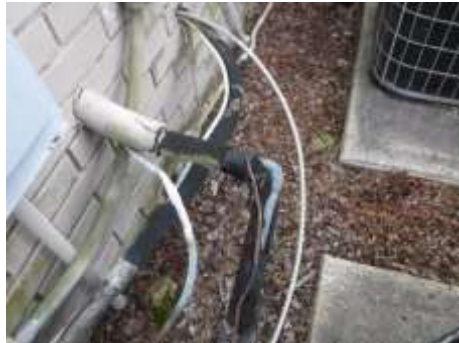
Figure 31 Lines need proper insulation.
