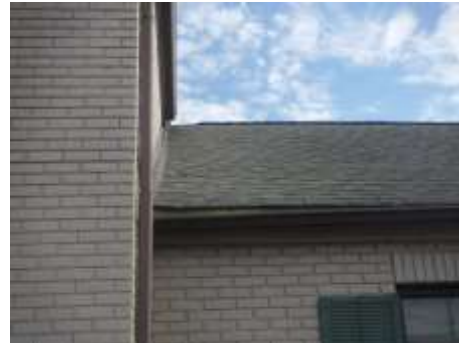
Figure 8 Gutters need proper slope and attachments are loose.
