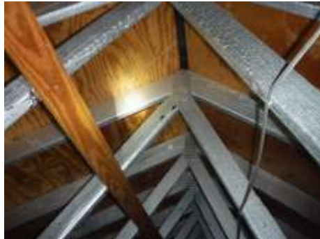
Figure 49 The trusses have been burnt, recommend an engineer evaluate.
