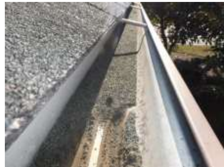
Figure 16 Shingles losing granules.
