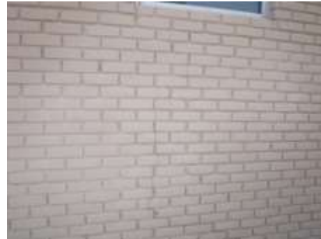
Figure 26 Same as 25 and cracks are in various locations.
