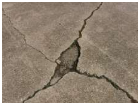
Figure 17 Driveway needs repairs in various locations. Possible trip hazard.
