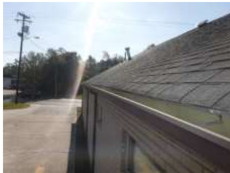
Figure 9 Improper slope and dented.
