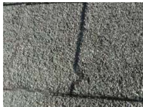
Figure 12 Shingles are damaged in various locations.
