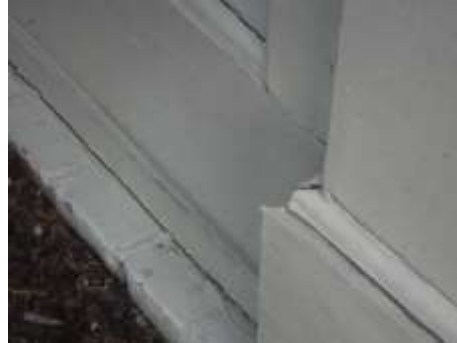
Figure 2 Trim materials need repairs.
