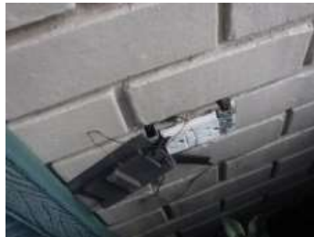
Figure 4 The GFCI outlet does not operate and the outlet needs a proper weather proof cover.
