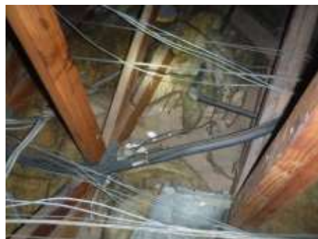
Figure 42 Replace missing insulation.
