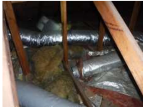
Figure 38 recommend all the debris be removed from the attic.
