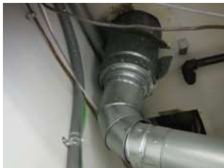
Figure 59 Vent needs repairs and seal all fire barrier wall ceiling where needed.
