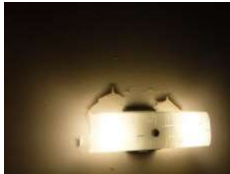
Figure 58 Both second floor baths have peeling paint.
