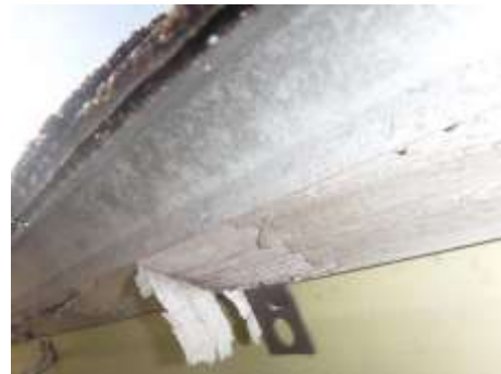
Figure 24 Fascia needs painting behind the gutters.
