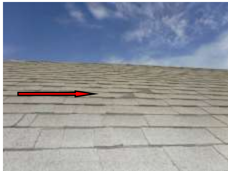
Figure 15 Broken shingle, recommend a roofer evaluate both roofs.
