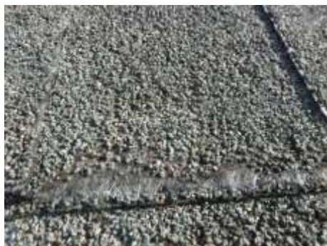
Figure 11 Roof has exposed fiberglass fibers and are brittle.
