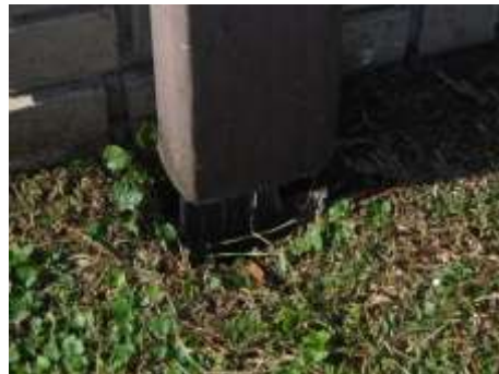
Figure 27 Recommend gutters terminate in a proper connector.
