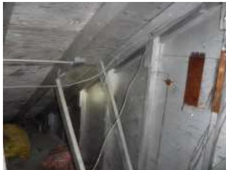
Figure 51 Wall is missing the insulation.
