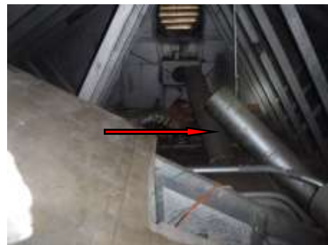
Figure 48 Recommend fresh air intake be connected.
