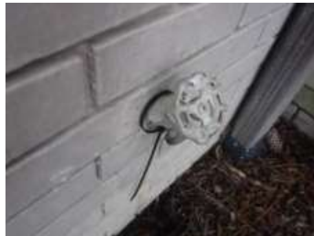
Figure 6 Recommend anti-siphon valves on the hose bibs to protect the water supply.
