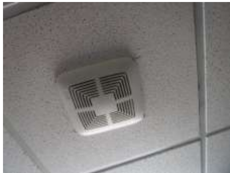
Figure 57 Bath fan is loud first floor rear bath.
