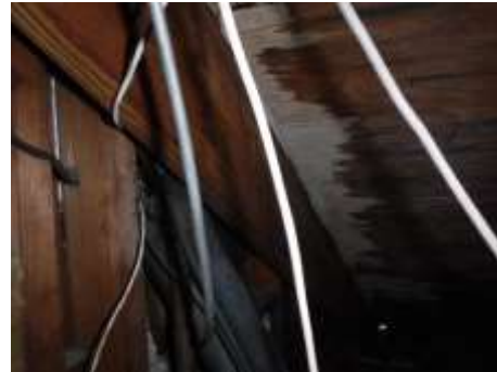
Figure 32 Moisture damage to the decking, recommend a roofer evaluate.
