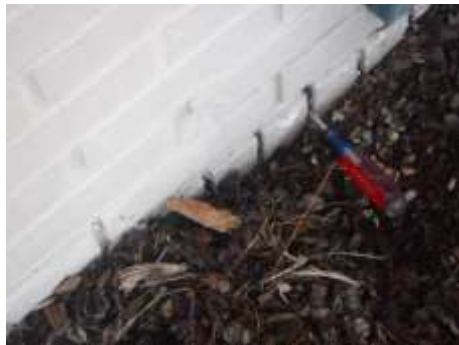
Figure 3 Weep holes need to be exposed and beds should drain in a positive direction away from the building.
