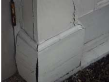
Figure 1 Trim materials need repairs.
