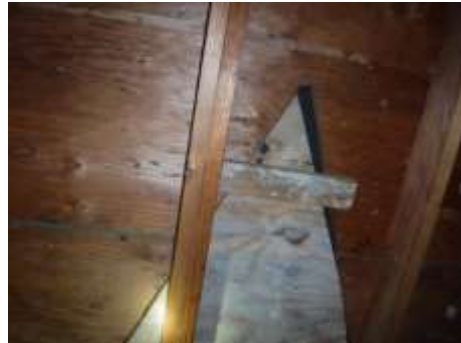
Figure 43 The attic needs additional ventilation.
