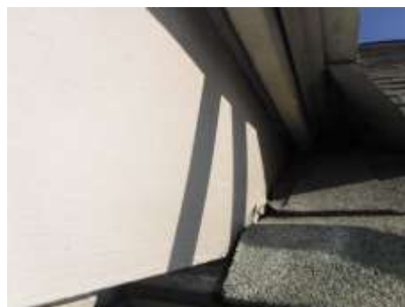
Figure 29 Should be a flashing at the fascia.
