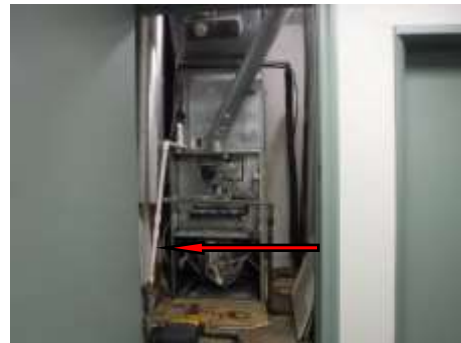
Figure 64 The on and off switch needs replacing.
