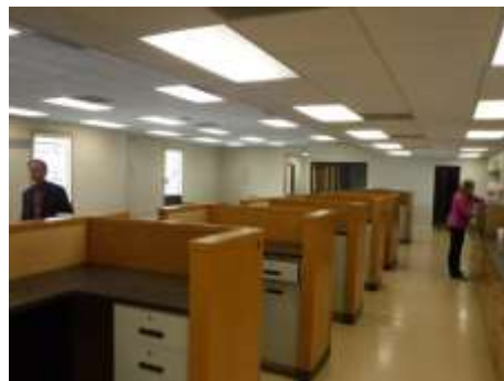
Figure 60 No grounding to the outlets at the teller bays.
