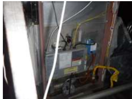
Figure 46 Recommend old AC and heater be removed and the gas line capped.
