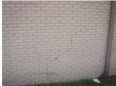
Figure 25 Typical brick cracks, recommend caulking.
