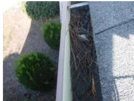
Figure 10 Gutters need cleaning.
