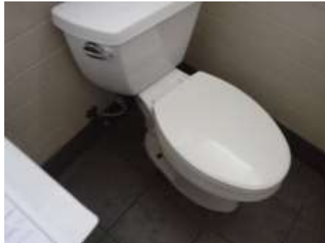
Figure 61 The toilet needs to be properly set.
