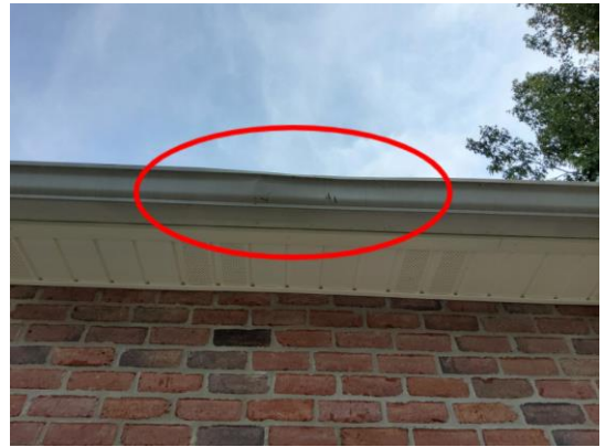
Photo 5: Minor Damage on Gutters .
