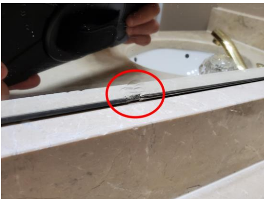
Photo 57: Bathroom Mirror Damage.
