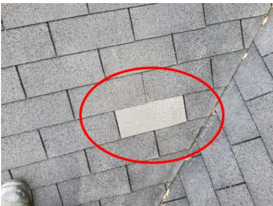
Photo 8: Prior Repairs Noted.
