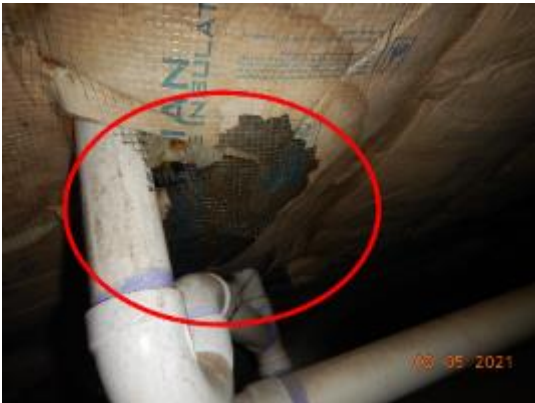
Photo 38: Shower Pan Leaks.
