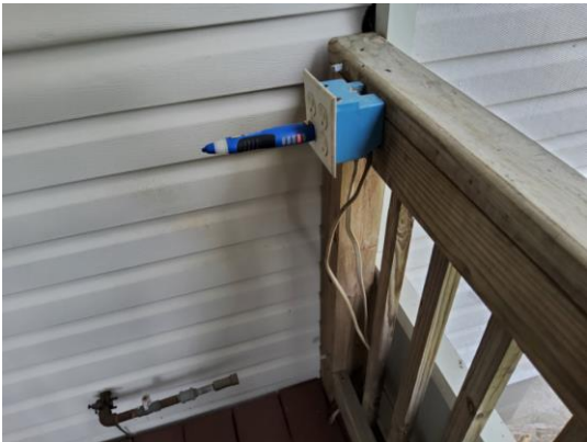
Photo 25: Wiring Exposed on Exterior .
