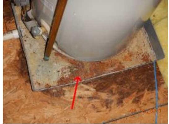
Photo 45: Corroded Drain Pan.
