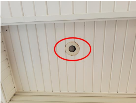
Photo 21: Trim Rings Rusting on Soffit Lights.
