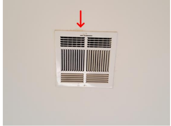
Photo 54: Water Staining - Ceiling.
