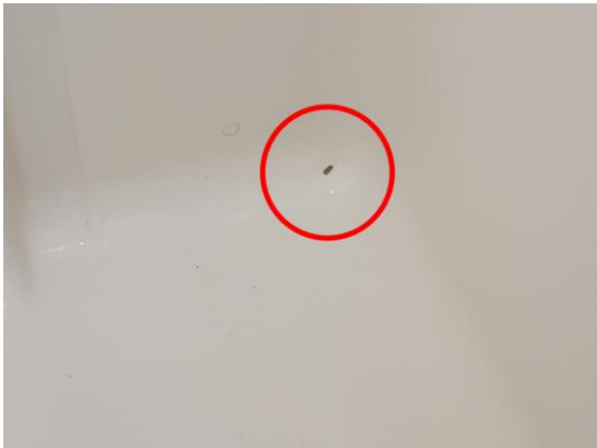
Photo 39: Shower Finish Damaged.
