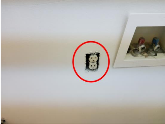
Photo 27: Cover Plate Missing.
