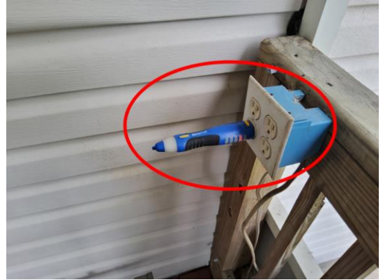
Photo 28: Ungrounded 3-prong Outlet.
