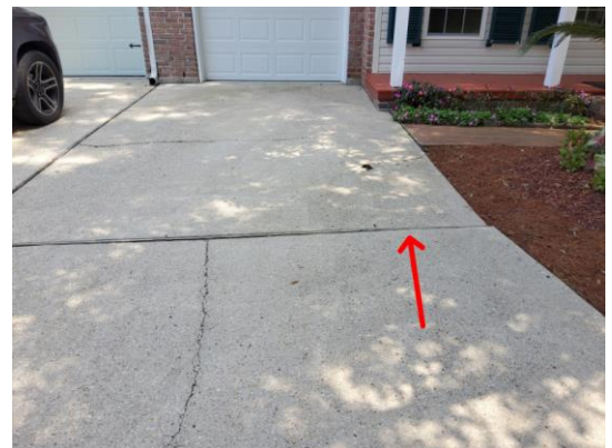
Photo 20: Driveway Settlement / Heaving.
