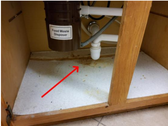
Photo 52: Cabinet Prior Water Damage- Improve.
