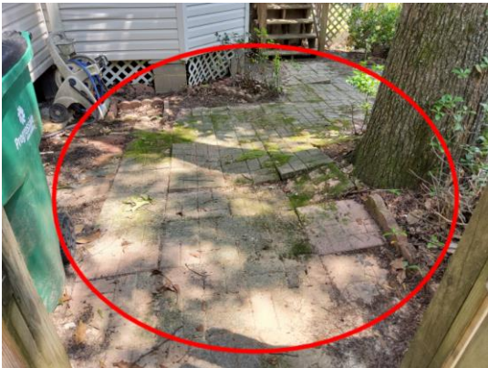
Photo 9: Walkway Trip Hazard.
