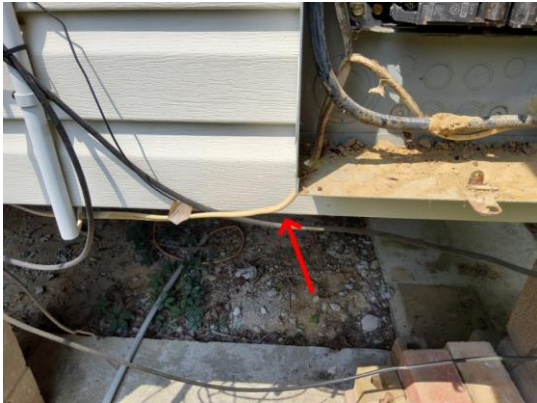
Photo 24: Wiring Exposed on Exterior .
