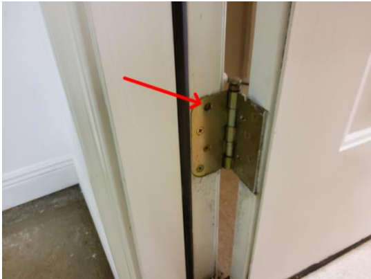
Photo 50: Door Hinge Screws Missing.
