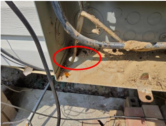
Photo 29: Cable Clamps Needed.
