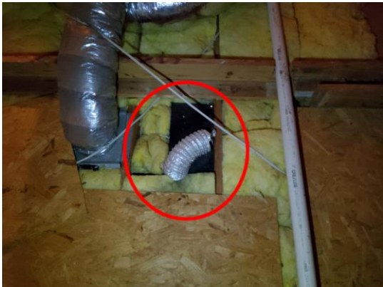
Photo 35: Vent Exhaust Vents to Exterior.
