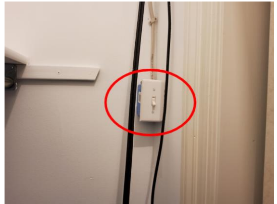
Photo 30: Light Switch Non-operable.
