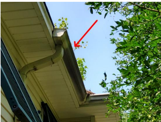
Photo 6: Gutter Cleaning Needed.
