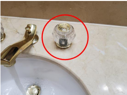
Photo 42: Sink Faucet Leaky.
