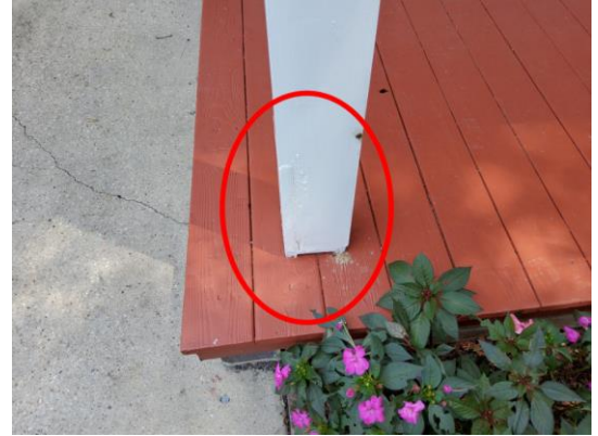
Photo 16: Wood Column Base Rot.
