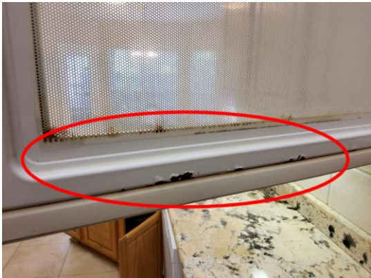
Photo 64: Rust in Microwave.
