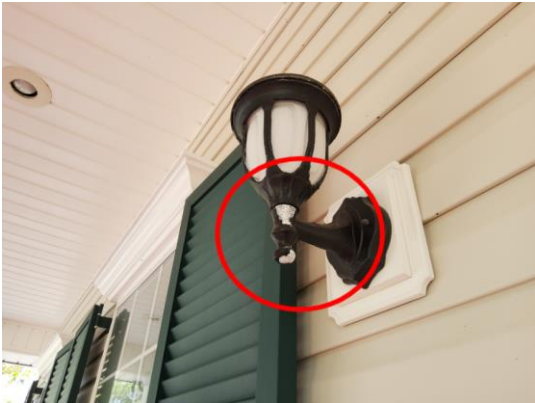
Photo 23: Light Fixture Paint Peeling.
