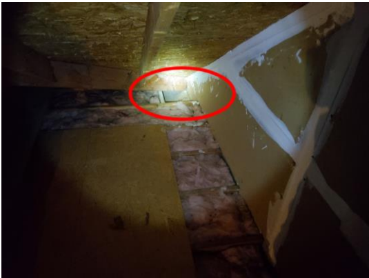
Photo 34: Missing Ceiling Insulation .
