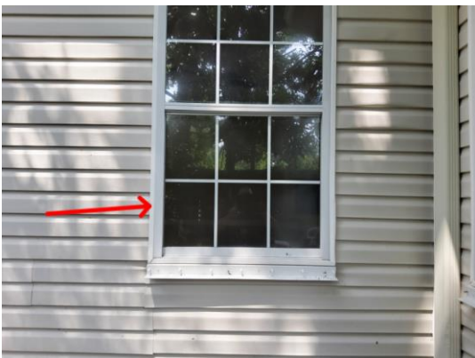
Photo 19: Window Screen Missing.
