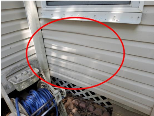
Photo 12: Vinyl Siding Damaged.
