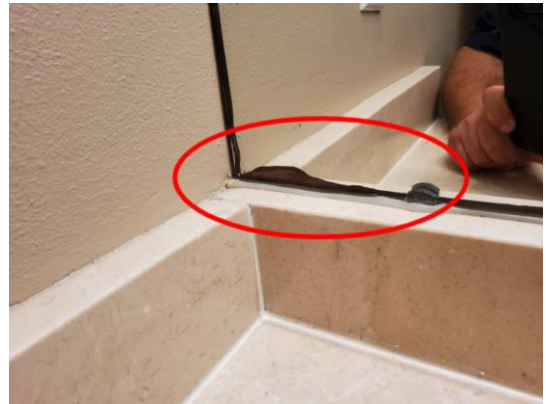
Photo 56: Bathroom Mirror Damage.
