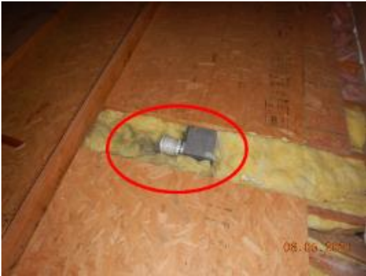
Photo 36: Vent Exhaust Vents to Exterior.
