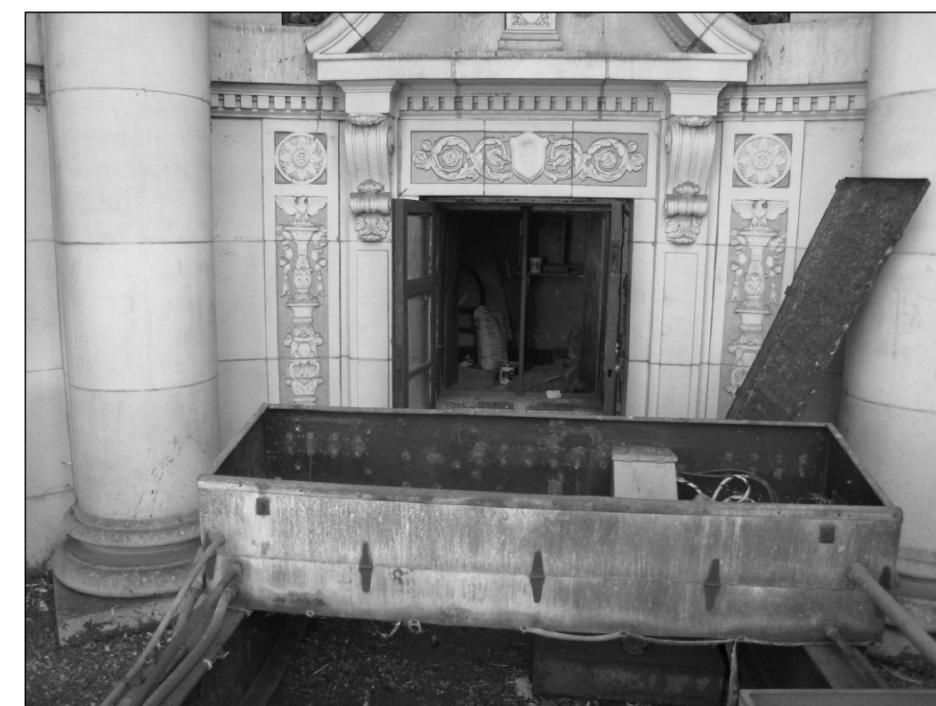
G PHOTO 2081 REAR WALL OF ALCOVE; NOTICE CRACK IN COLUMN BASE, PATCH AND REPAIR TO MATCH EXISTING
