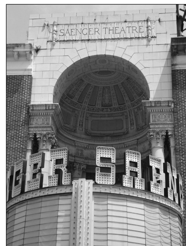
E PHOTO DSC01949 OVERVIEW OF ALCOVE; REMOVE VEGETATION, PATCH AND REPAIR, CLEAN AND RESTORE
