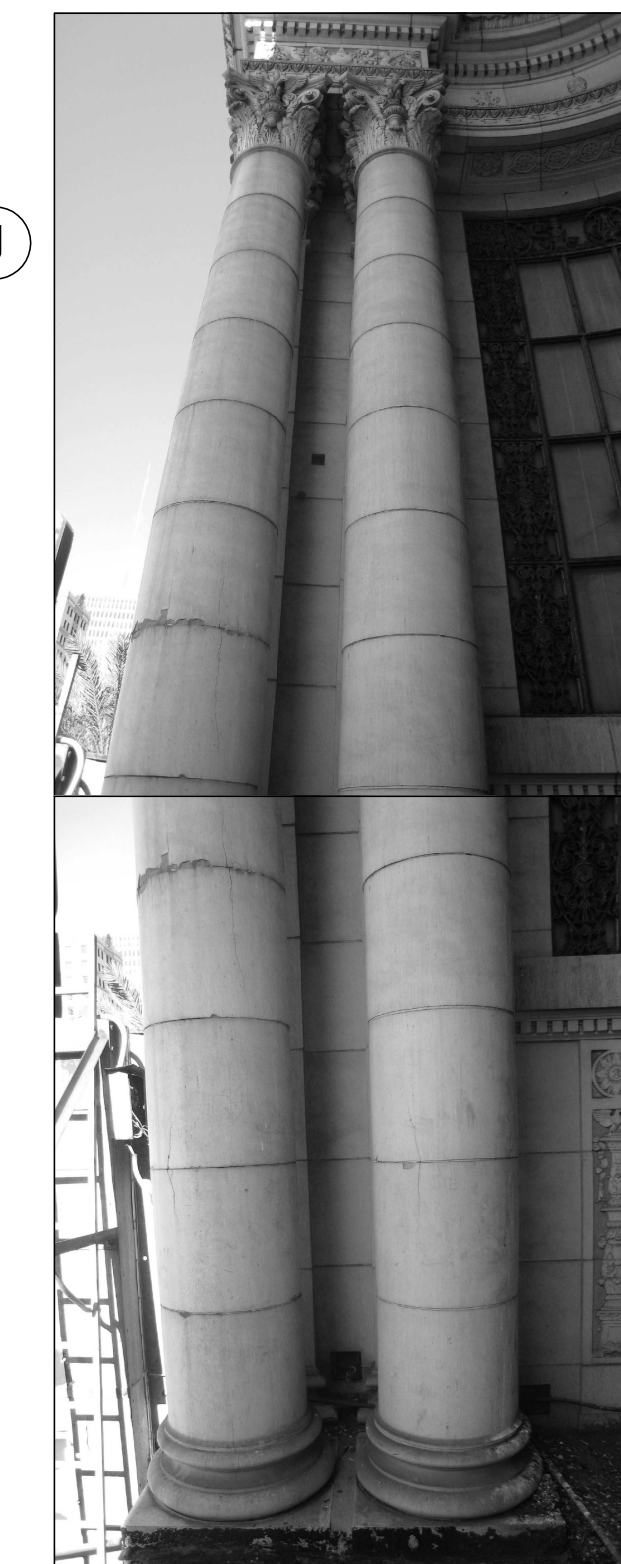
B PHOTOS 2077-2078 CRACKS AND JOINT DAMAGE ON COLUMN SURFACES; GLAZING DELAMINATING FROM COLUMNS, RESTORE AND REPOINT
