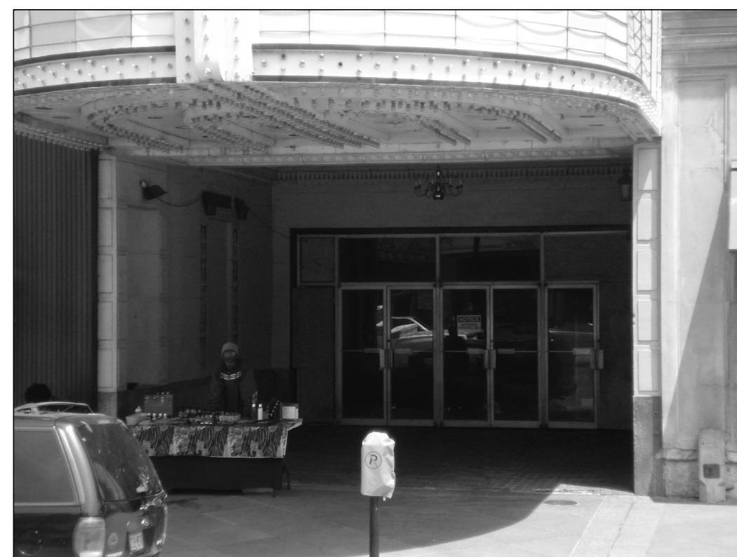
C PHOTO DSC01596 MAIN CANAL STREET ENTRANCE; NOTE DAMAGES TO THE TERRA COTTA ADJACENT TO THE MARQUIS
