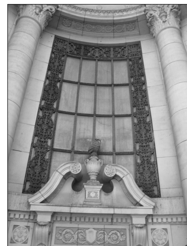
D PHOTO 2072 PEDIMENT IN CENTER OF ALCOVE; CLEAN AND REPOINT AS REQUIRED TO RESTORE TO ORIGINAL
