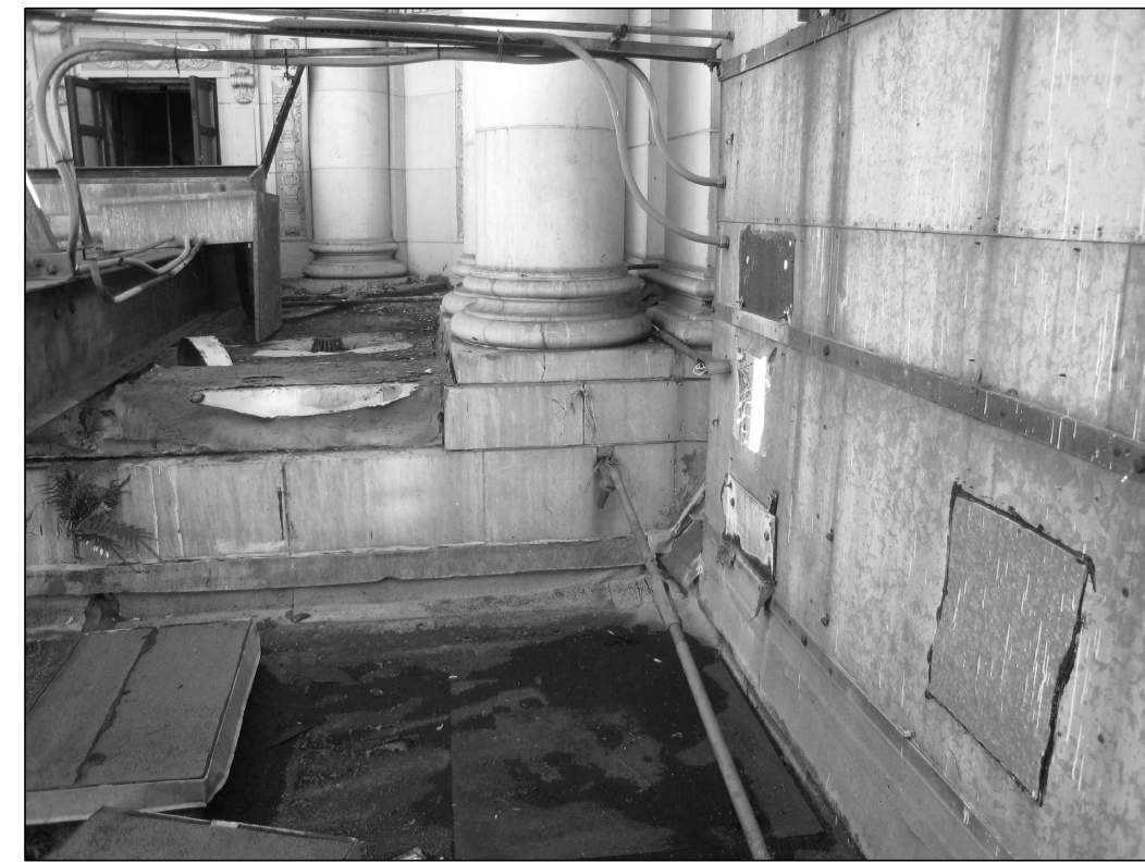
I PHOTO 2091 TERRA COTTA PENETRATIONS BEHIND MARQUEE; PATCH AND REPAIR, REMOVE ALL METAL STAINS AND RESTORE GLAZING TO ORIGINAL TO MATCH ADJACENT.
