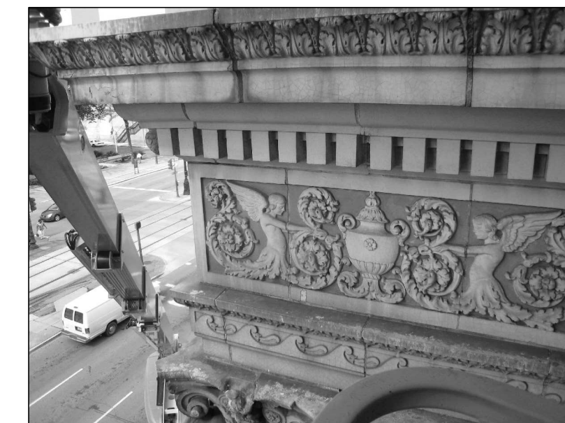
K PHOTO 1931 SCULPTURAL FRIEZE ABOVE COLUMNS - REMOVE STAINS AND REPOINT, CHECK FOR SECURITY
