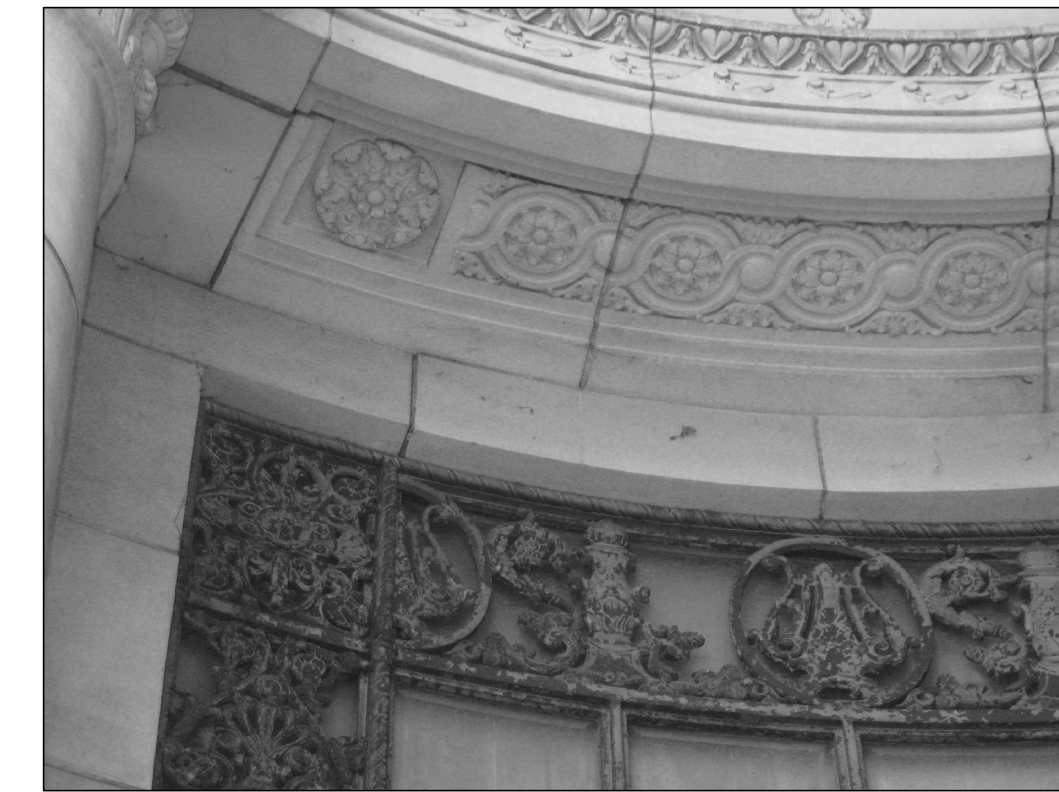
J PHOTO 2084 TERRA COTTA JOINTS ABOVE GLAZING; REPOINT AND REMOVE ALL STAINS, VERIFY CONDITION
