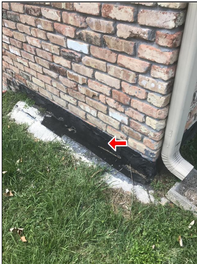
5.0 Item 1(Picture) black coating on foundation and 1st row of bricks
