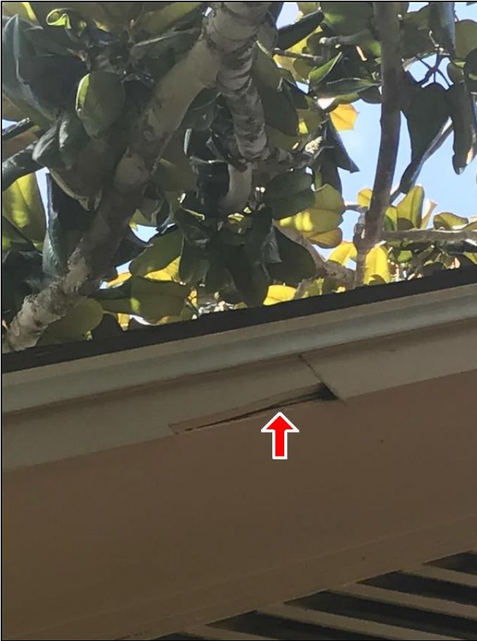
2.5 Item 1(Picture) broken/damaged fascia board
