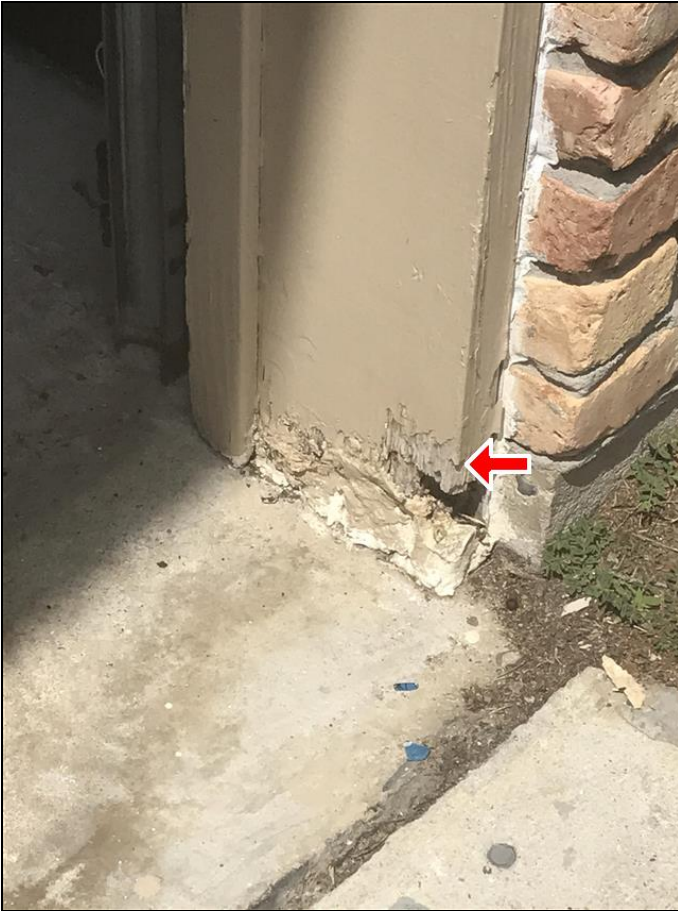
2.1 Item 2(Picture) damage to garage door frame
