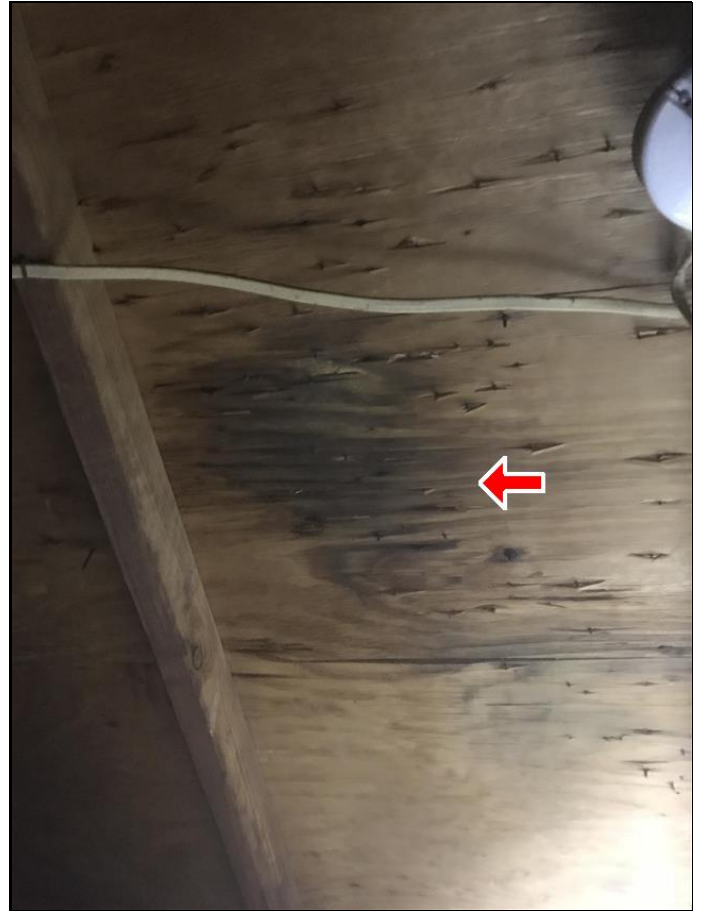
5.5 Item 2(Picture) moisture stains
