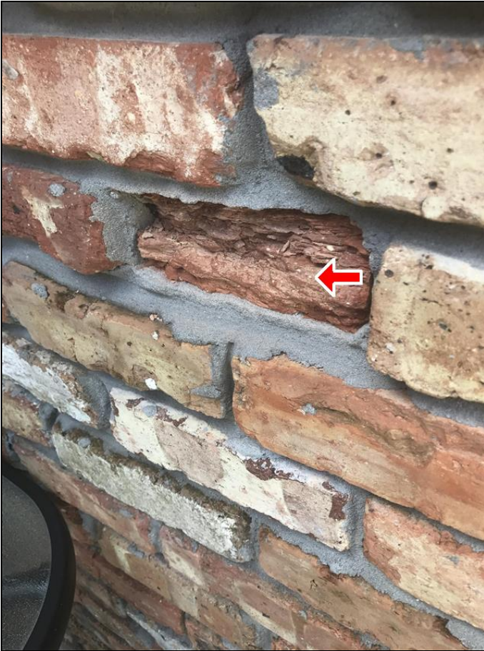
2.0 Item 3(Picture) crumbling brick in wall
