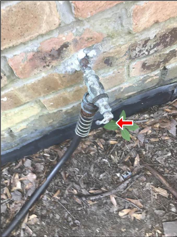
6.1 Item 1(Picture) hose handle broken
