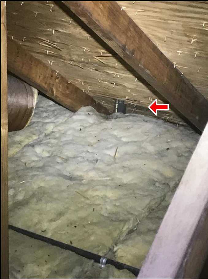
5.5 Item 1(Picture) moisture stains by plumbing vent
