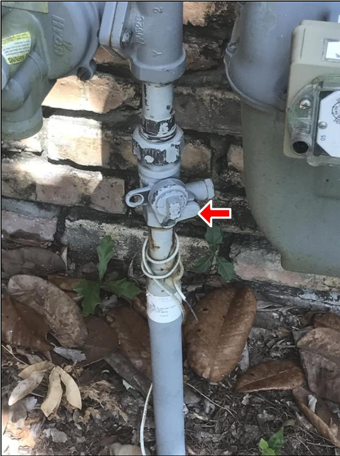
6.5 Item 1(Picture) main gas shut off valve
