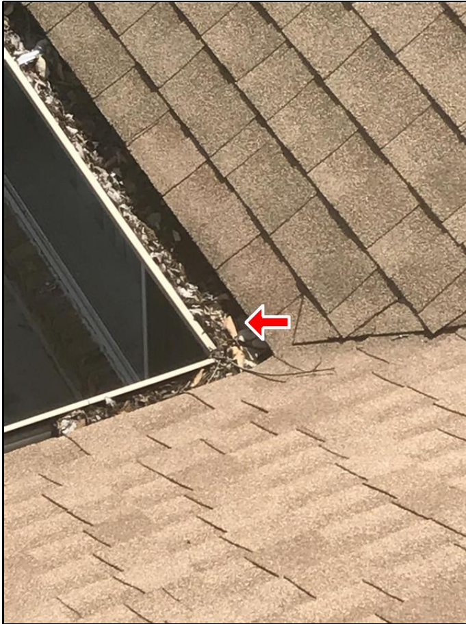
1.3 Item 1(Picture) gutter debris
