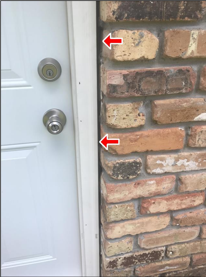
2.1 Item 1(Picture) door frame needs sealing
