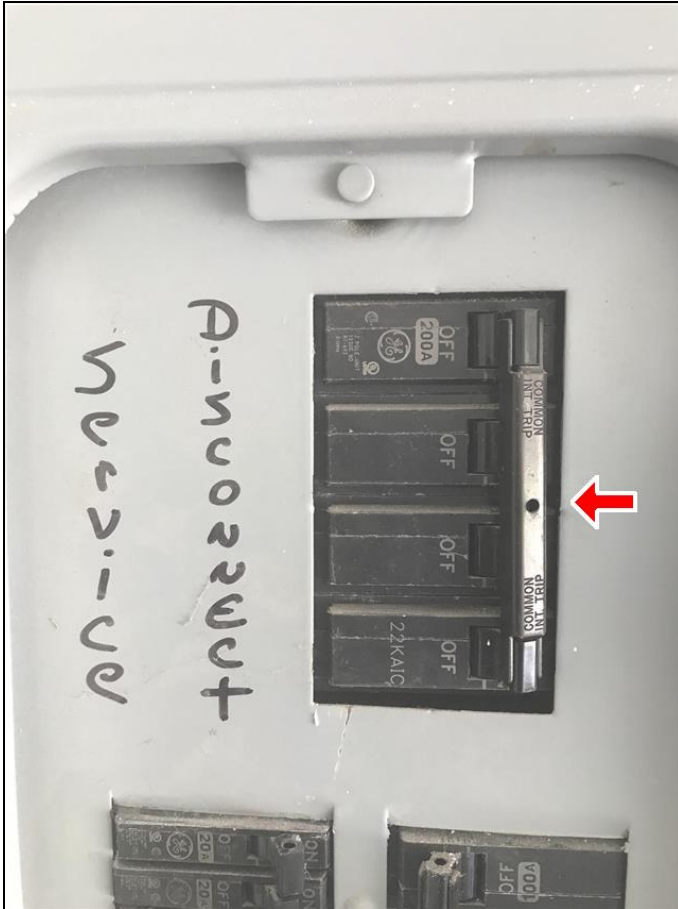
7.6 Item 1(Picture) main electrical disconnect
