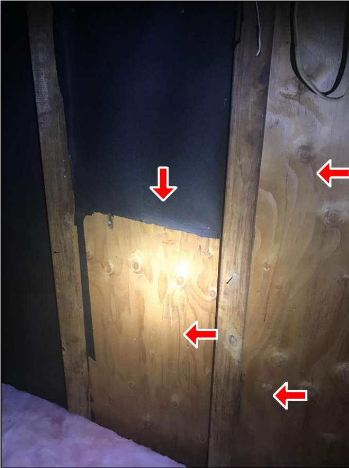
5.5 Item 3(Picture) black barrier missing in areas
