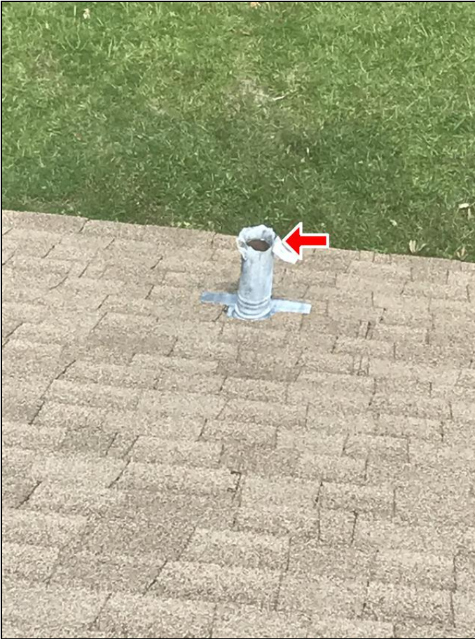
1.1 Item 1(Picture) rodent damage on cover
