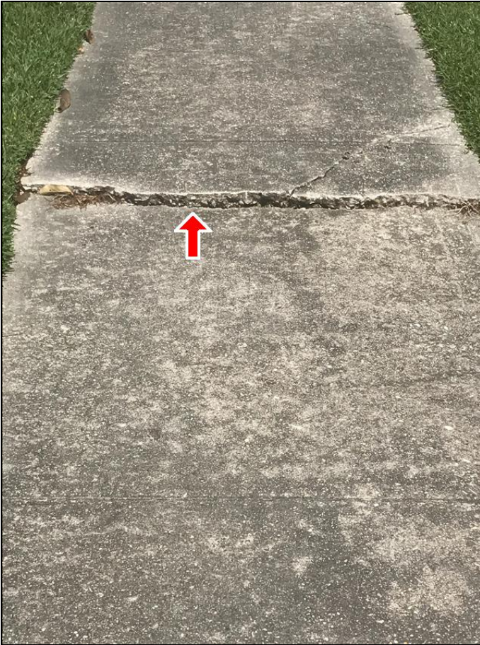
2.4 Item 1(Picture) possible trip hazard
