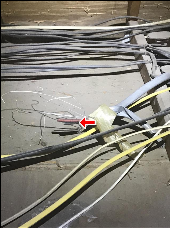
7.3 Item 1(Picture) open wiring
