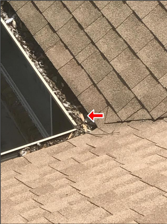
1.3 Item 1(Picture) gutter debris
