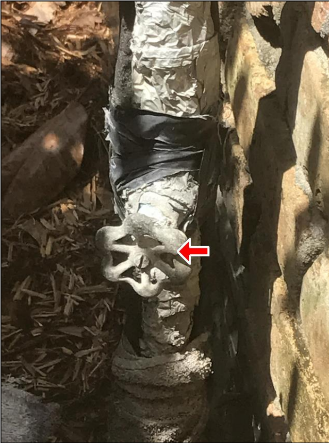
6.3 Item 1(Picture) main water shut off
