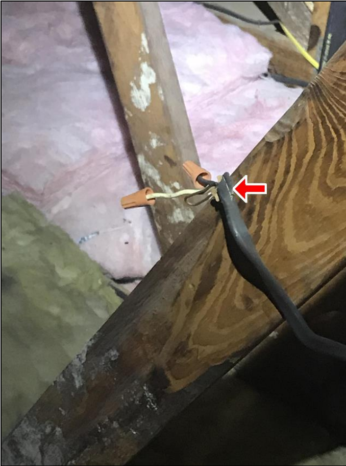
7.3 Item 3(Picture) open wiring in attic
