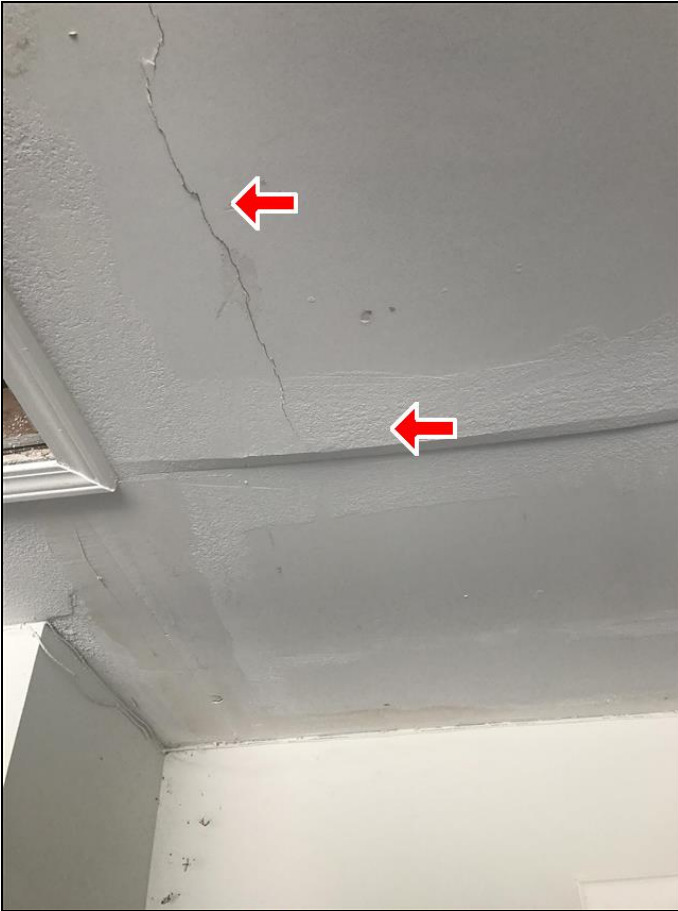
3.0 Item 1(Picture) ceiling cracks, drywall loose in garage
