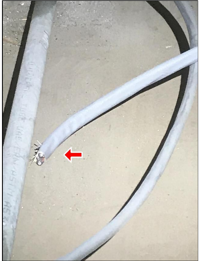
7.3 Item 2(Picture) open wiring in attic
