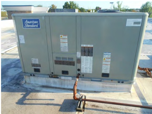
27. Gas-fire rooftop HVAC package unit
