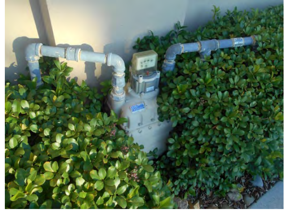
20. Natural gas service
