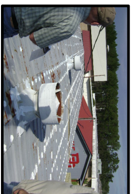
DAMAGED ROOF AND VENTILATORS N.T.S.
