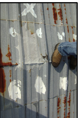
DAMAGED ROOF RIDGE N.T.S.
