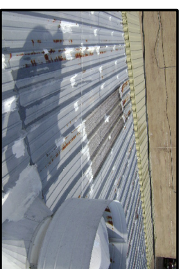
DAMAGED FIBERGLASS ROOF PANELS N.T.S.
