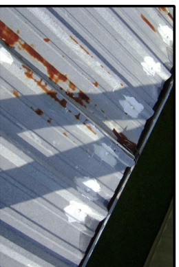
DAMAGED ROOF PANELS N.T.S.
