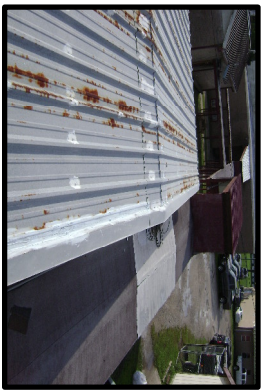
DAMAGED ROOF END RAKE N.T.S.
