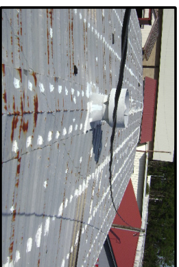
DAMAGED ROOF AND VENTILATORS N.T.S.
