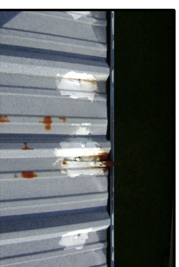
DAMAGED ROOF PANELS N.T.S.
