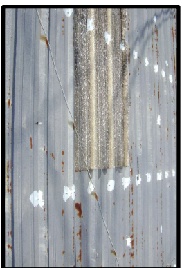
DAMAGED FIBERGLASS ROOF PANELS N.T.S.
