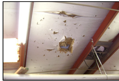
DAMAGED INTERIOR CEILING INSULATION N.T.S. L A1|A2
