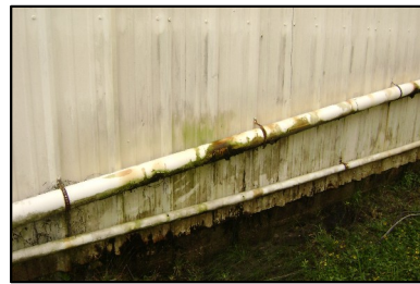
DAMAGED EXTERIOR WALL PANELS N.T.S. N A1|A2
