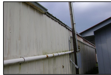
"CODE VIOLATION" DRAINAGE OVER ELECTRICAL N.T.S. P A1|A2
