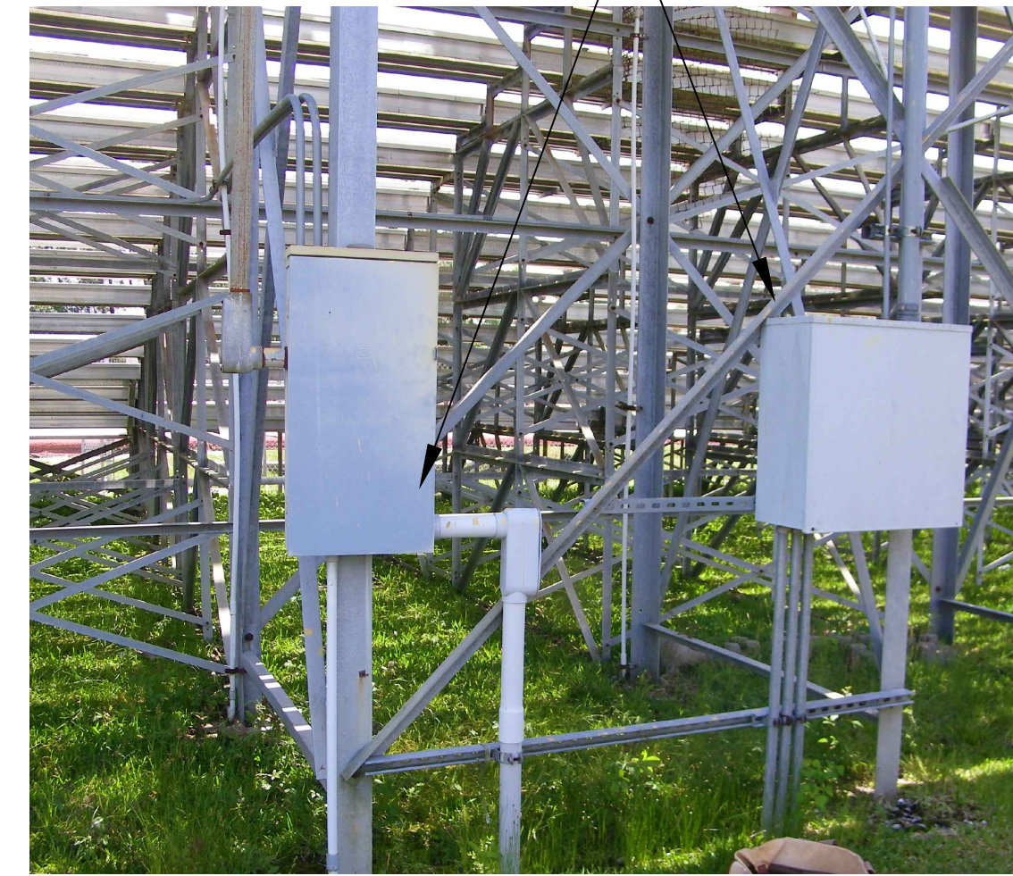
REMOVE ALL ELECTRICAL POWER FROM SUPPORTS AND SAVE FOR REINSTALLATION ON NEW PRESS BOX.
