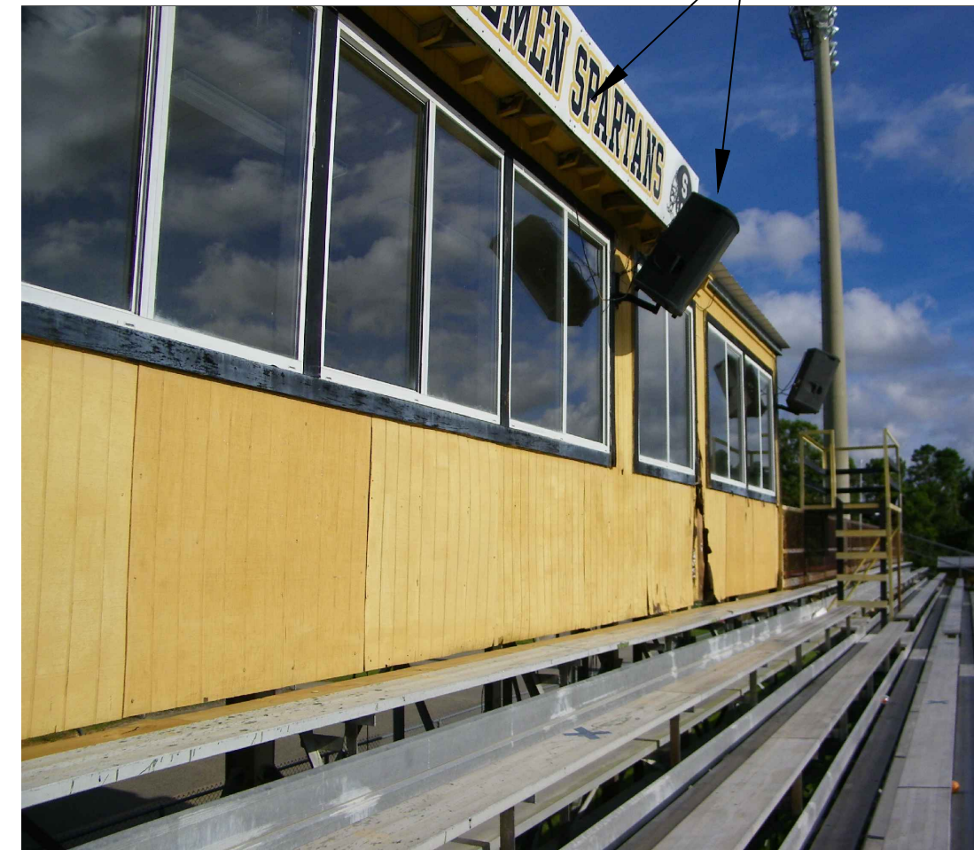
REMOVE ALL SPEAKERS, CAMERAS AND SIGN TO REINSTALL ON NEW PRESS BOX.
