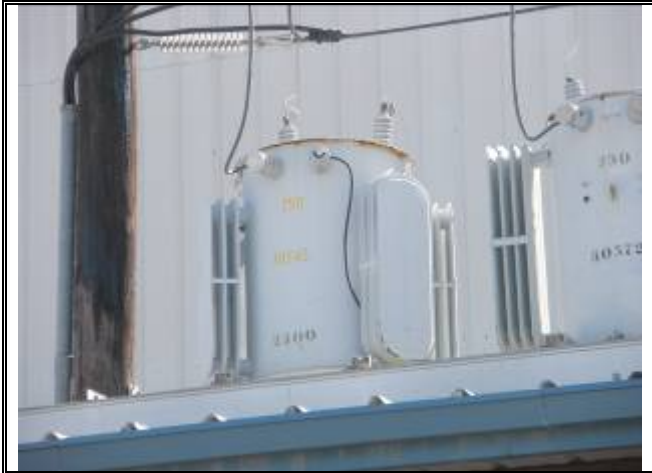
Photograph No. 079: transformers
