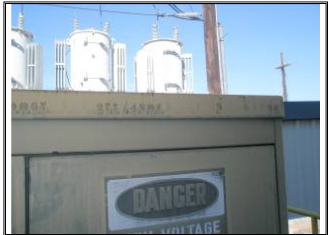
Photograph No. 077: transformers
