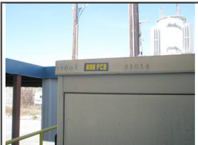
Photograph No. 075: transformers
