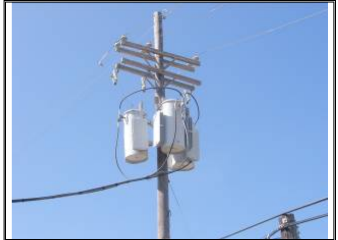
Photograph No. 082: transformers
