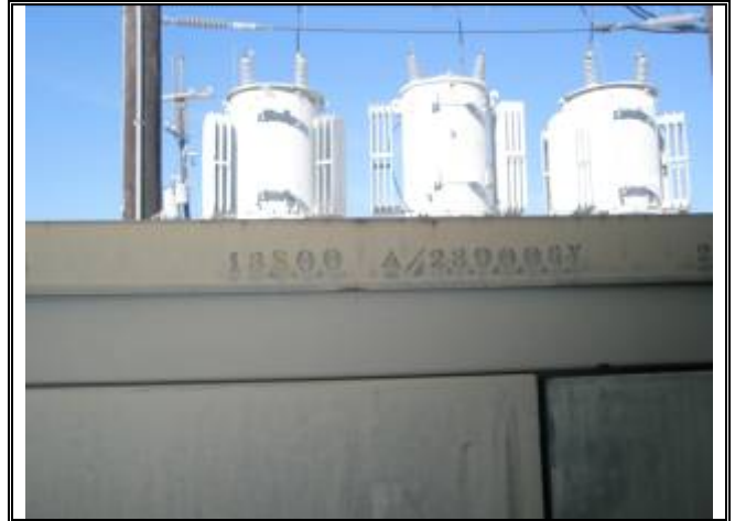
Photograph No. 076: transformers
