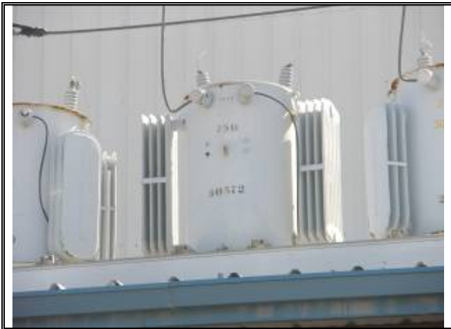
Photograph No. 080: transformers
