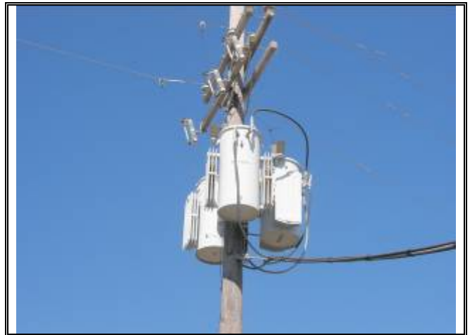
Photograph No. 083: transformers
