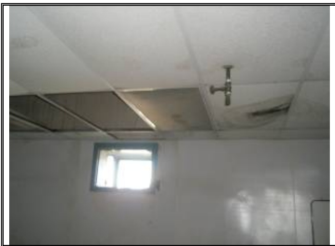
Photograph No. 051: inside compressor room of bldg 4
