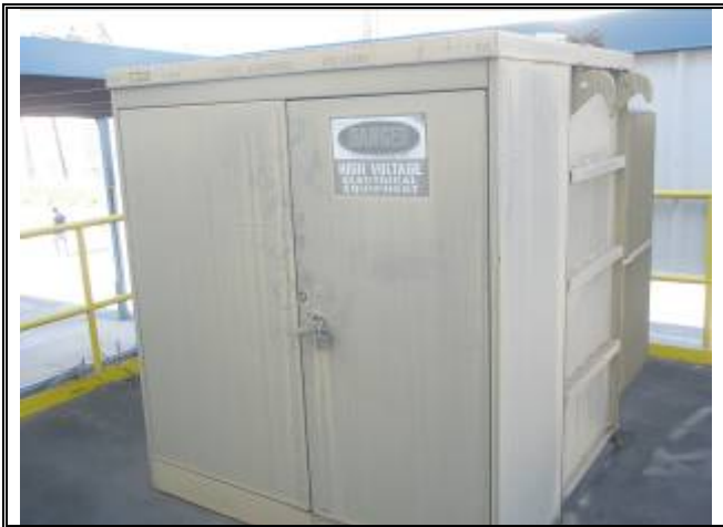
Photograph No. 074: transformers
