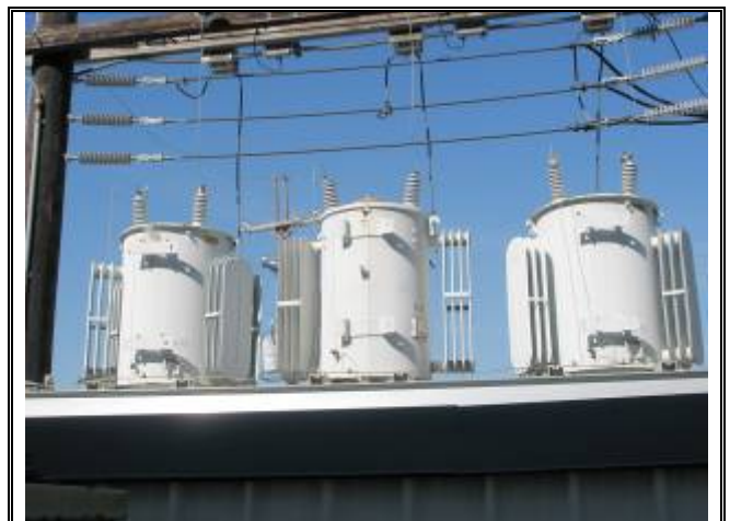
Photograph No. 078: transformers
