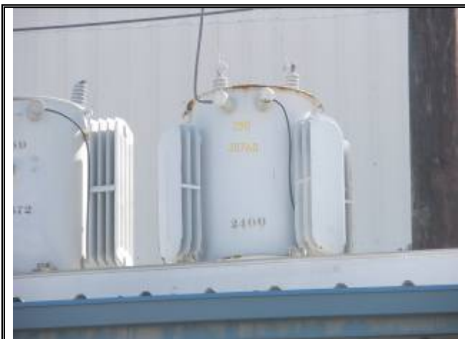
Photograph No. 081: transformers
