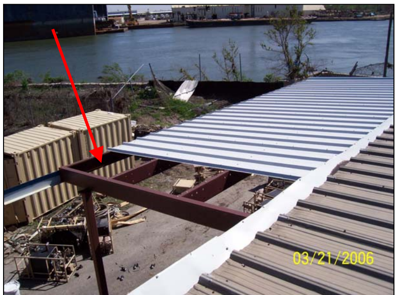
9. Overview & damage to canopy.
