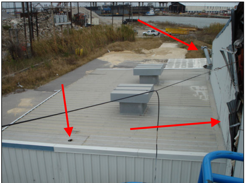
15. Missing and detached vents also damaged side panels.
