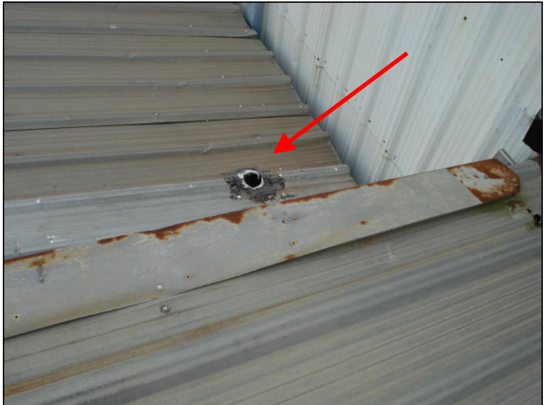
10. Vent pipe broken off flush with roof.
