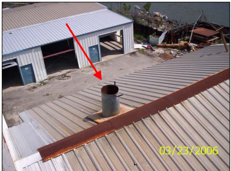
3. Missing 18" turbine vent.
