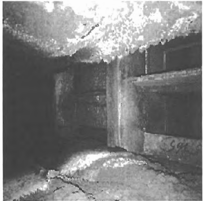
Photo of inside of HVAC taken by HVAC contractor, supplied by St. Mayfield.
