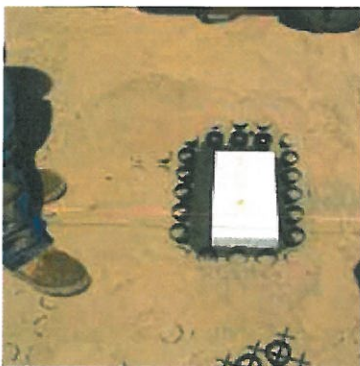
Grasspave2 is cut and a concrete brick is placed inside a Grasspave2 installation. Notice that the concrete is slightly raised above the top of the rings.
