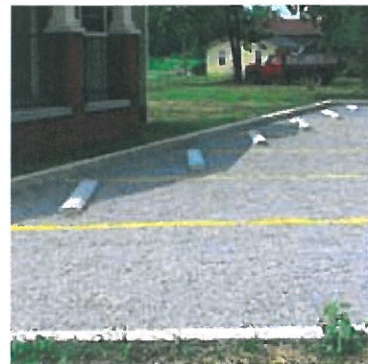
Painting is an option for Gravelpave2. This parking lot shows an attractive combination of painted lines and curb stops.
