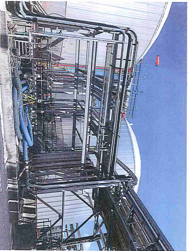
PHOTO 1 - TANK FARM C MANIFOLD AND PIPERACK
