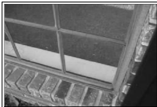
2 holes in window pane covered with packing tape
