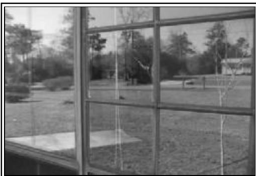
cracked window pane covered with silicone and packing tape
