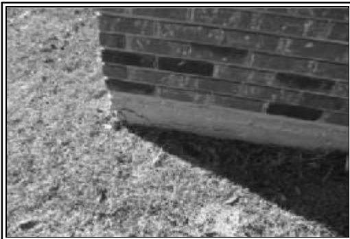
contractor to verify slab/cracked on den corner
