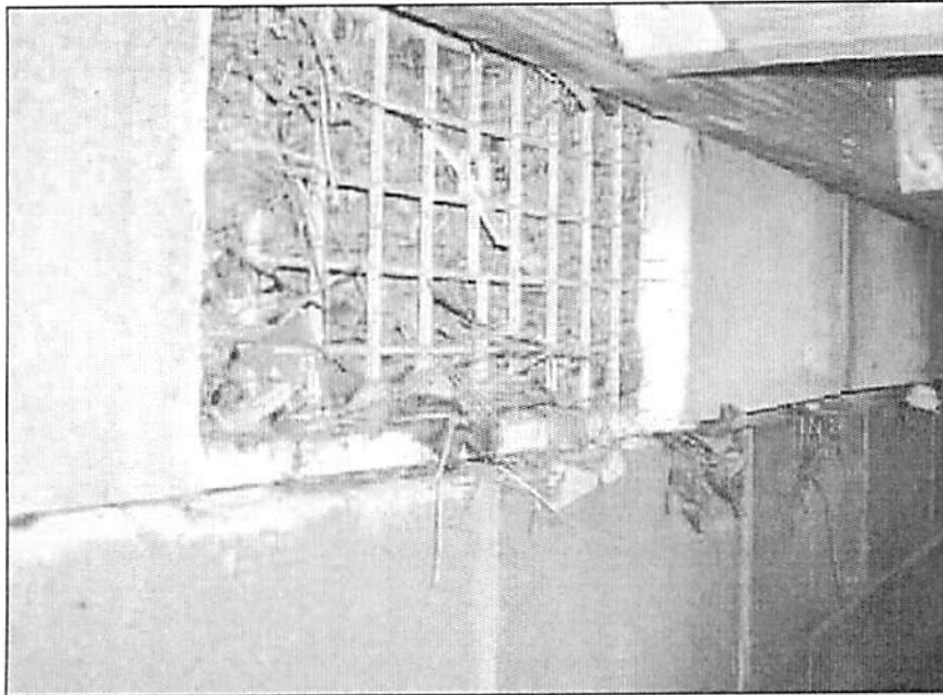
Figure 15. Typical air vent clogged by flood debris
