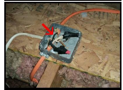
Missing junction box cover in main attic
