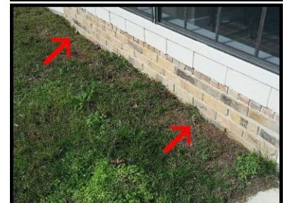
High soil/grading blocks slab
