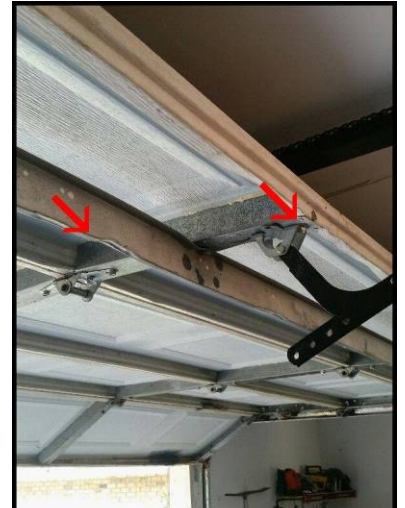
Dents & damage noted
