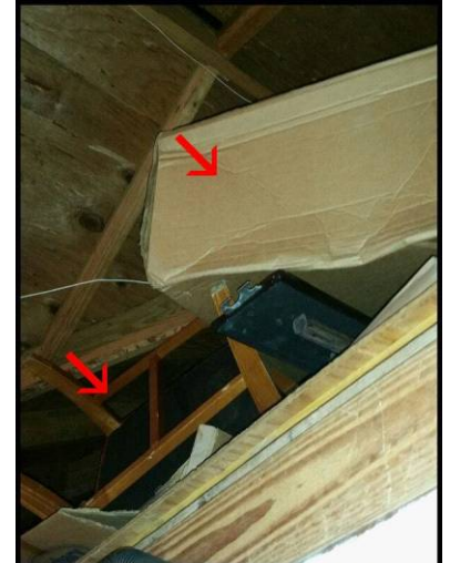
Personal items block garage attic entrance
