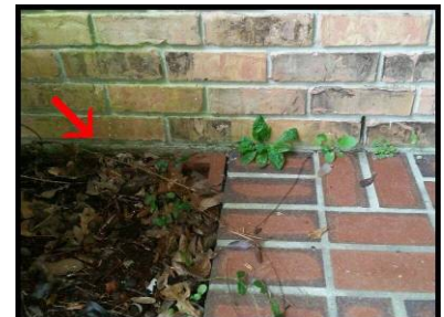
Some areas of slab not visible
