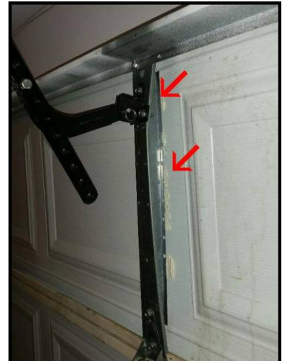
Damage at the control arm
