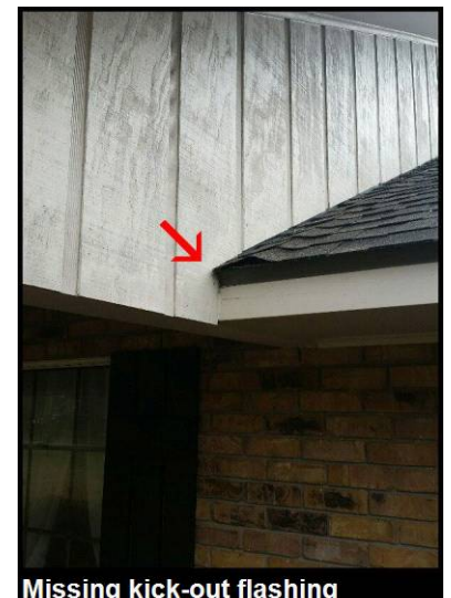
Missing kick-out flashing
