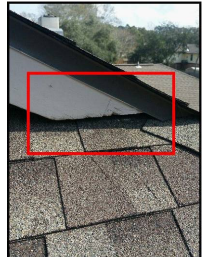
Missing flashing & pest entry point
