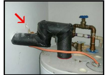
No outlet / disconnect
