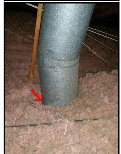
Improper clearance to combustibles
