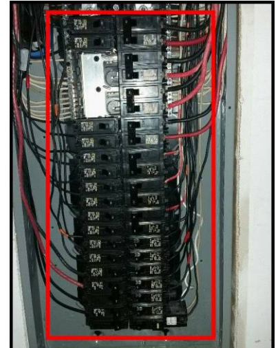
Close up of main panel circuits. No AFCI's
