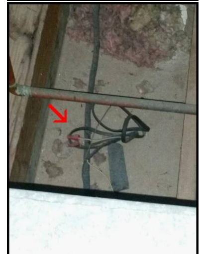
Exposed wires in main attic at left
