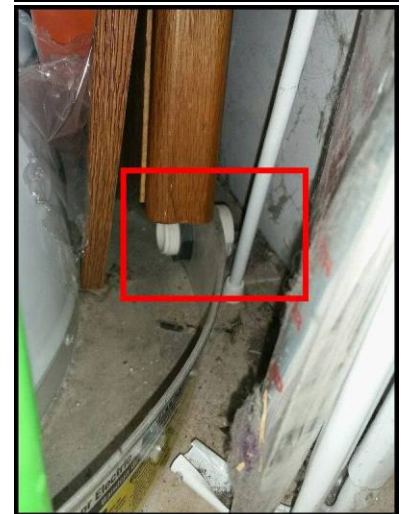
Drain pan missing the drain line
