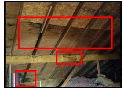
Evidence of past/present leaks
