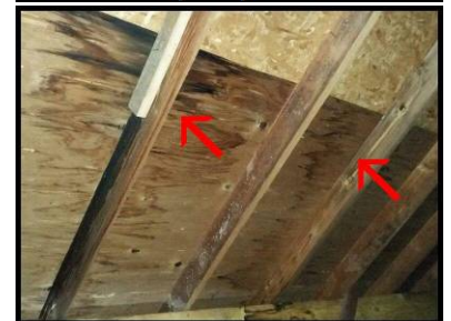
Close up of the stains
