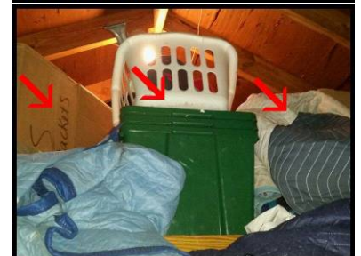
Personal items block garage attic entrance
