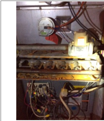
Repair: Water stains and rust in the furnace unit.
