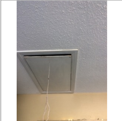
Repair: Attic stairs not sealed in the garage.
