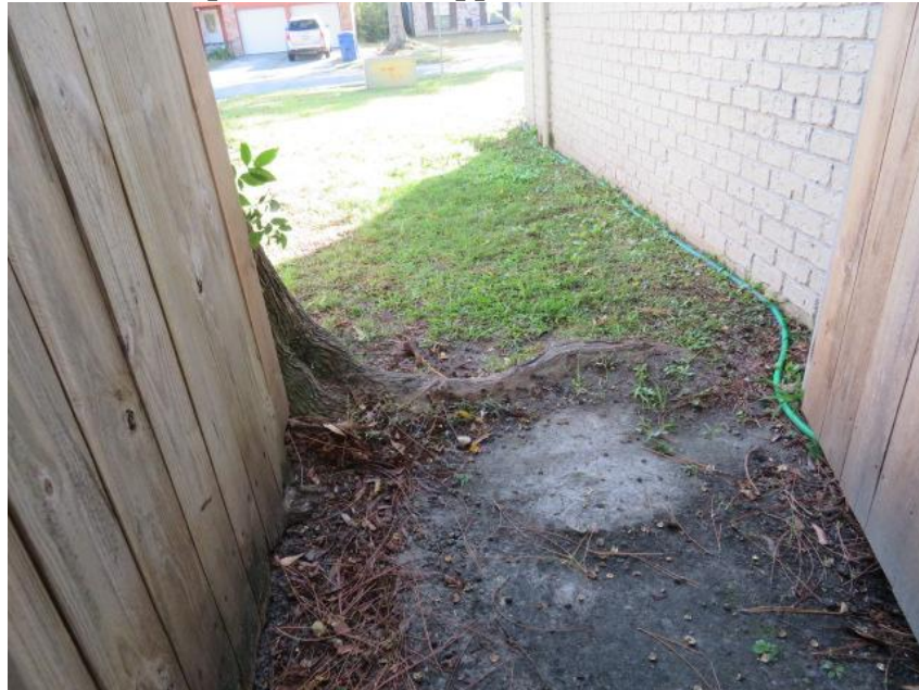
Picture #6, exposed tree root approx 4.5' from the brick crack
