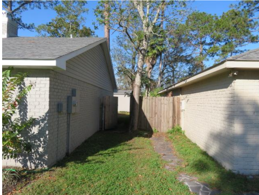
Picture #5, view of Tallow tree near brick crack
