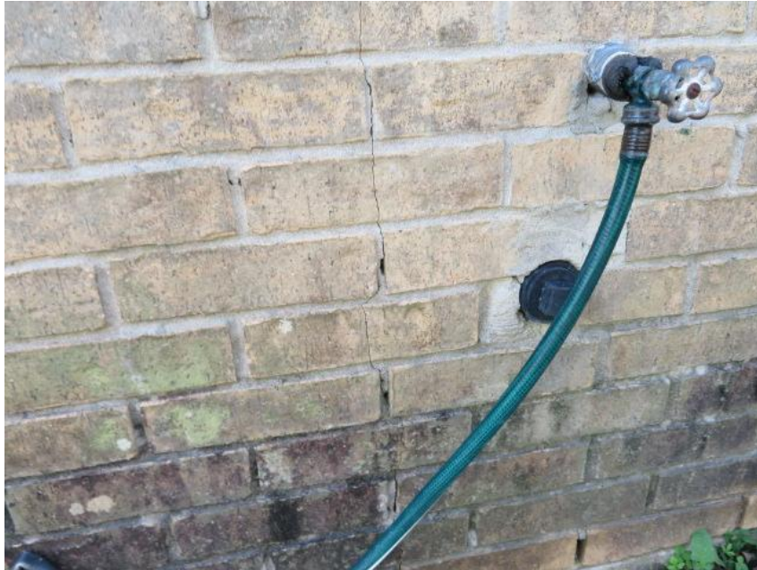
Picture #9, affected area
