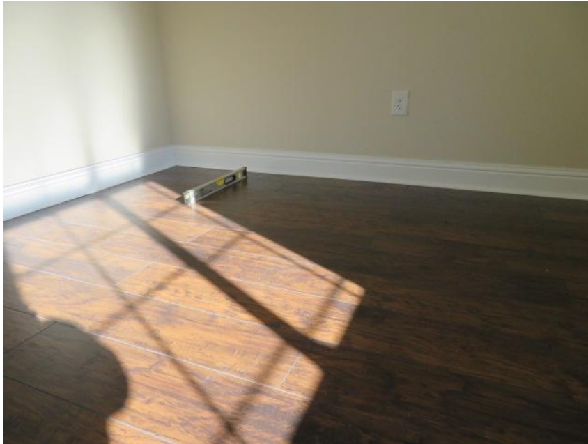
Picture #13, BRM affected area.
