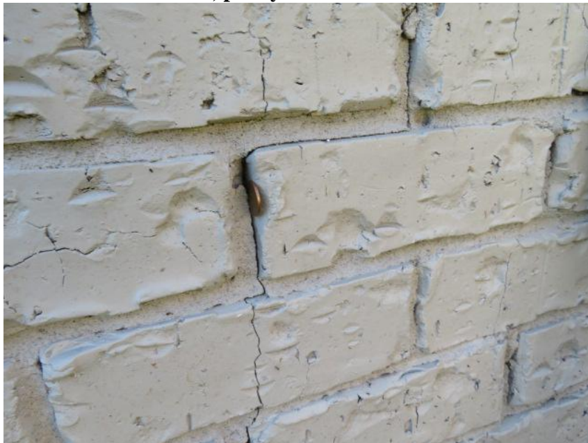
Picture #10, penny in widest brick crack
