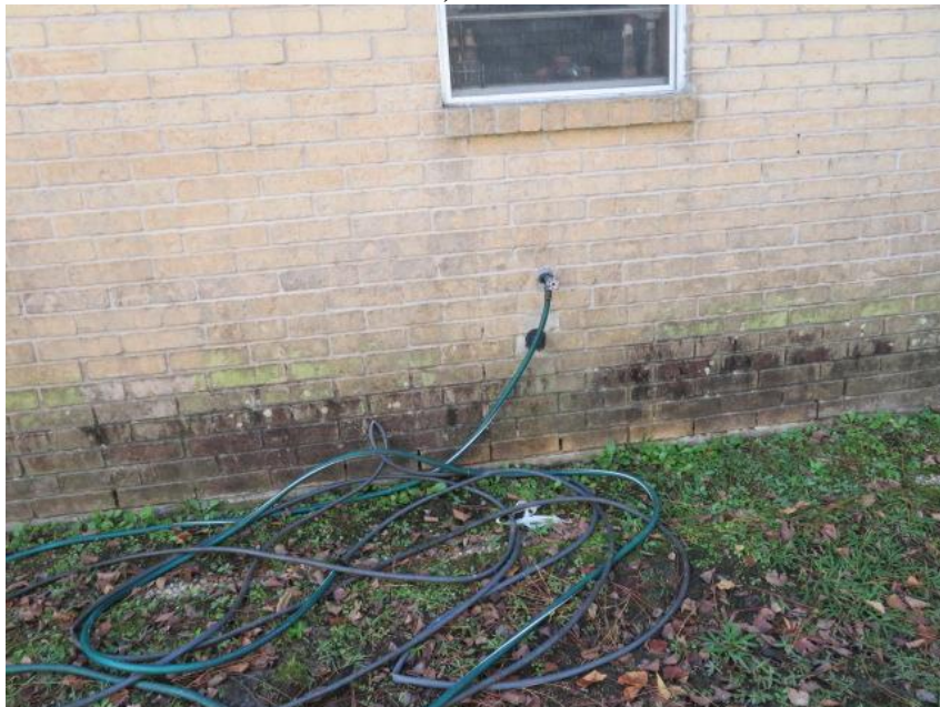
Picture #8, affected area
