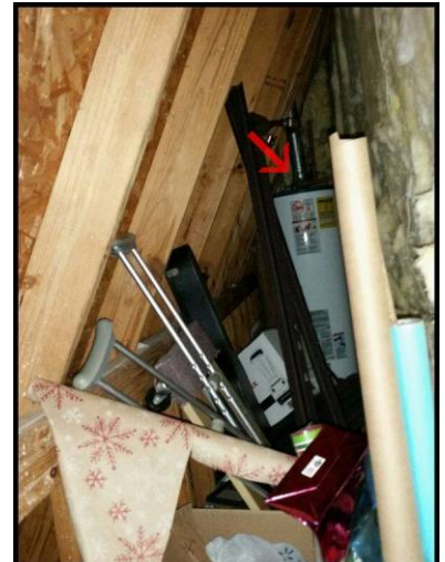
Unable to access left water heater
