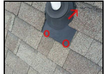
Missing face nails / Cracked shingle
