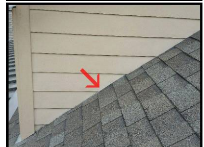
Missing moisture break at intersection
