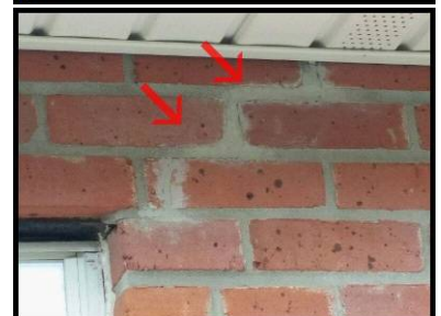
Right side of house
