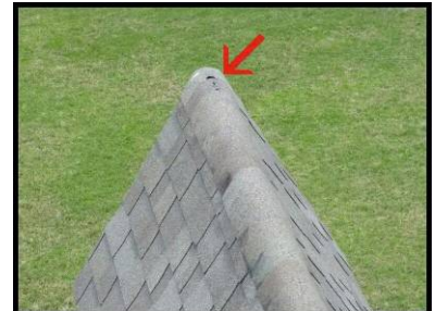
Damaged shingles at dormers
