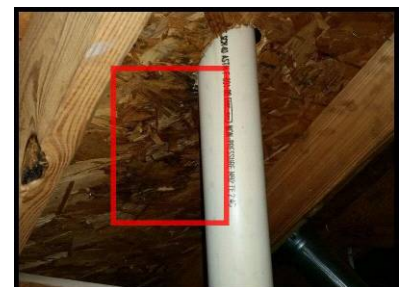
Moisture stains noted at vent pipe
