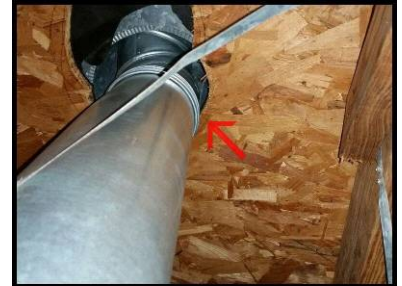
Improper clearance to combustibles
