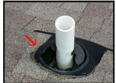
Damaged vent boot over master area
