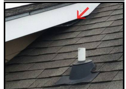
Loose soffit at rear
