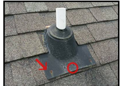
Seal ALL nails / Missing Face nails
