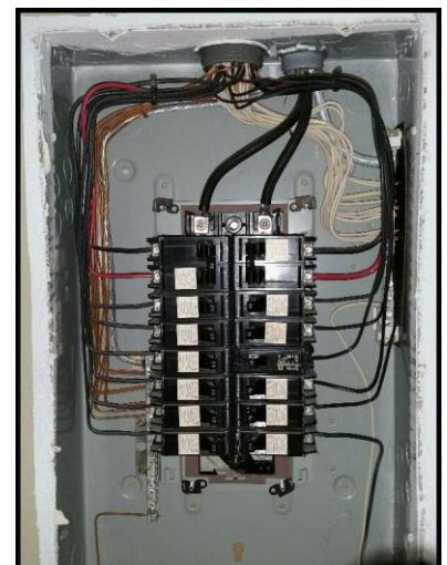
Panel at laundry / No AFCI circuits
