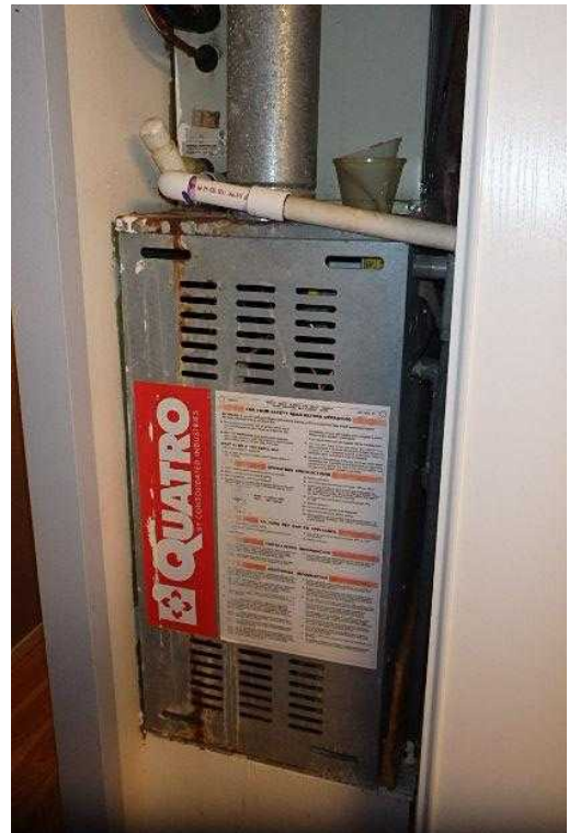
#80 HVAC unit in the kitchen.
