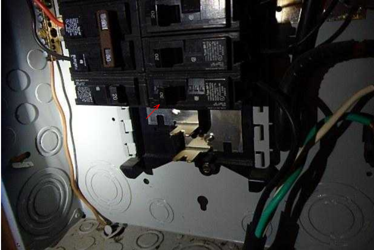
#65 30 amp circuit for the extension cord.
