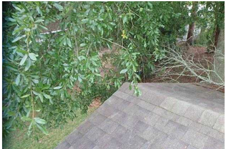
#40 Tree limbs close to the roof in the left rear.
