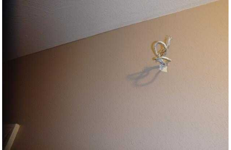
#94 No door chime in the hallway.
