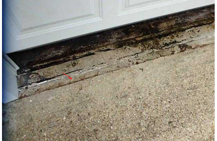
#50 The driveway is higher than the garage on one side.
