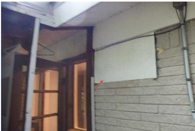
#31 Wood over opening.
