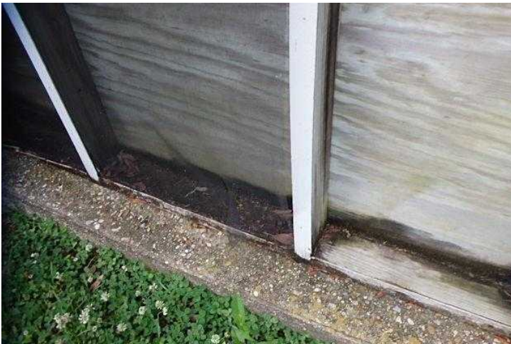
#23 Plywood added on the inside with hold moisture at the sill plate.
