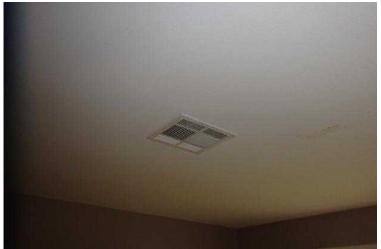
#88 No light fixture in the den.
