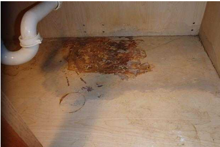
#75 Past leaks present.
