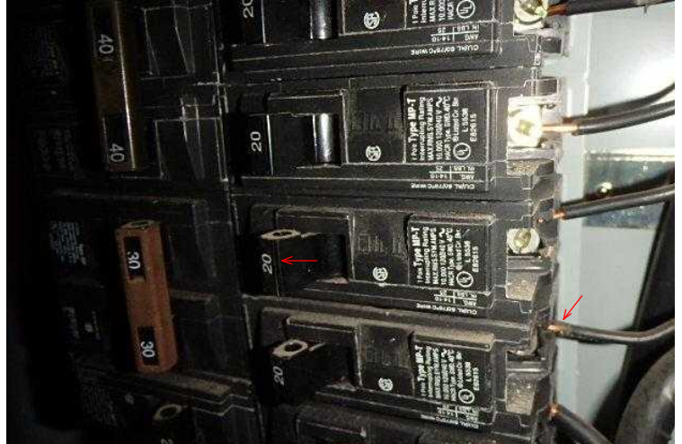
#66 Some of the breakers are oversized. Fire hazard.
