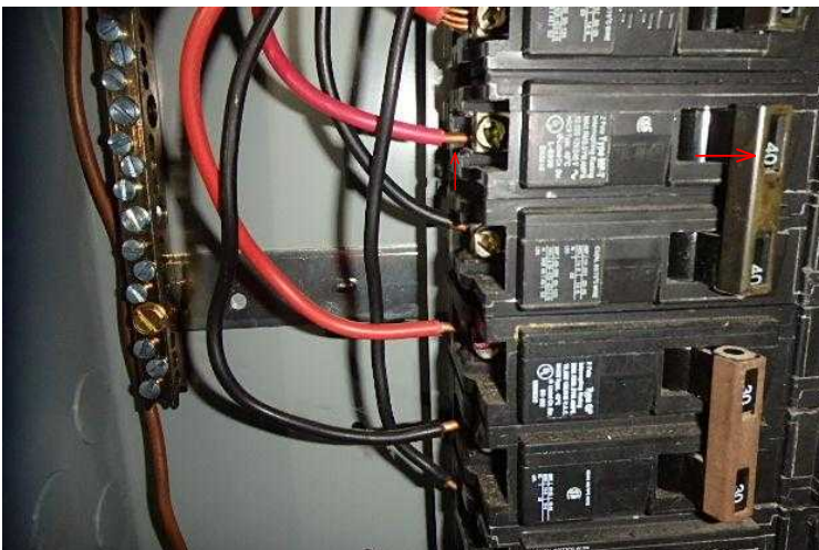
#67 Breaker should be 30 amp.
