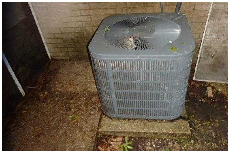
#28 A/C condensing unit.
