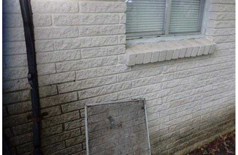
#30 Window screen not installed.
