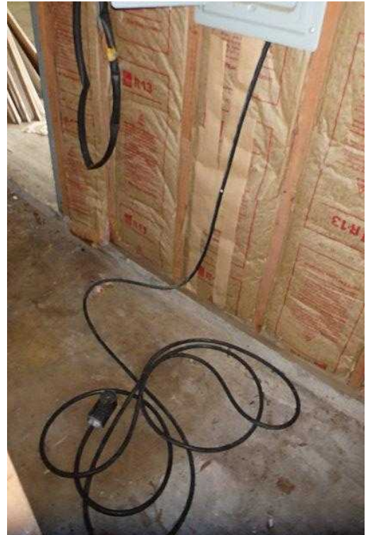
#60 Extension cord hanging out of the electrical panel.
