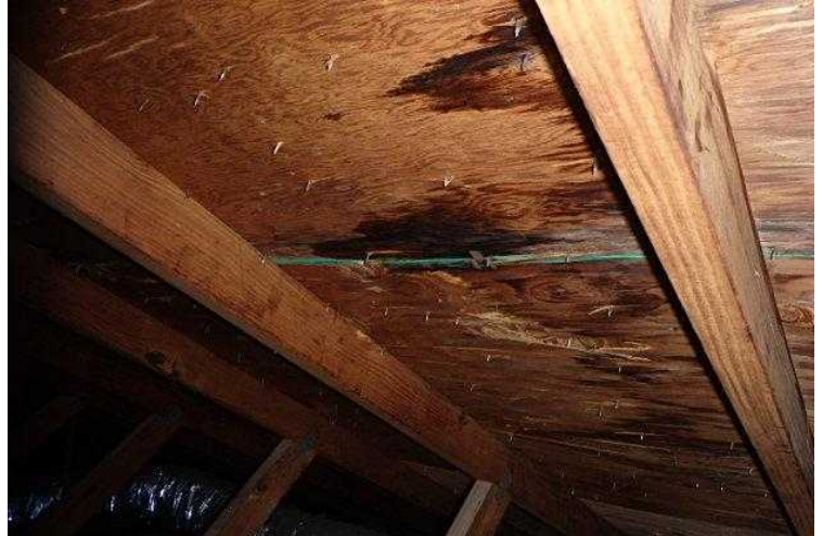
#114 Moisture stains present. These may be old.
