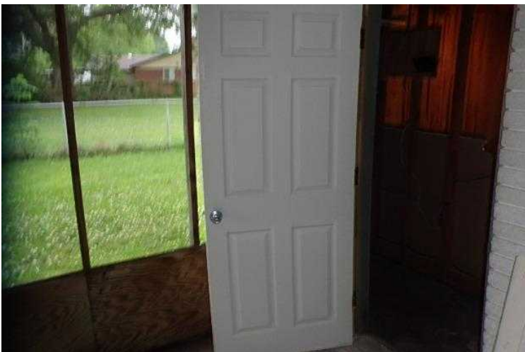
#27 Door to the utility room should be metal clad or solid wood.
