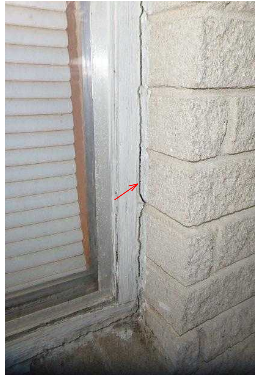
#34 Wood trim around the bathroom window. Open joint indicates some movement.
