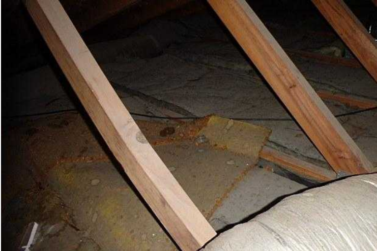
#109 The original insulation was improperly installed with the paper side facing up.
