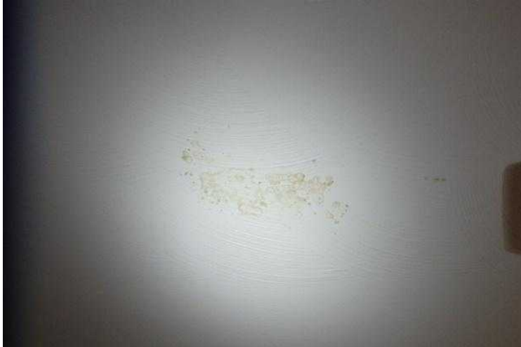
#89 Stain on the ceiling.
