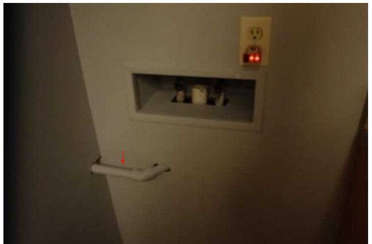
#72 Washing machine service in the kitchen? A/C drain line routed to this drain also.
