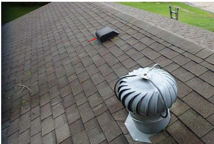
#47 Turbine and open vent. A vent pipe for the kitchen can be installed and routed to the open vent.
