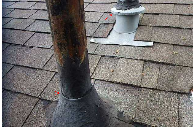
#46 No "rain shield" was installed on the water heater flue.
