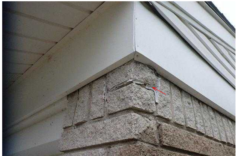
#12 Loose bricks in the upper right corner. Brick veneer is non-structural.
