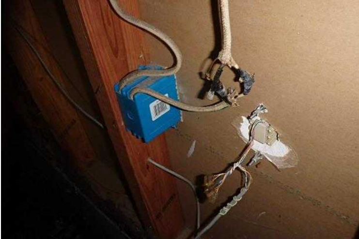
#57 Wire splices should be in junction boxes.
