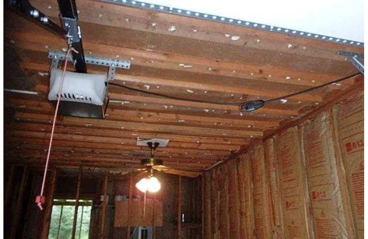
#58 Garage door is plugged into an extension cord. The garage door opener turns off when the light switch is turned "off".
