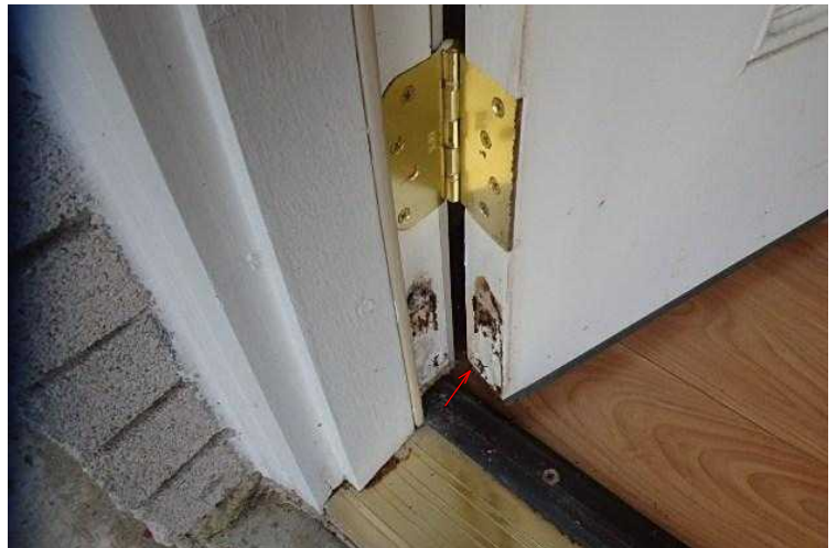
#4 Some soft wood on the backside of the door.
