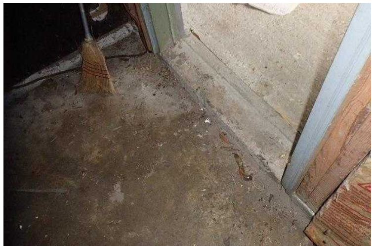
#68 No threshold installed at the patio door.
