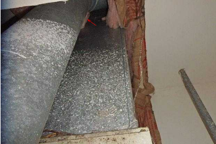
#85 The insulation needs to be moved away from the flue.
