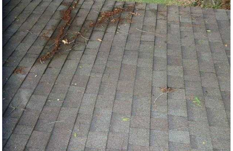
#42 No damage to the shingles from fallen branch.
