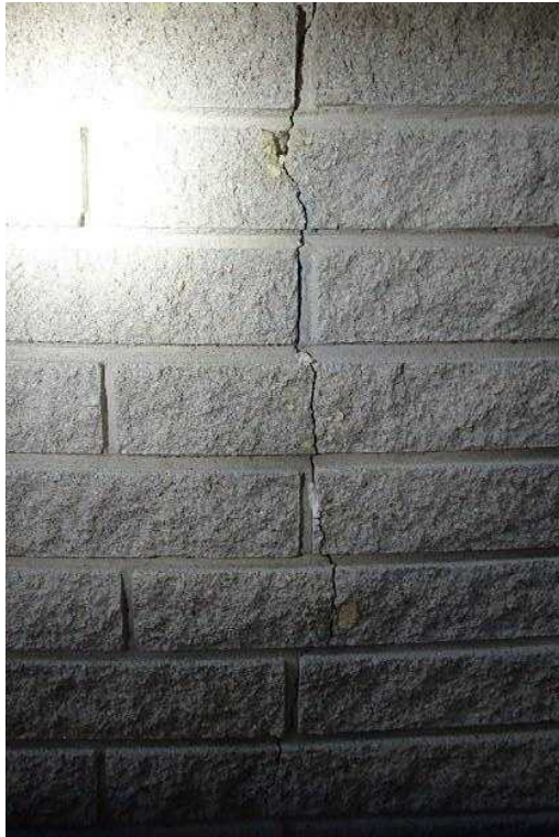
#33 Crack in the rear brick.
