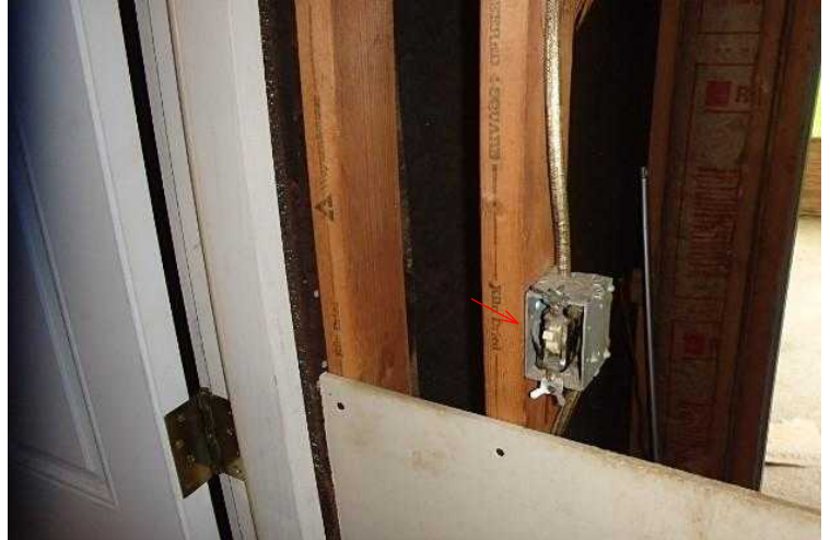
#54 The wall switch controls the garage outlets.
