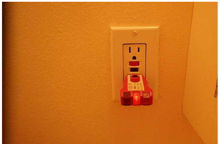
#104 The gfcı receptacle tested as non-grounded.
