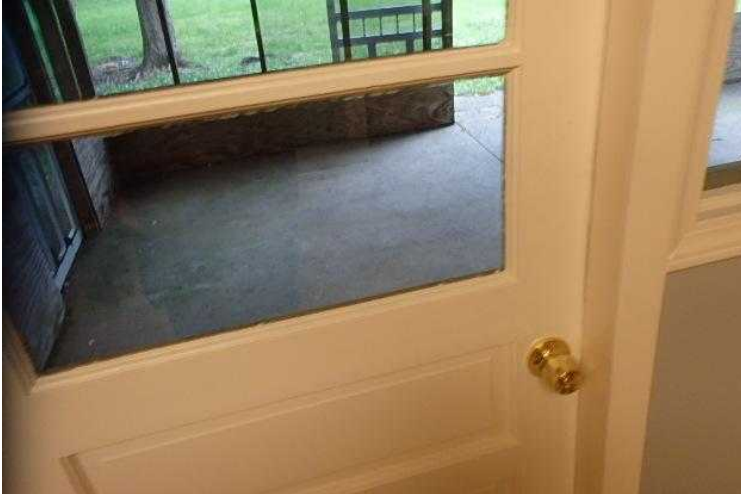
#69 No dead bolt on the kitchen patio door. Single pane glass.
