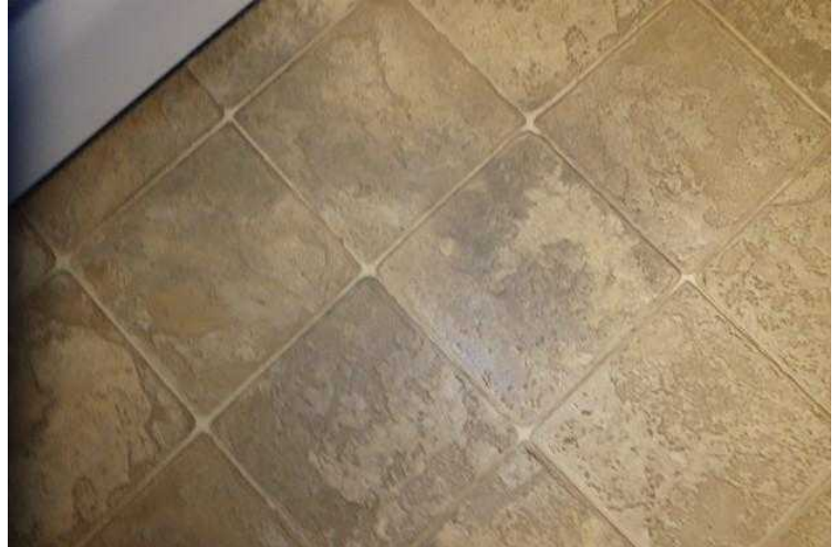
#90 Stains on the flooring in the kitchen.
