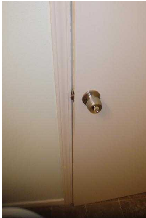
#99 The bathroom door rubs the door frame when closed.
