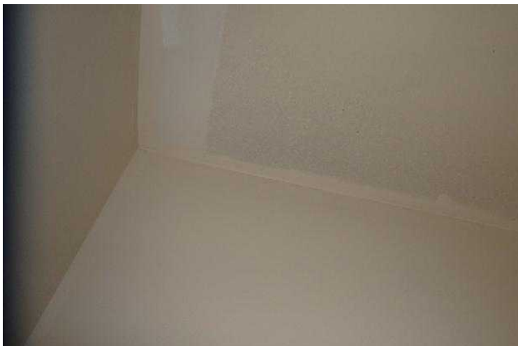
#91 Den closet ceiling not painted.
