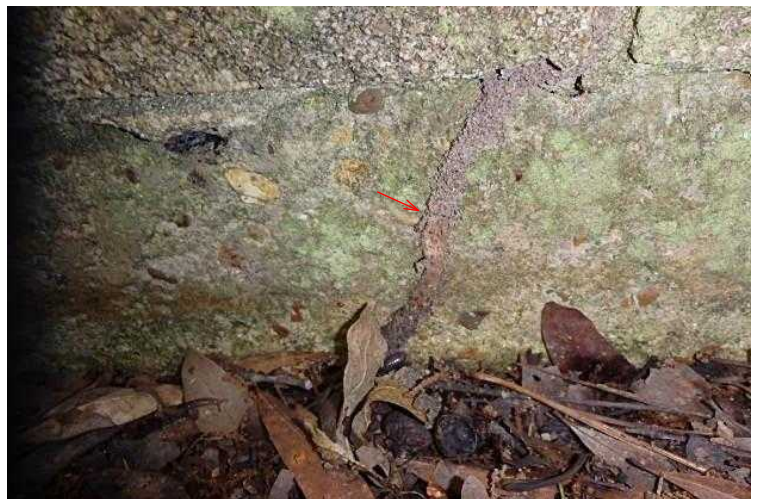
#32 Termite tube in the rear. Active termites were present.
