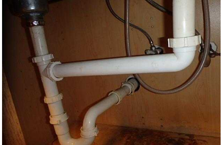
#74 PVC drain pipe attach to galvanized drain piping in the walls.
