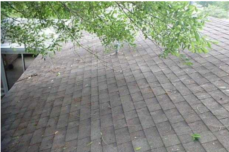
#43 Rear roof. Cut back tree branches soon before damage results.
