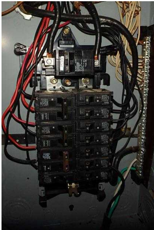
#63 Panel breakers and wiring.
