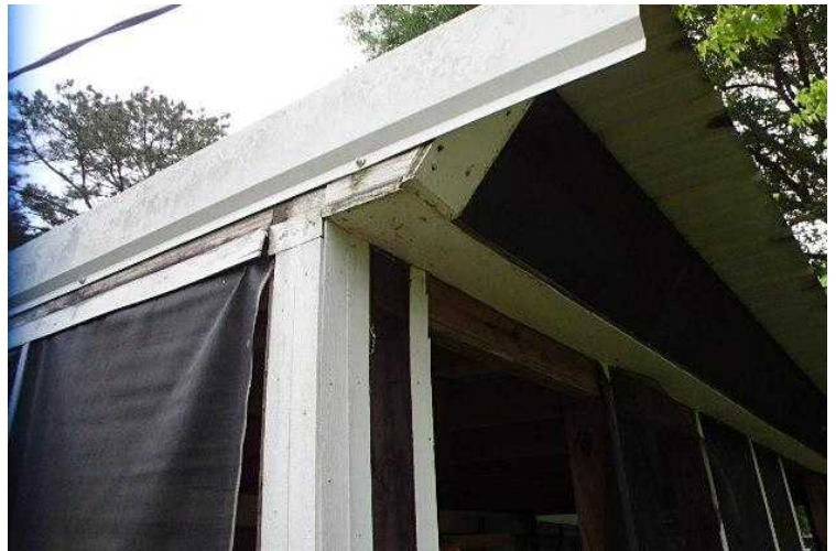
#24 Exposed wood around the top. Keep painted.
