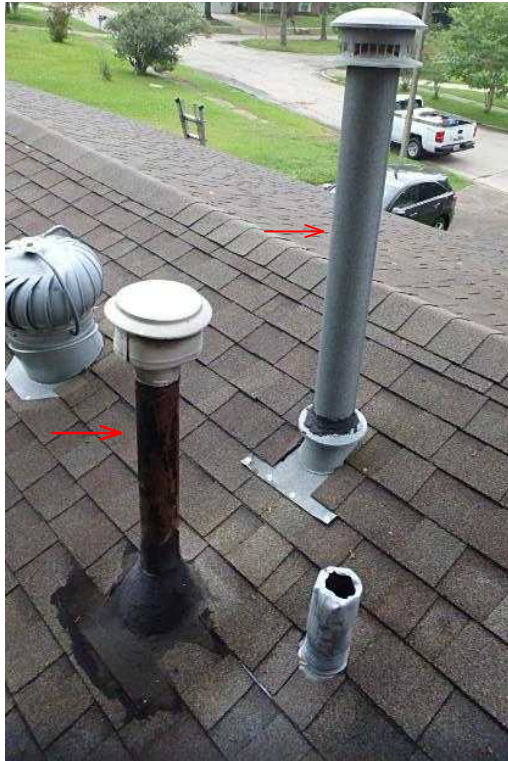
#45 Water heater and furnace flues. The properly terminate on the outside of the roof.
