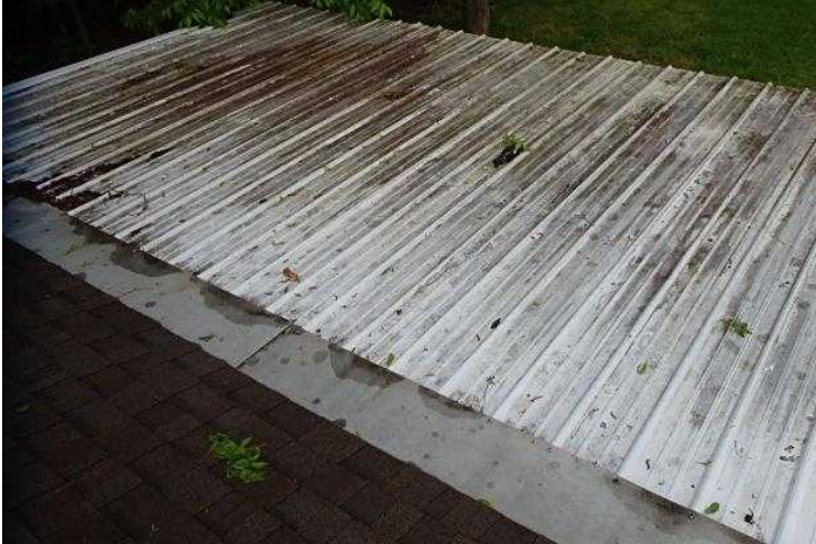
#49 Patio metal roofing. Some rusting present.
