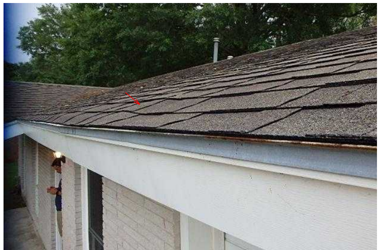
#36 Hump in the roof on the right front. Appears to be from different rafter heights.
