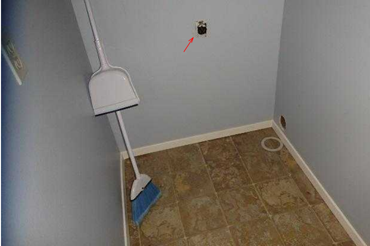
#61 Electric dryer service present in room off the kitchen.
