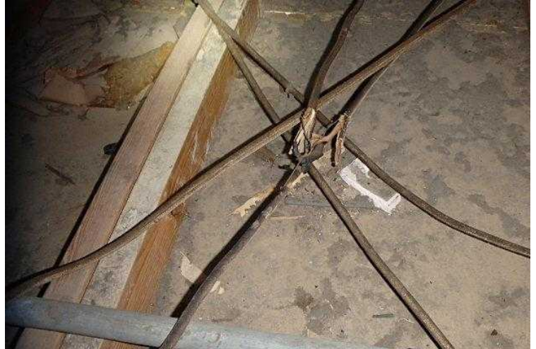
#110 Open wire splices should be in junction boxes.
