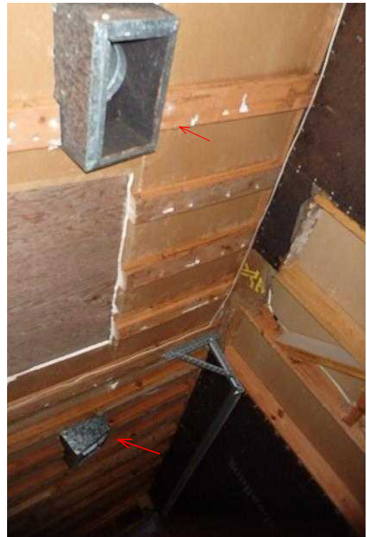
#56 A/C ducts were added to the garage.
