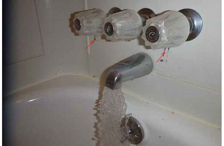
#98 Water was dripping from the faucets when operated.
