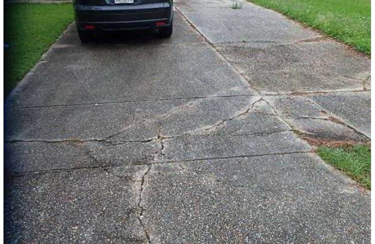
#2 Concrete driveway. Cracking and some settlement present.
