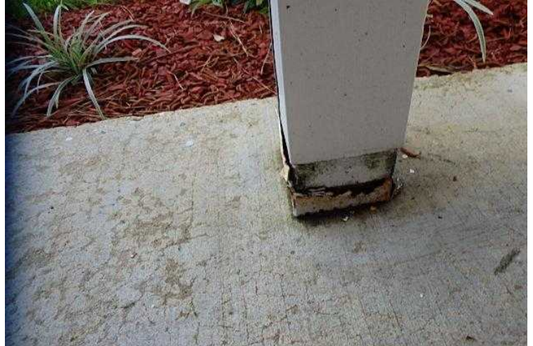
#6 Metal covering rusting along the bottom of the column.
