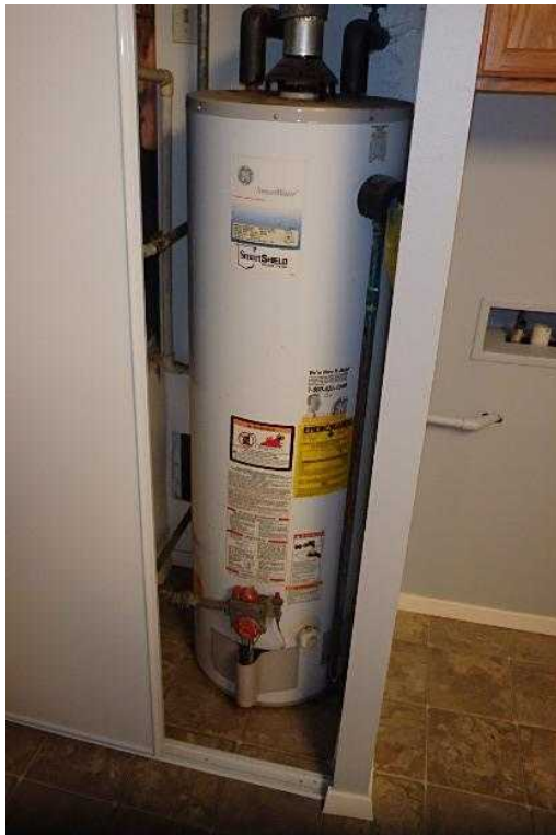
#77 No safety pan under the water heater. Pilot was not lit.
