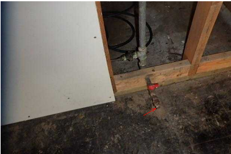
#59 Gas service present. Cap off valve when not in use.
