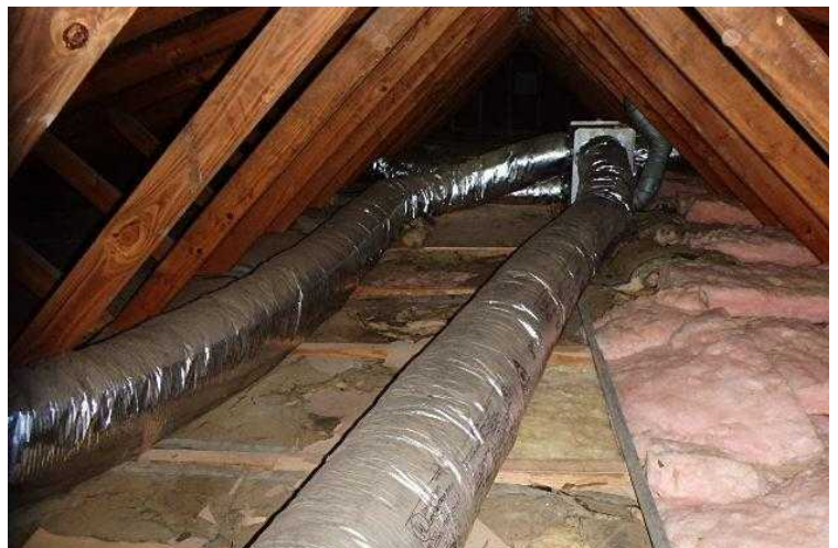
#112 Flex ducts and plenum. Middle attic.
