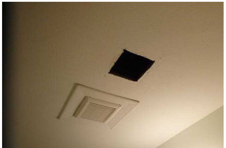
#96 Ceiling register missing.
