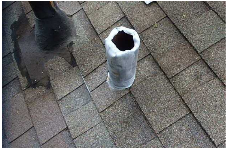
#44 Cast iron and galvanized vent pipes with lead vent flashings.
