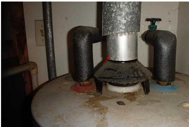
#79 Single wall pipe installed below the flue.
