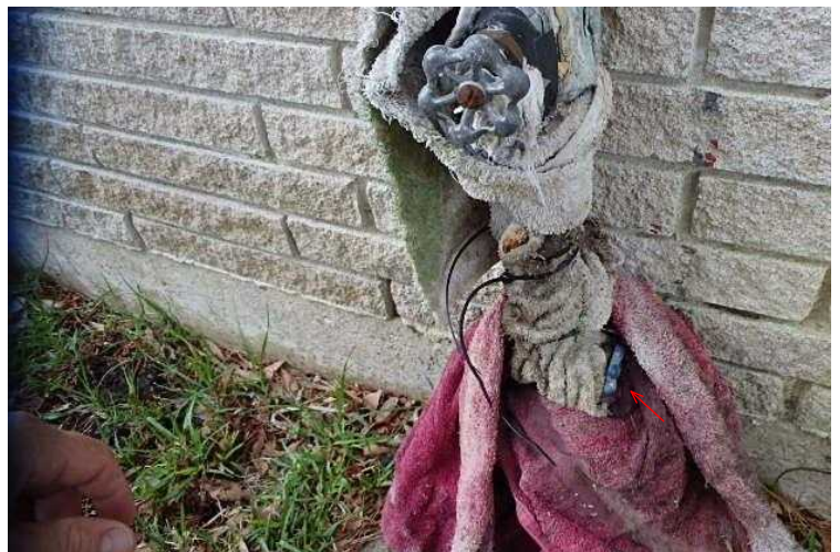
#8 Main water shut off valve on the front left.
