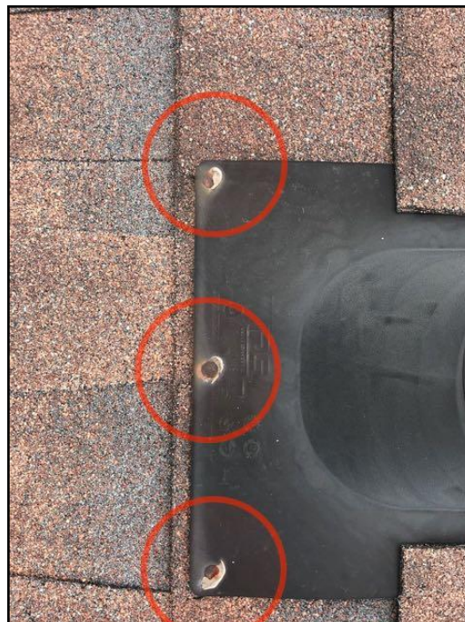
9. Exposed, missing fasteners
