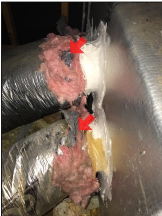
74. Damaged insulation on ductwork
