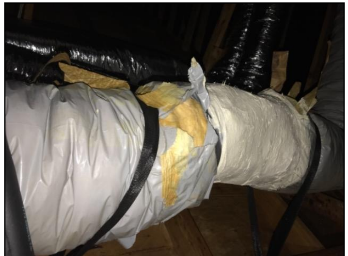
75. Damaged insulation on ductwork
