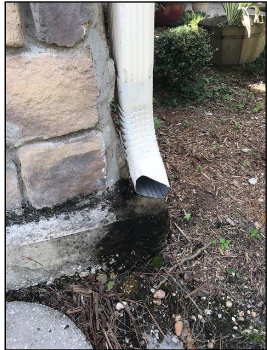
18. Downspouts discharge too close to building
