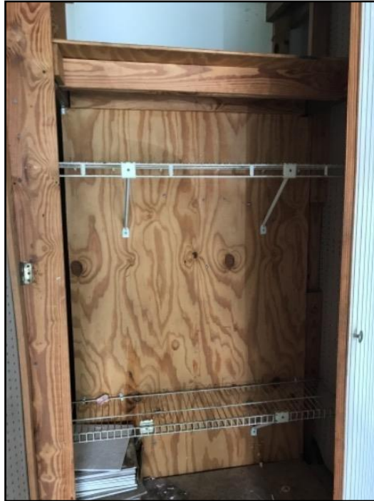
81. Water heater installed behind here
