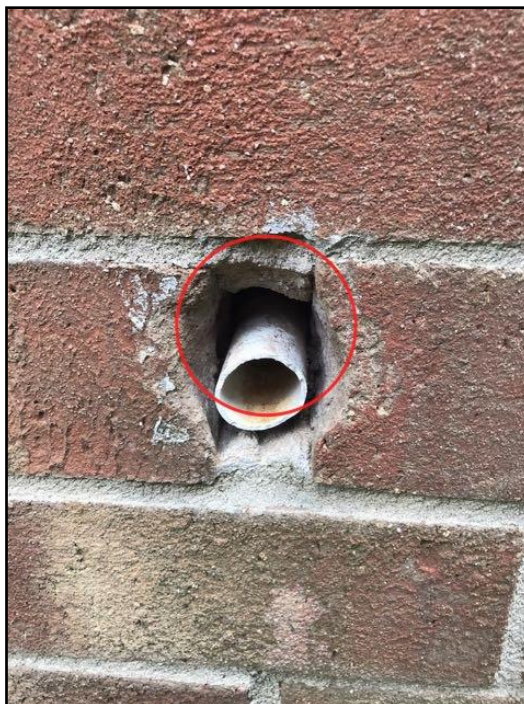
21. Openings observed which may result in pest...
