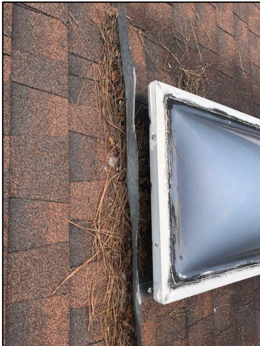
6. Debris build-up at the roof surface may...
