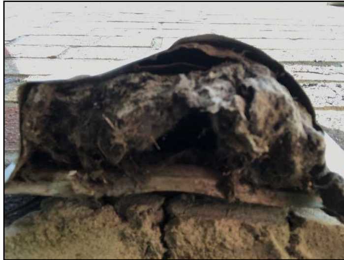
126. Dryer vent obstructed
