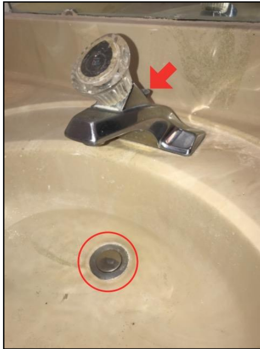
88. Drain stop ineffective
