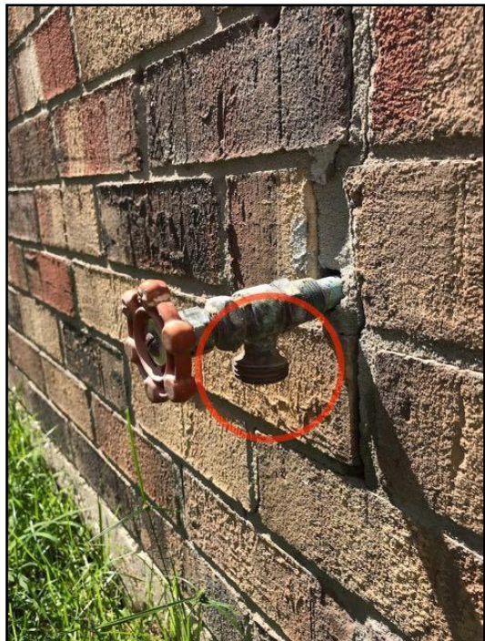
86. Backflow prevention missing
