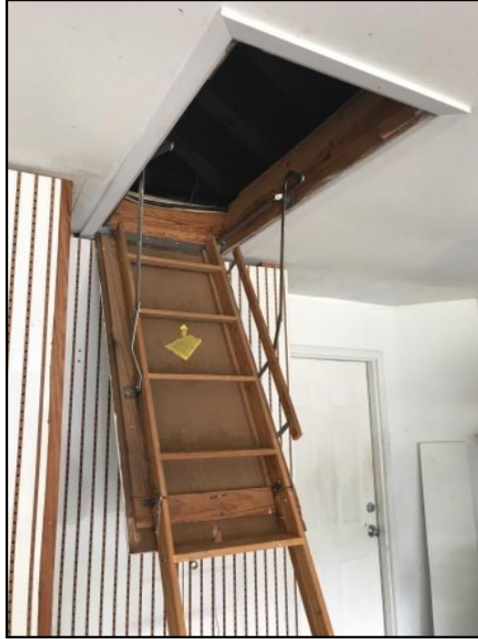
120. Fire separation between garage and attic no...
