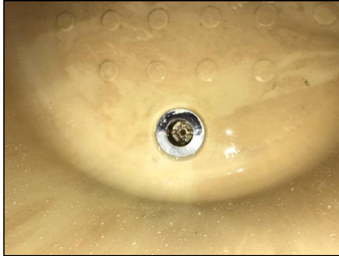
90. Drain stop missing
