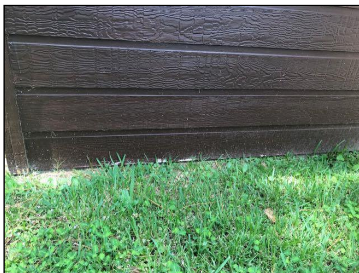
22. Too close to grade
