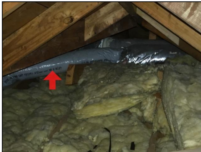
72. Gray vinyl ductwork
