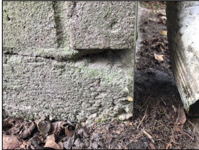
37. Typical corner cracks noted at slab
