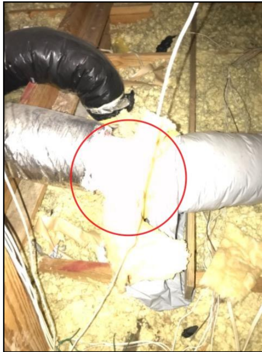
76. Damaged insulation on ductwork
