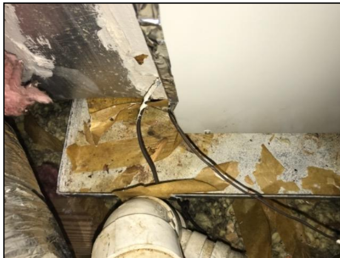
65. Overflow drain pan needs cleaning. Recommen...
