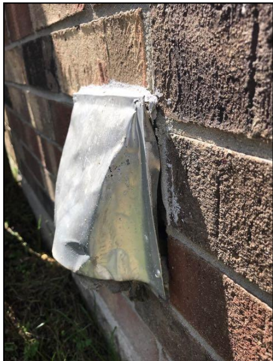
19. Recommend caulking/sealing the intersection...
