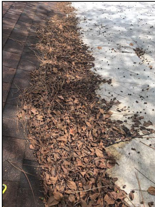
2. Debris build-up restricts fully viewing of...
