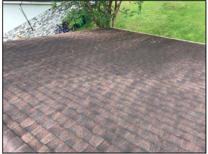
5. Discoloration/algae observed at the roofing...
