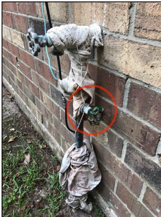
80. Main water valve
