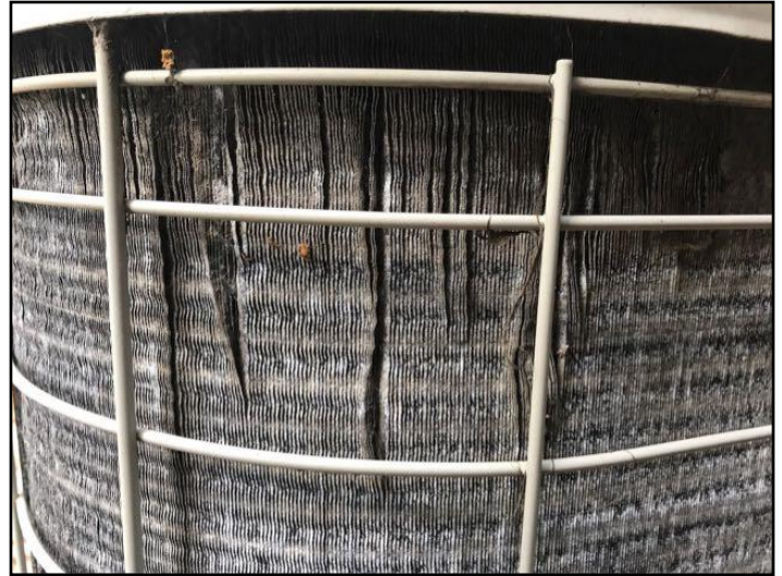
71. Damaged fins on condenser
