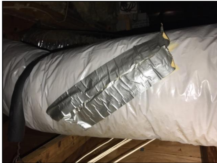
73. Duct tape used on the HVAC system. This is...
