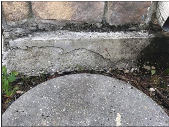
38. Spalling, crumbling or broken material
