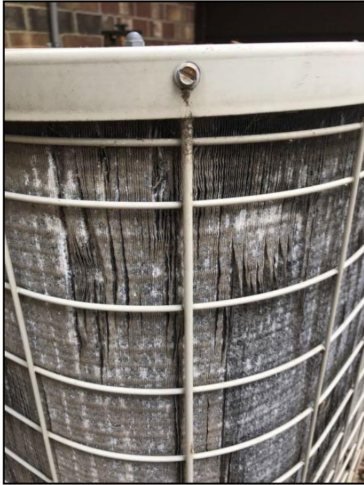
70. Damaged fins on condenser
