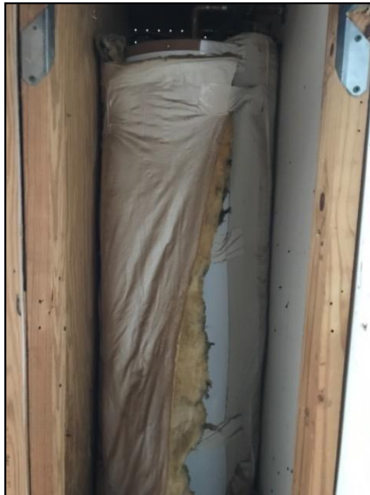
82. Water heater is covered by an insulated...
