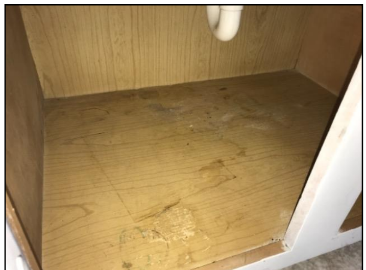
115. Stained, worn, damaged
