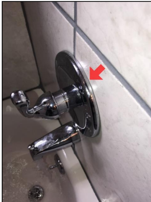
89. Recommend sealing around fixtures to preven...
