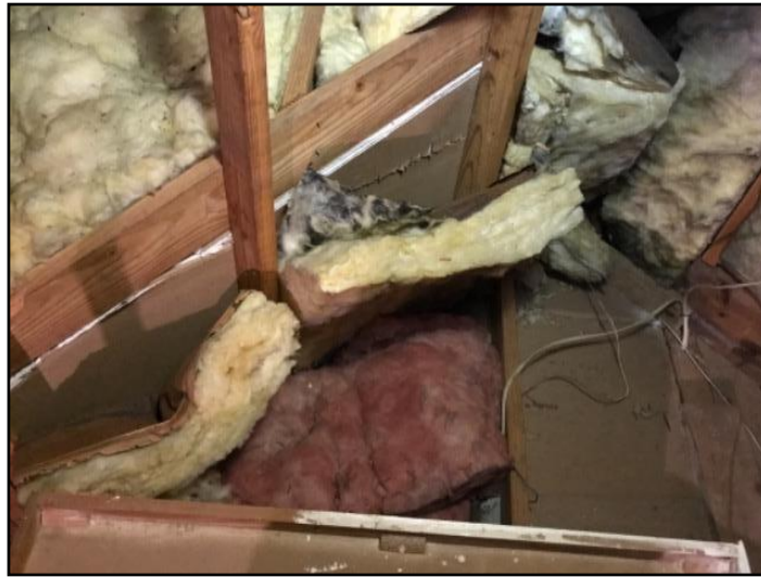
77. Worn and/or falling insulation noted at..
