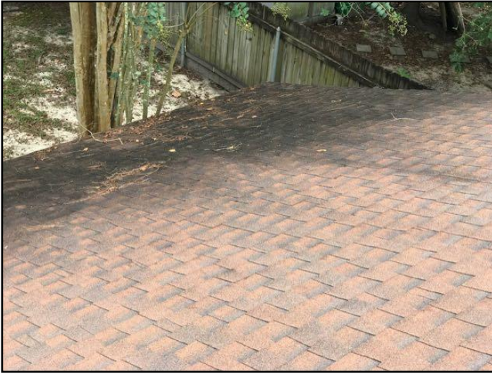
4. Discoloration/algae observed at the roofing...
