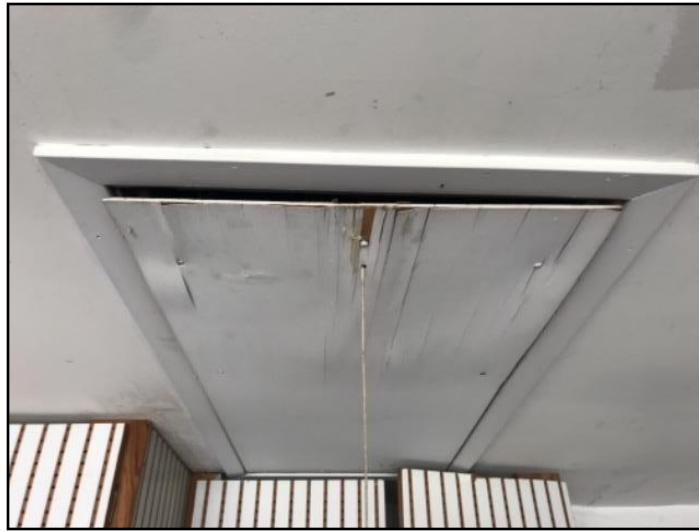
79. Attic access does not fully close
