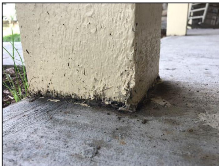
30. Minor damage/deterioration at the base of...
