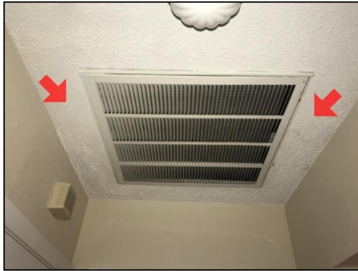
101. Previous repairs noted. Recommend verifying...
