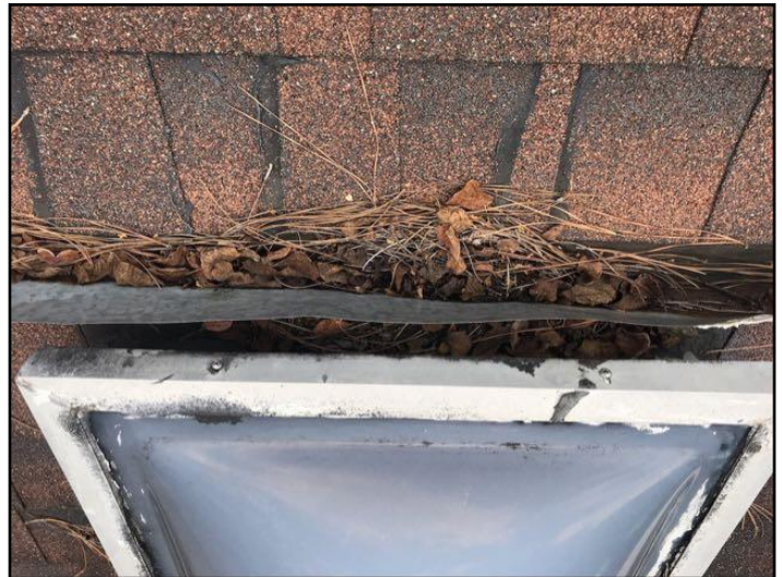
7. Debris build-up at the roof surface may...
