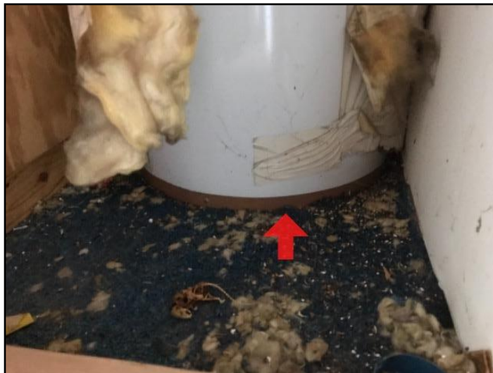
84. Safety pan and drain missing
