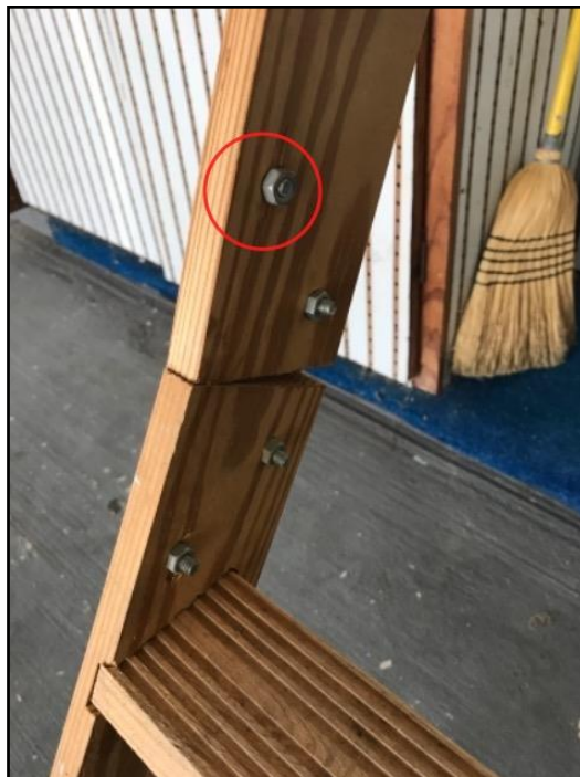
78. Some attic ladder fasteners are unsecured....
