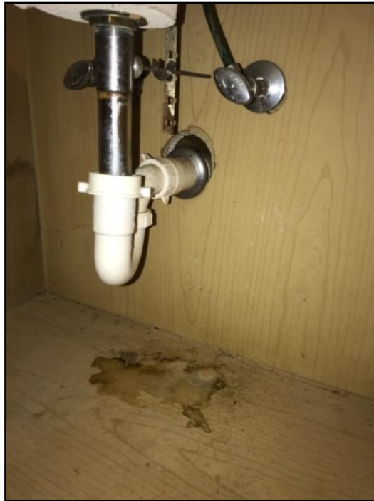
116. Stained, worn, damaged
