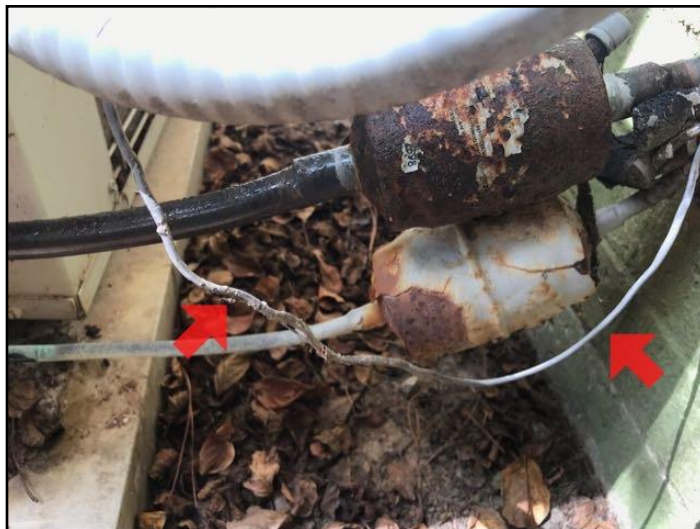
63. Recommend properly protecting control wires.
