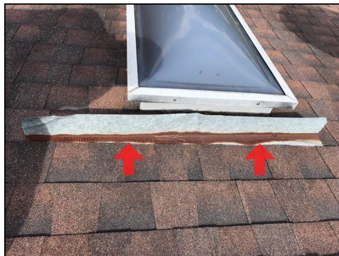
8. Rusty flashing observed at the roof surface.
