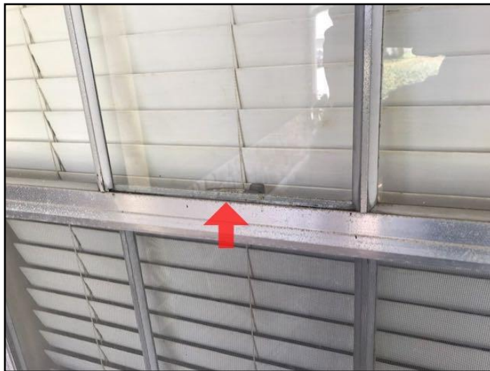
29. Missing or loose pieces
