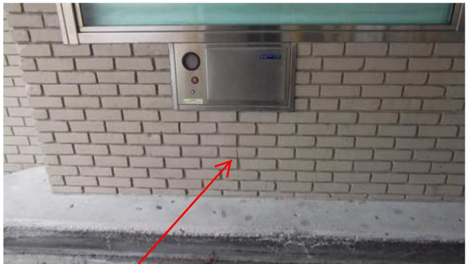
Crack in brick veneer.
