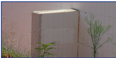
A “Dead-Man” centered on a 30' retaining wall formed as a T-wall intersection.
