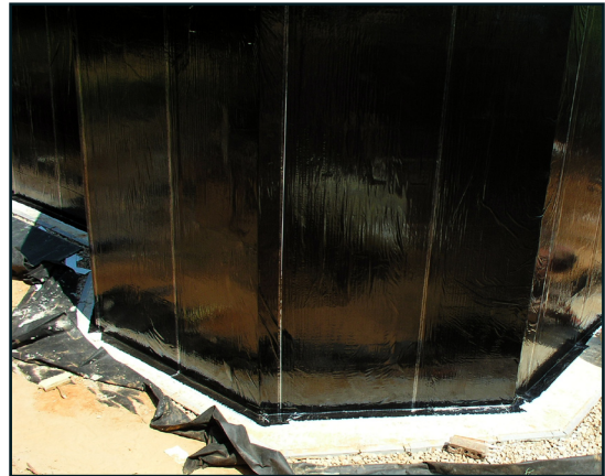
This method insures no penetration through the block below grade and is a tried and true method but is time-consuming to install.
