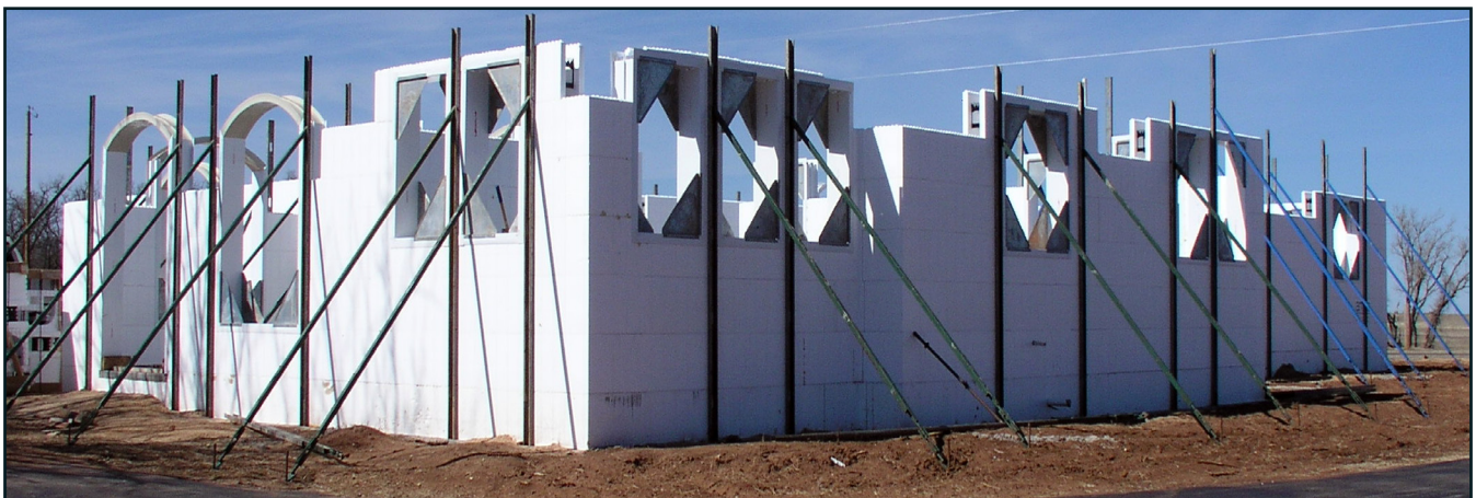
For larger openings than 3' wide, additional bracing and "bracing legs" (long 2x4 wood legs screwed to the vertical bucks and run to a base plate will help keep your openings straight and plumb during the pour.
