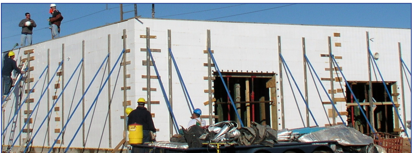
Ample Outer Bracing with “Scabs” on Non-Factory or Irregular Cut Joints (No Walk Boards)
