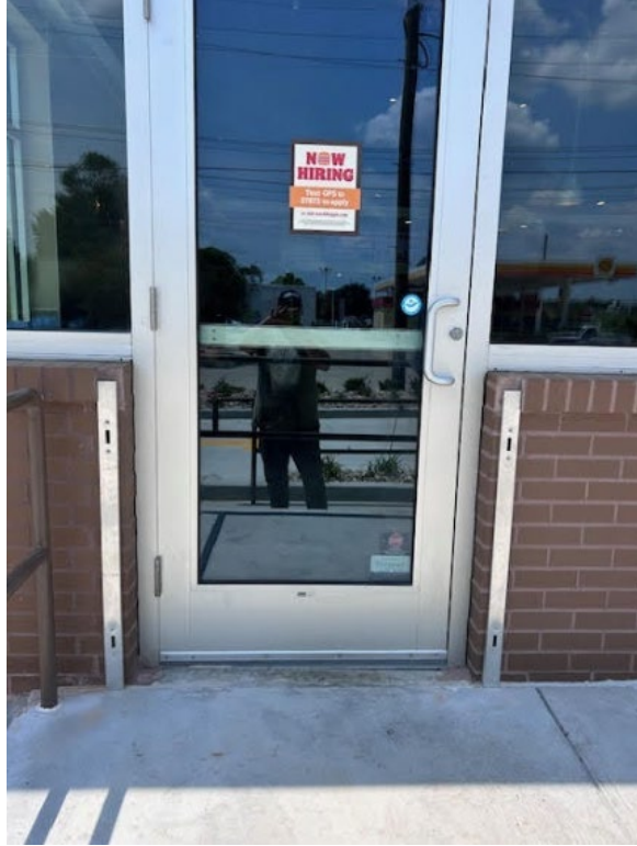
Door 2 Front Entry without Flood Barrier August 09/2024
