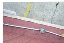
Canopy - No Cover on Junction
