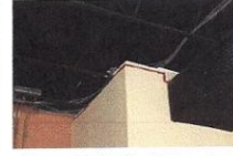
Upper Walls @ Air Handler
