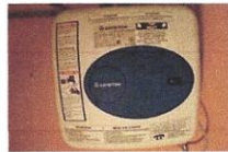
Bath - Water Heater
