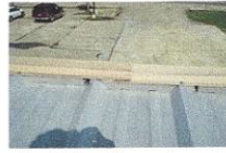
Front Edge Closure Incomplete
