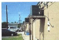
Rear - Condenser Unit & Platform
