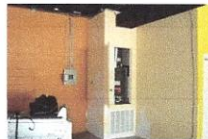
Air Handling Unit
