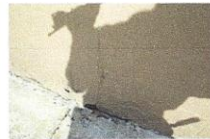
Wall - Possible Moisture Penetration
