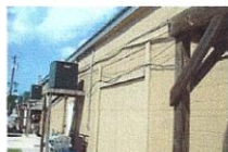
Rear Wall - AC Unit
