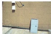
Rear Wall - Electrical Panel
