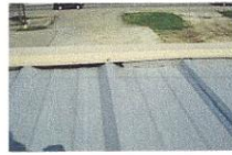
f - Front Edge Closure Incomplete
