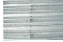
Roofing Lap - Beginning Deterioration
