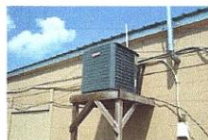
Rear Wall - AC Unit & Platform
