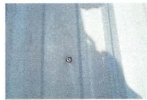
Roof - Fastener Rust
