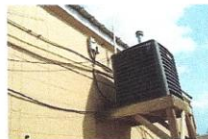
Rear - Condenser Unit & Platform
