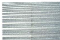
Roofing Lap - Beginning Deterioration
