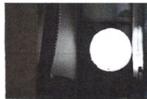
Air Handler - Enclosure
