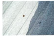
Roof - Fastener Rust (2)
