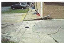
Left Rear Corner - Pipe (2)
