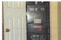
Air Handling Unit Closeup
