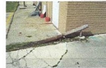
Left Rear Corner - Pipe
