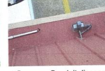
Front Canopy - Conduit disconnect
