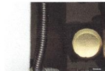
Air Handler Enclosure
