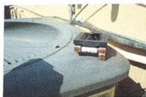
Rear - Condenser Unit Pullout
