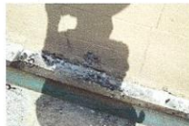
Wall - Possible Moisture Penetration
