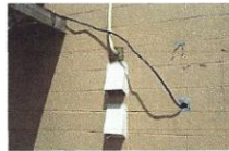
Rear Wall - Wiring Alteration
