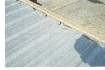
Front Edge Closure Incomplete
