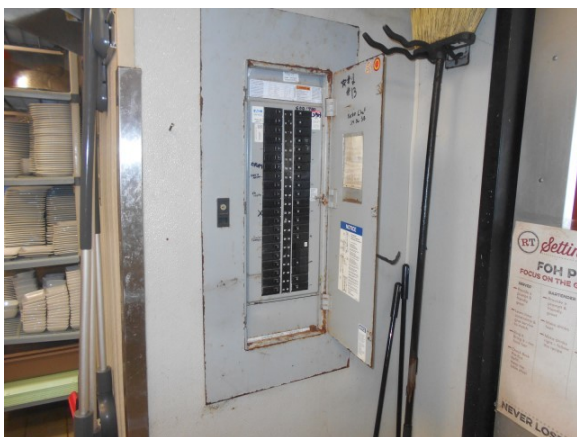
35. Electric circuit breakers
