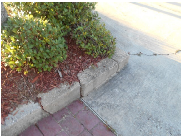
29. Cracked curbing and concrete
