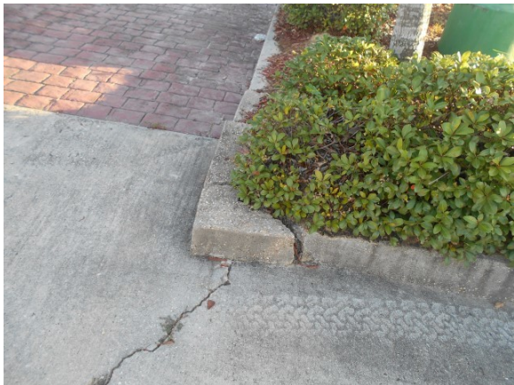
27. Cracked curbing and concrete
