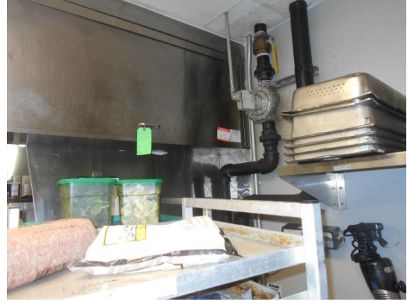
32. Fire suppression under the hood
