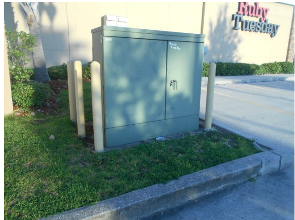
16. Pad mounted transformer
