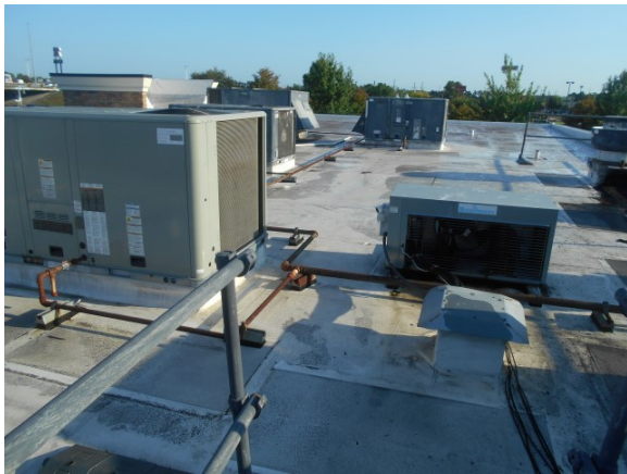
51. Rooftop gas-fired packaged HVAC units
