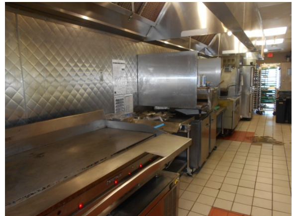
34. Fire suppression under the hood
