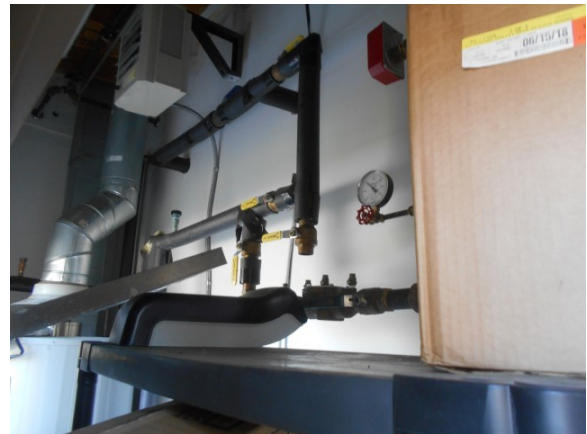
46. Black iron gas piping
