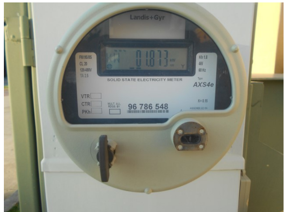
18. Electric service meter
