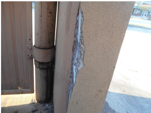
23. Damaged to compactor enclosure
