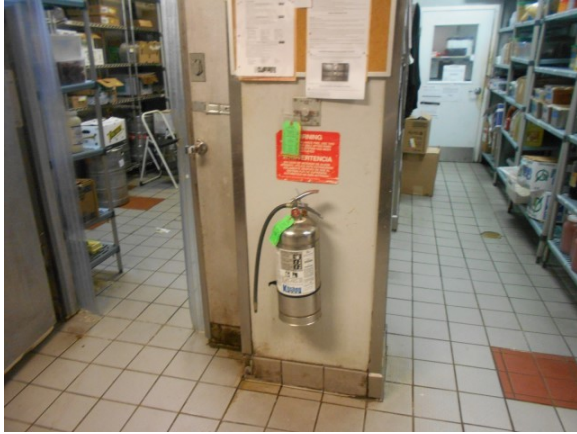
37. ANSUL system and chemical fire suppression
