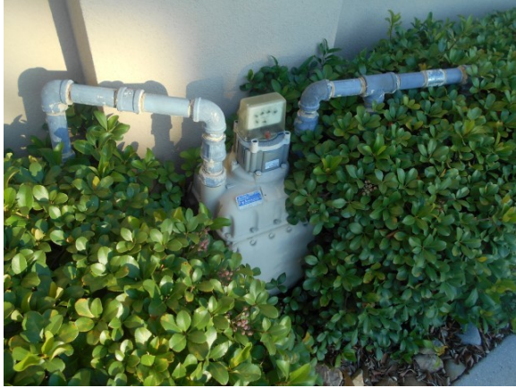
19. Natural gas service meter
