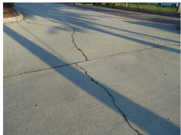
30. Cracked concrete paving
