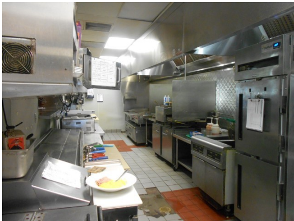
33. Missing floor tiles in kitchen
