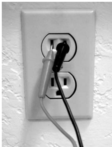
Figure 13-1 Checking power supply through receptacle with a test light
