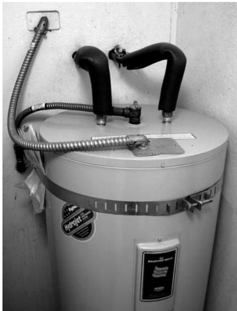
Figure 11-8 Top of water heater showing electrical connections
