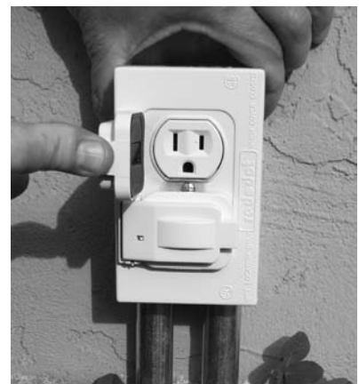
Figure 6-15 Weatherproof box supported by conduits on the wall
