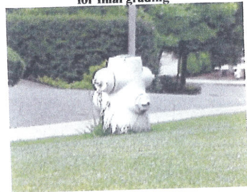
Hydrant set too high for final grading
