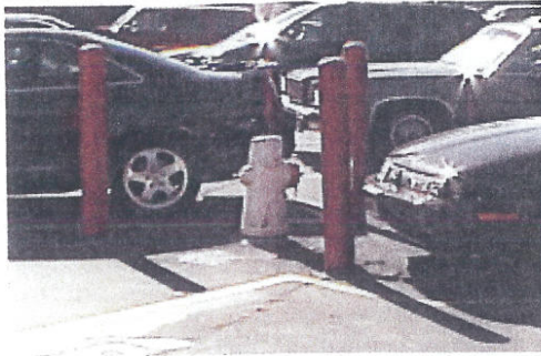
Pumper outlet facing into tree, hose outlet into parking space.
