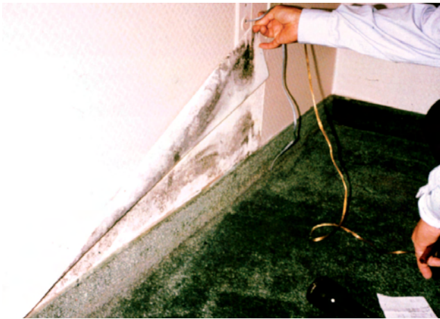
Photograph 8: Hotel Mold —Vinyl wall coverings are low perm materials that retard inward vapor movement and lead to mold growth.
