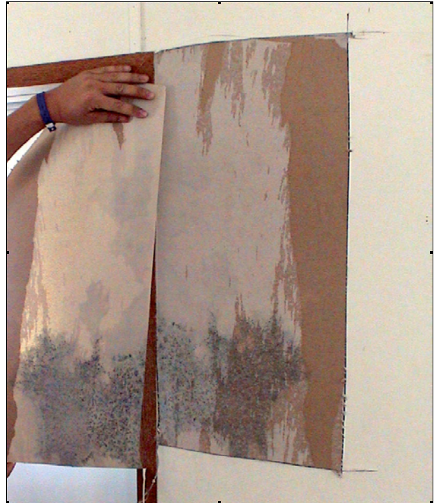
Photograph 6: Vinyl Covered Gypsum Board —FEMA trailers are lined with vinyl-covered gypsum board as are HUD manufactured houses. This leads to mold problems. The only solution is to not install vinyl covered gypsum board.
