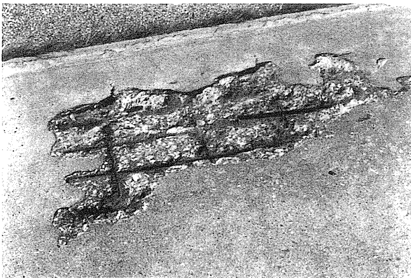
FIGURE 3.2.2.5(2). Delamination of Concrete Caused by Corrosion of Reinforcing Steel
