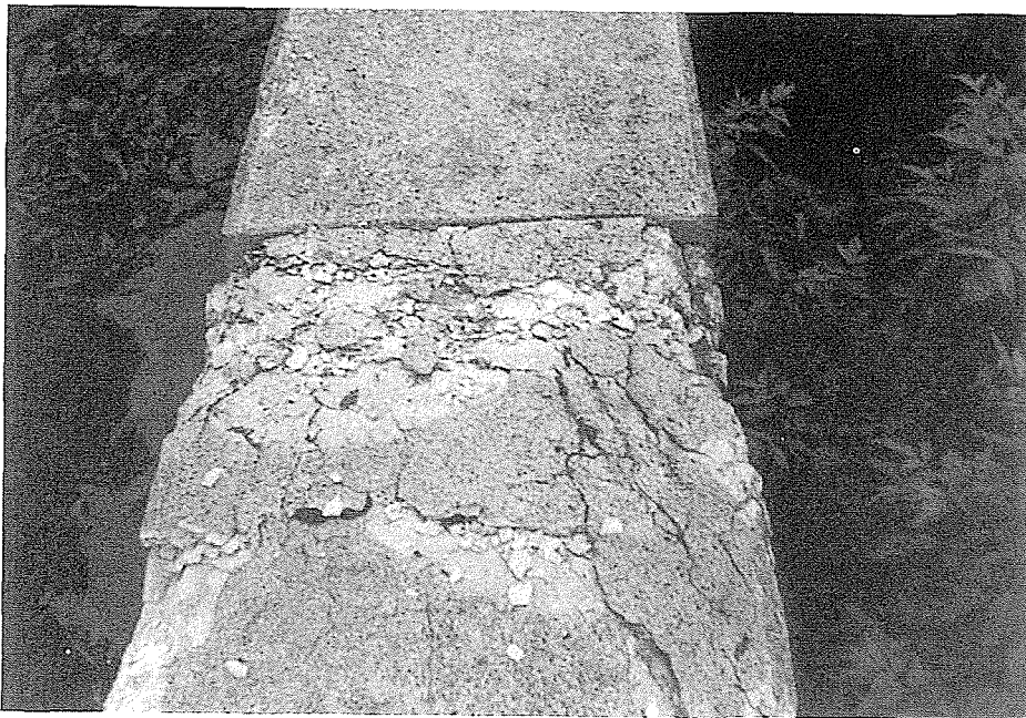
FIGURE 3.2.2.5(4). Freeze Thaw Damage to Concrete Wall
