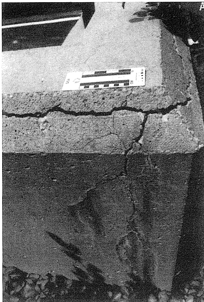
FIGURE 3.2.2.5(3). Cracking of Concrete Due to Alkali-Silica Reaction and Efflorescence on the Face of the Wall
