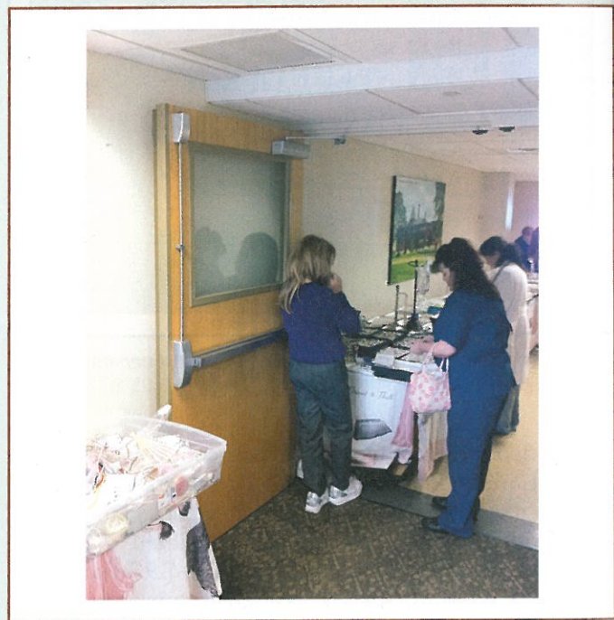
Exhibit 18/19.94 Smoke barrier door left free of obstruction to permit proper closing.
