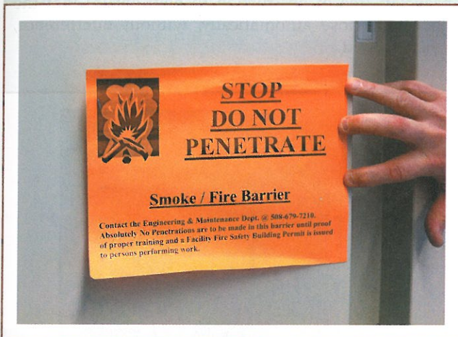
Exhibit 18/19.89 Placard with warning against penetration of smoke barrier.
