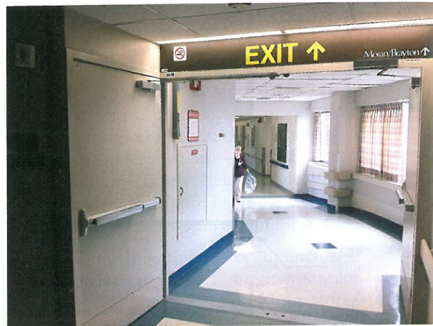
Exhibit 18/19.86 Smoke barrier where penetrations are located above ceiling.
