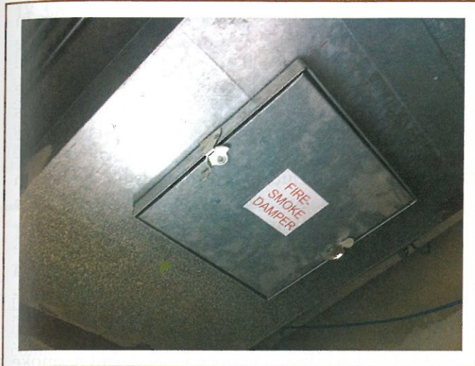
Exhibit 18/19.88 Smoke barrier duct penetration protected by smoke damper.
