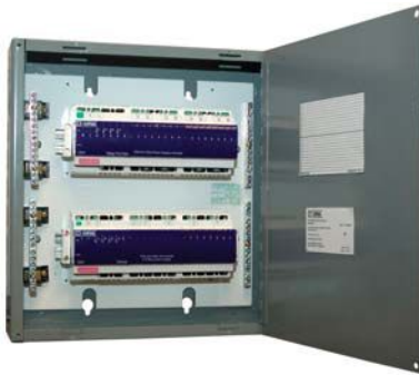
Area Lighting Panel
