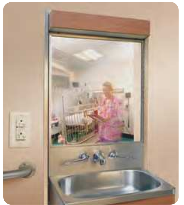
EXHIBIT 517.3 Hospital grade tamper-resistant GFCI in a hospital environment. (Courtesy of Legrand/Pass & Seymour®)
