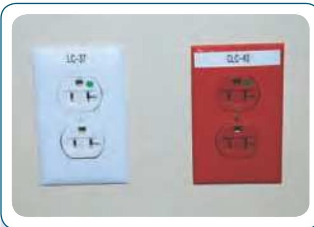
EXHIBIT 517.4 A receptacle from the normal system (left) and the emergency system (right). Note the label that indicates the panelboard and the circuit number. (Courtesy of the International Association of Electrical Inspectors)
