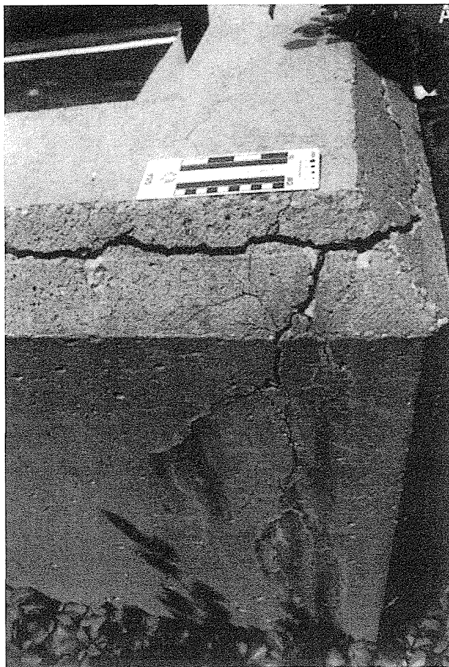
FIGURE 3.2.2.5(3). Cracking of Concrete Due to Alkali-Silica Reaction and Efflorescence on the Face of the Wall
