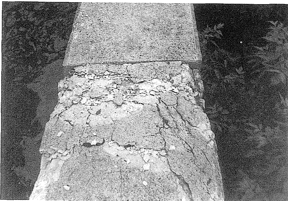
FIGURE 3.2.2.5(4). Freeze Thaw Damage to Concrete Wall
