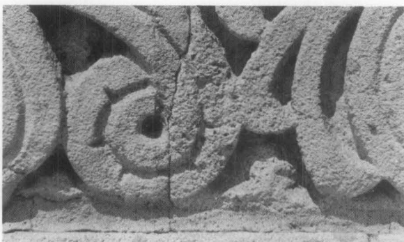
Cracking of limestone. Photograph: John H. Myers.
