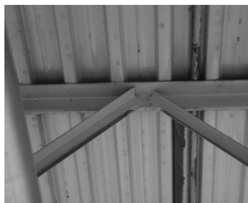
Fig. 5. Angles interfering with top chord reinforcement.
